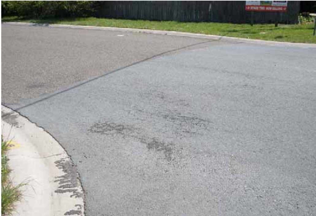
Photo 77 – Start of Maclura Dr. Crocodile cracking.
