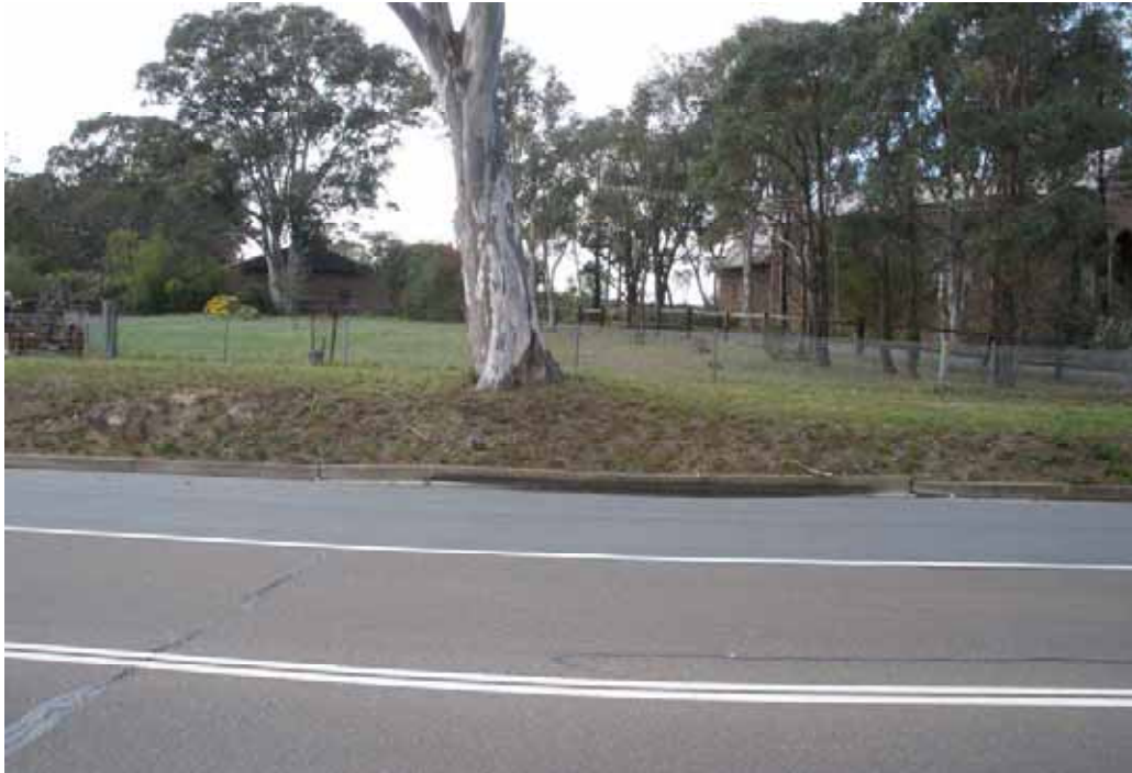
Photo 27 – Opposite church. Gutter failure due to tree roots.
