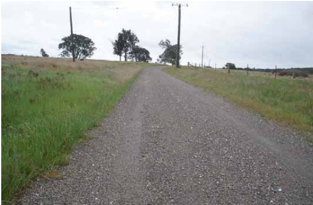
Photo 106 – Stoney Creek Rd (unsealed). Depressioning along southern wheel path.
