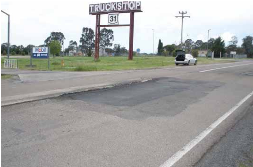
Photo 2 – George St at Truck Stop 31 entrance. Patching from previous failure with deformation still present.
