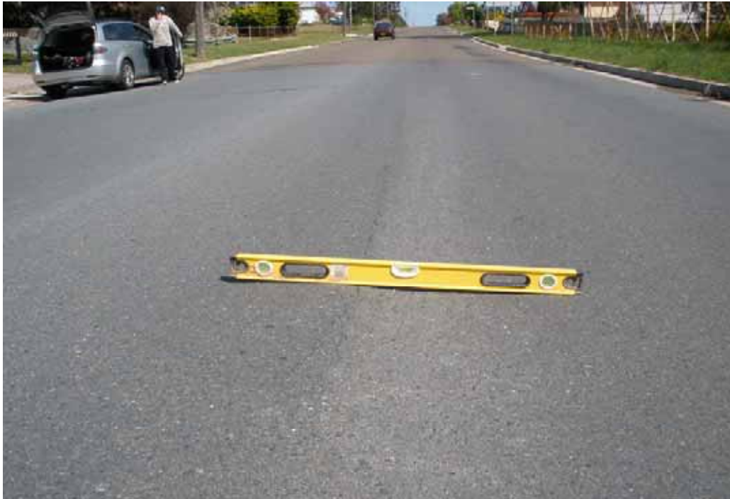
Photo 57 – Brayton Rd, near end of newer pavement. Difference in asphalt height possible rutting with cracking.
