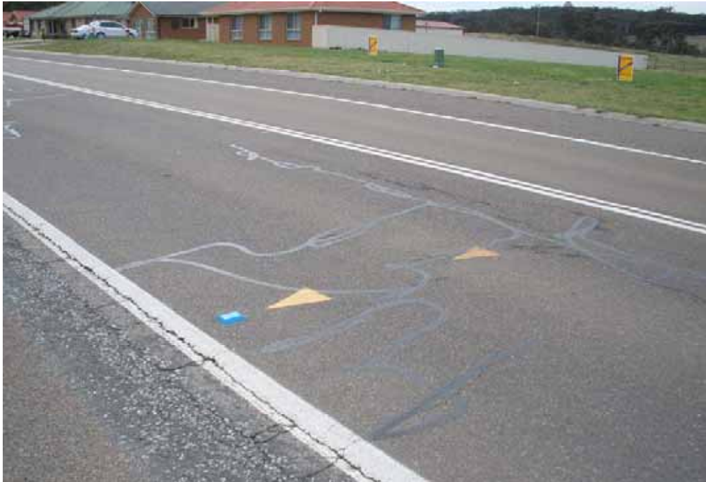
Photo 15 – George Street, opposite vacant blocks. Numerous cracking some sealed with bitumen emulsion.
