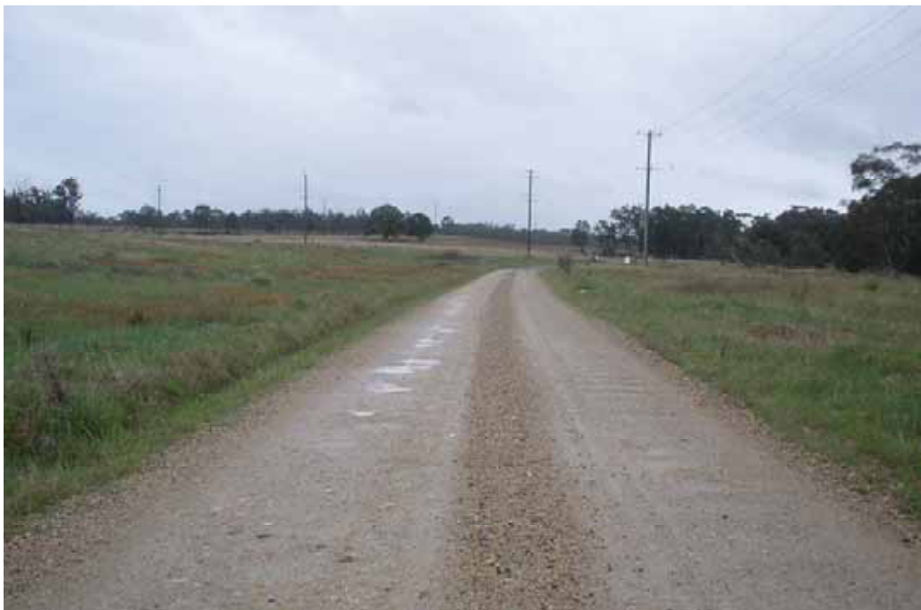
Photo 116 – Stoney Creek Rd (unsealed). Small potholes, uneven surface and corrugations.
