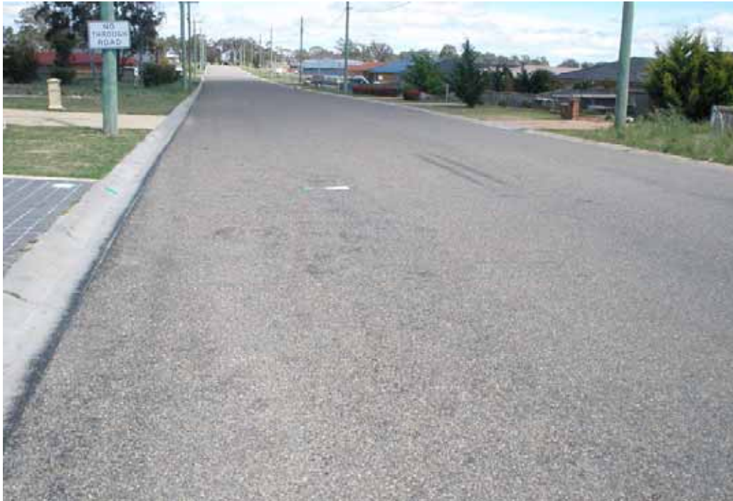
Photo 89 – Near intersection of Brayton Rd & Stoney Creek Rd. Bitumen bleeding.
