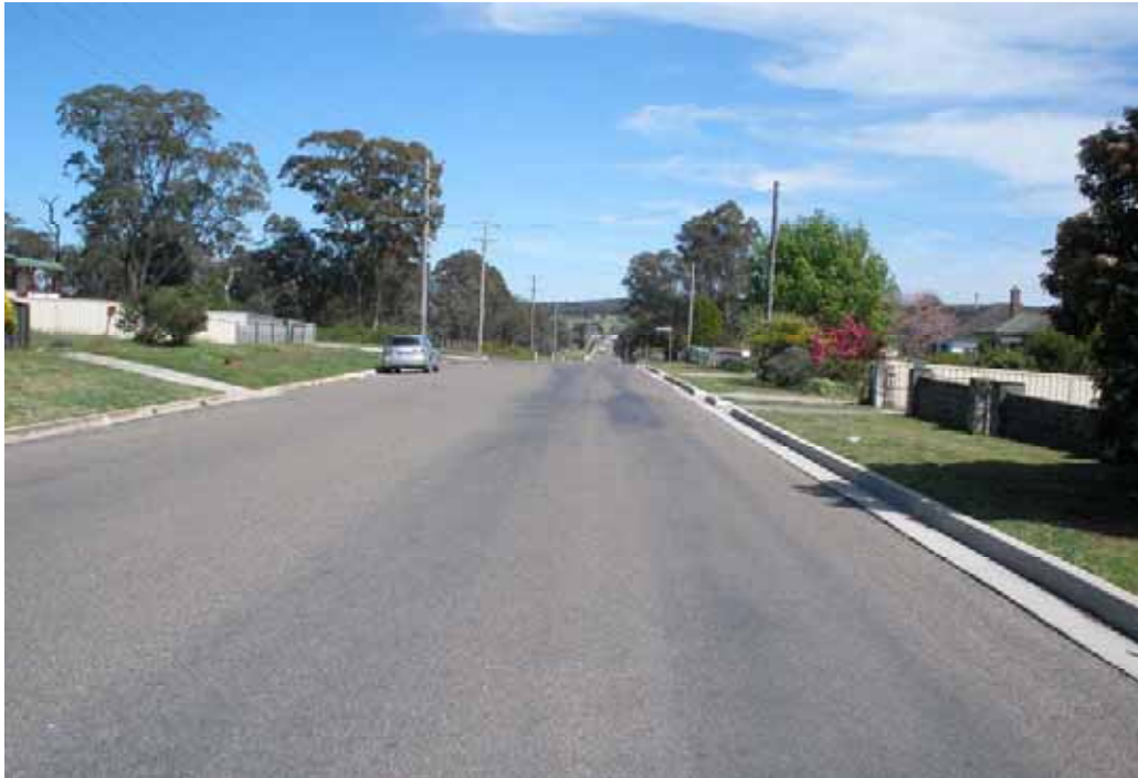
Photo 63 – Opposite No 16 Brayton Rd. Bitumen bleeding (east bound).
