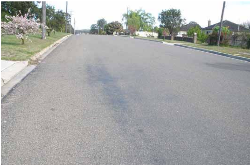
Photo 62 – Opposite No 6 Brayton Rd. Bitumen bleeding and slight rutting.
