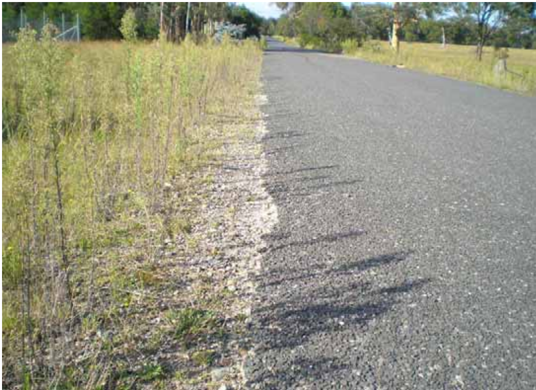
PHOTO 64: Pavement edge failure
