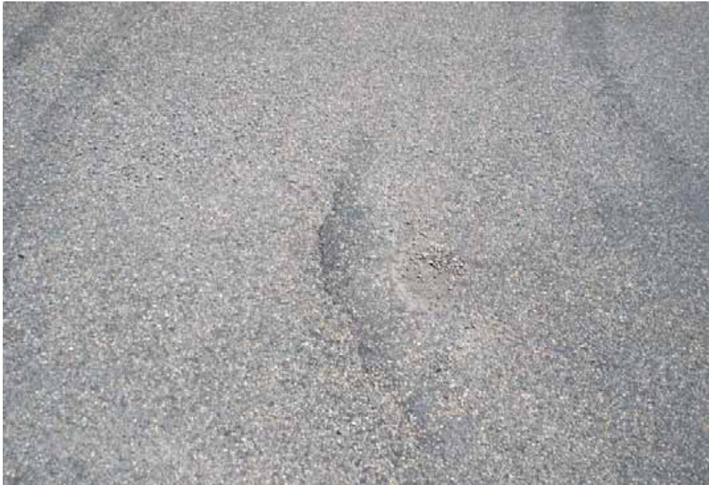
Photo 95 – Intersection of Stoney Creek Rd & Jilba Ave. Bitumen bleeding and shoving.
