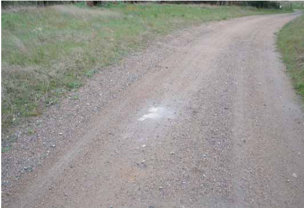
Photo 103 – Stoney Creek Rd (unsealed). Small pothole.
