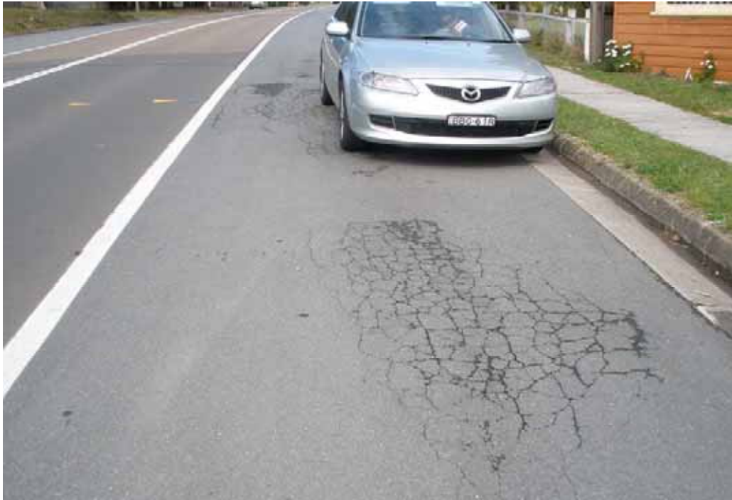
Photo 29 – Opposite No 46 George St. Crocodile cracking in shoulder.
