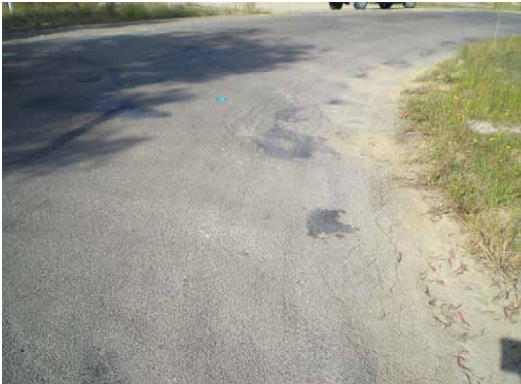
PHOTO 38: Settlement, cracking/rutting in asphalt at pavement edge
