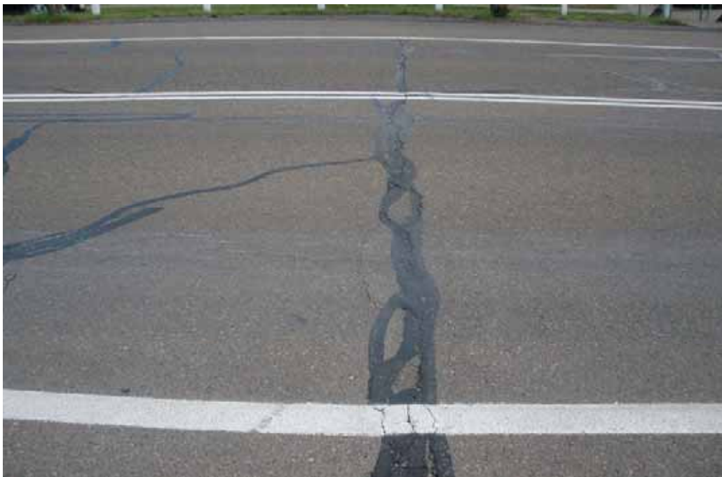
Photo 38 – Opposite post office. Pavement cracking post application of bitumen emulsion. Edges of cracking rising.
