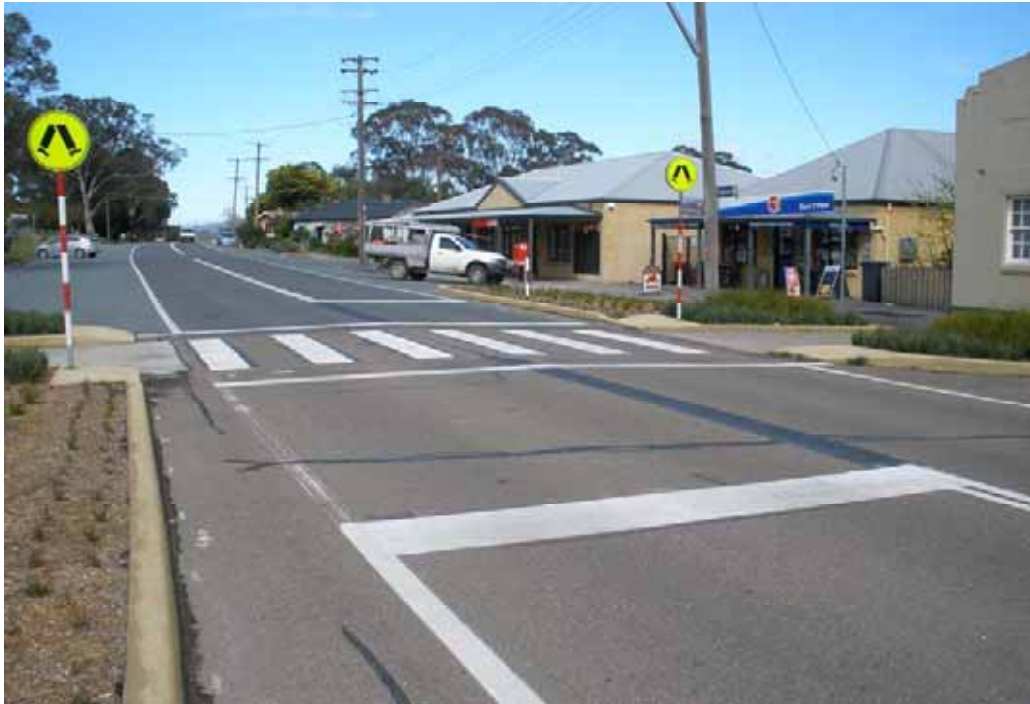
Photo 35 – Opposite pub. Numerous cracking with bitumen emulsion sealing.
