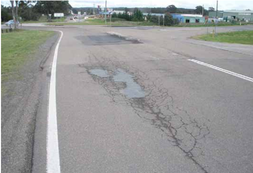
Photo 7 – Opposite entrance to Truck Stop 31. Extensive cracking with some old patching.
