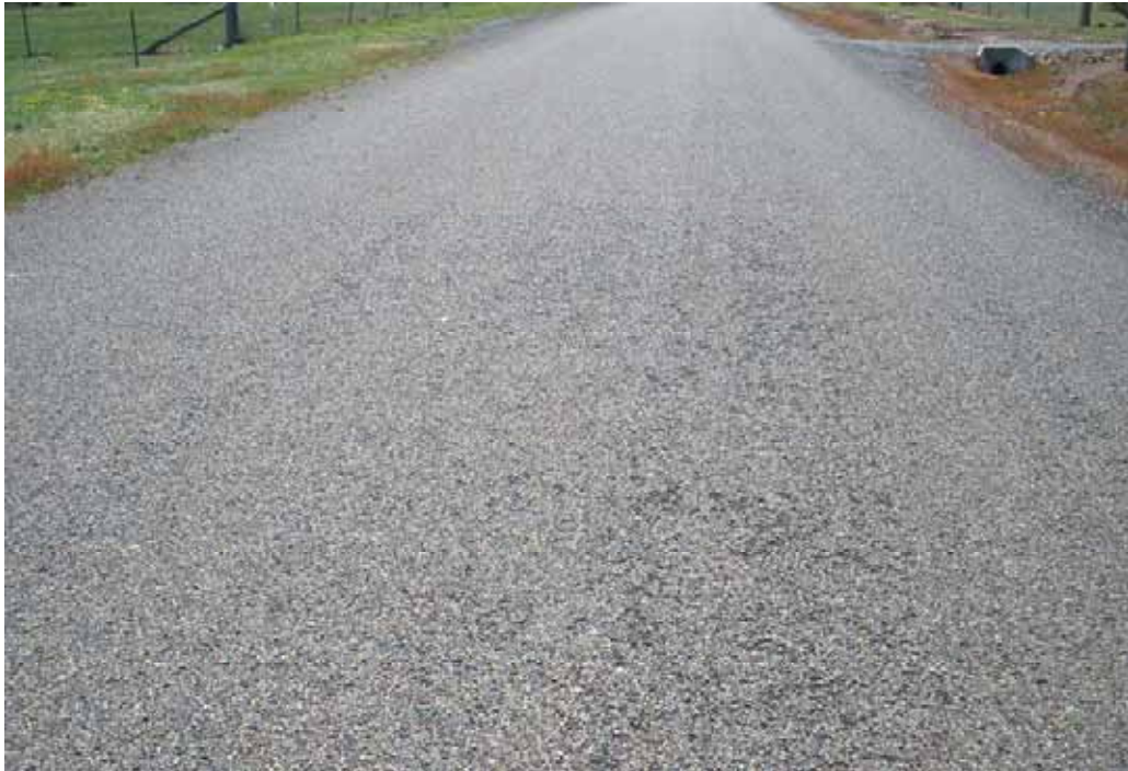
Photo 85 – Opposite Lots 18/19 Maclura Dr. Aggregate loss.
