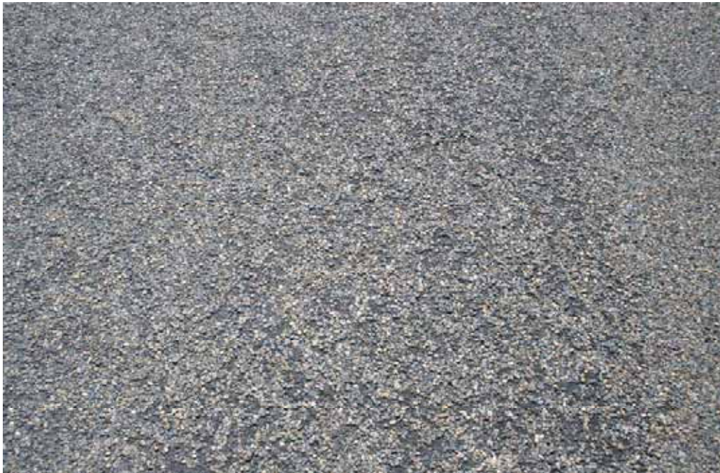
Photo 86 – Opposite Lots 18/19 Maclura Dr. Aggregate loss.
