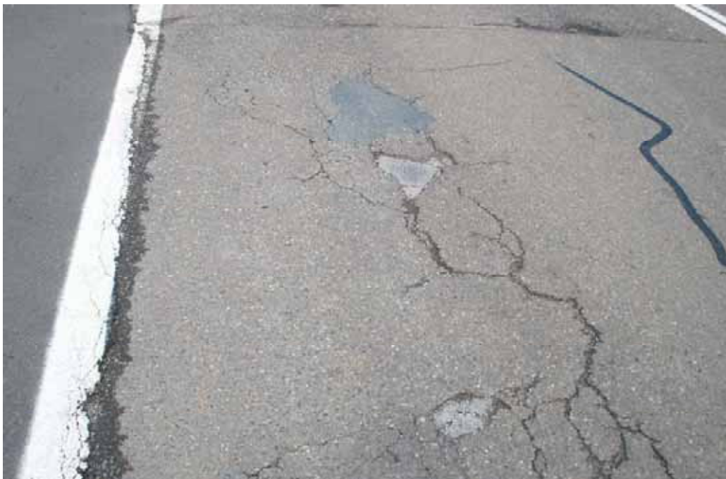
Photo 46 – Opposite park. Extensive pavement failure some old patches.
