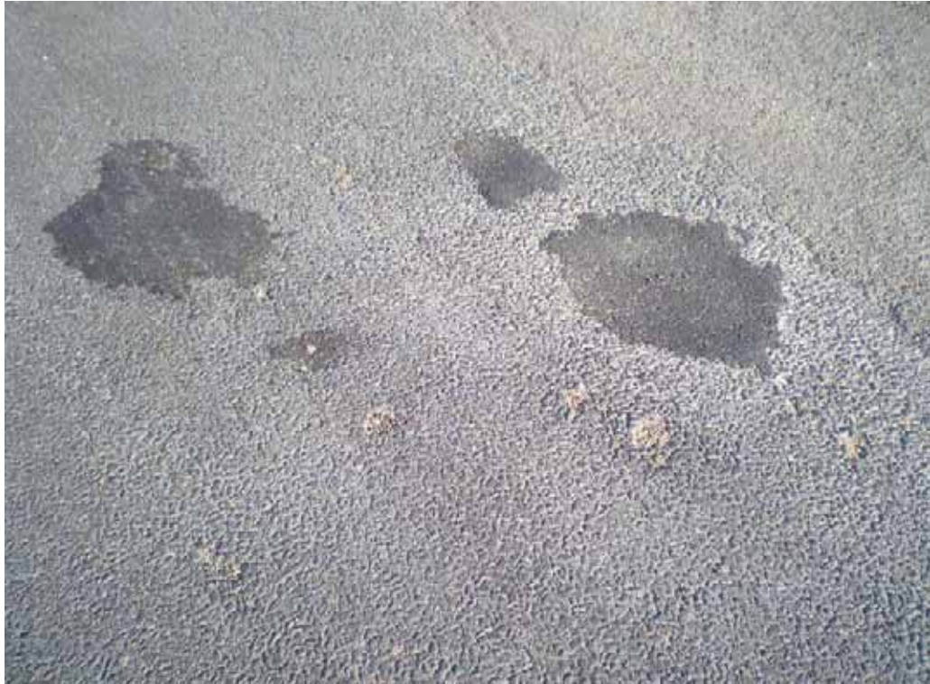
PHOTO 15: Repaired potholes, loss of seal
