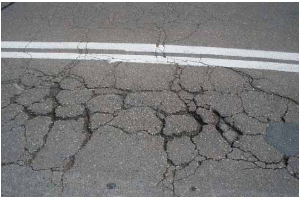
Photo 42 – Opposite park. Extensive pavement failure some old patches.
