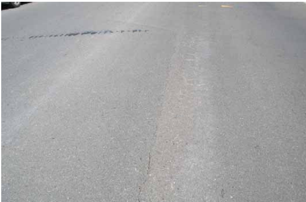
Photo 58 – Brayton Rd, near end of newer pavement. Difference in asphalt height possible rutting with cracking.
