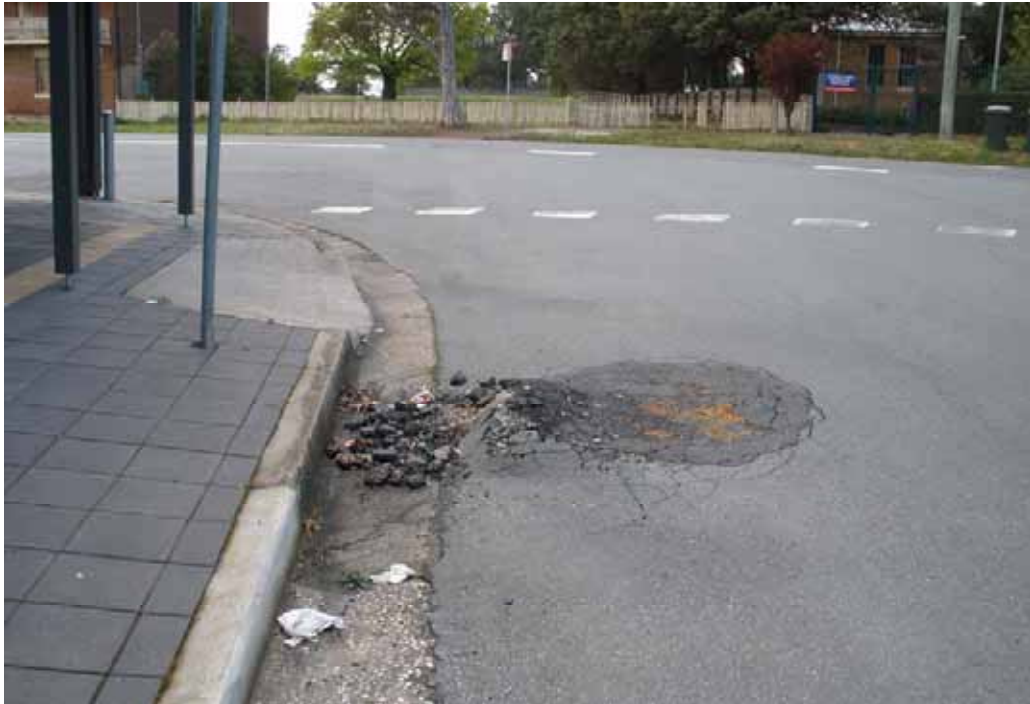
Photo 31 – Goulburn St at intersection with George St. Pavement failure in left wheel path.
