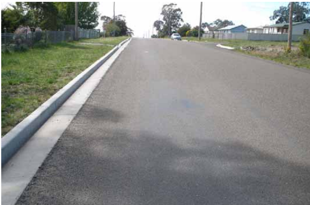
Photo 68 – Opposite No 39 Brayton Rd. Bitumen bleeding, start of small potholes and slight rutting.
