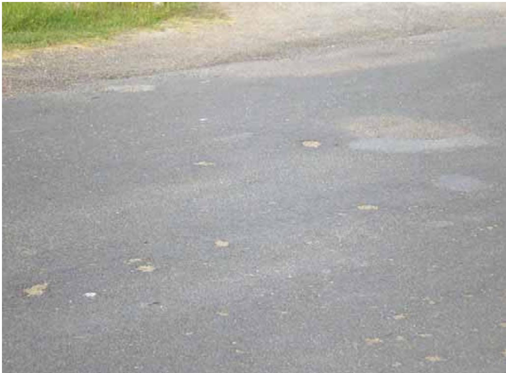
PHOTO 22: Loss of seal, repaired potholes
