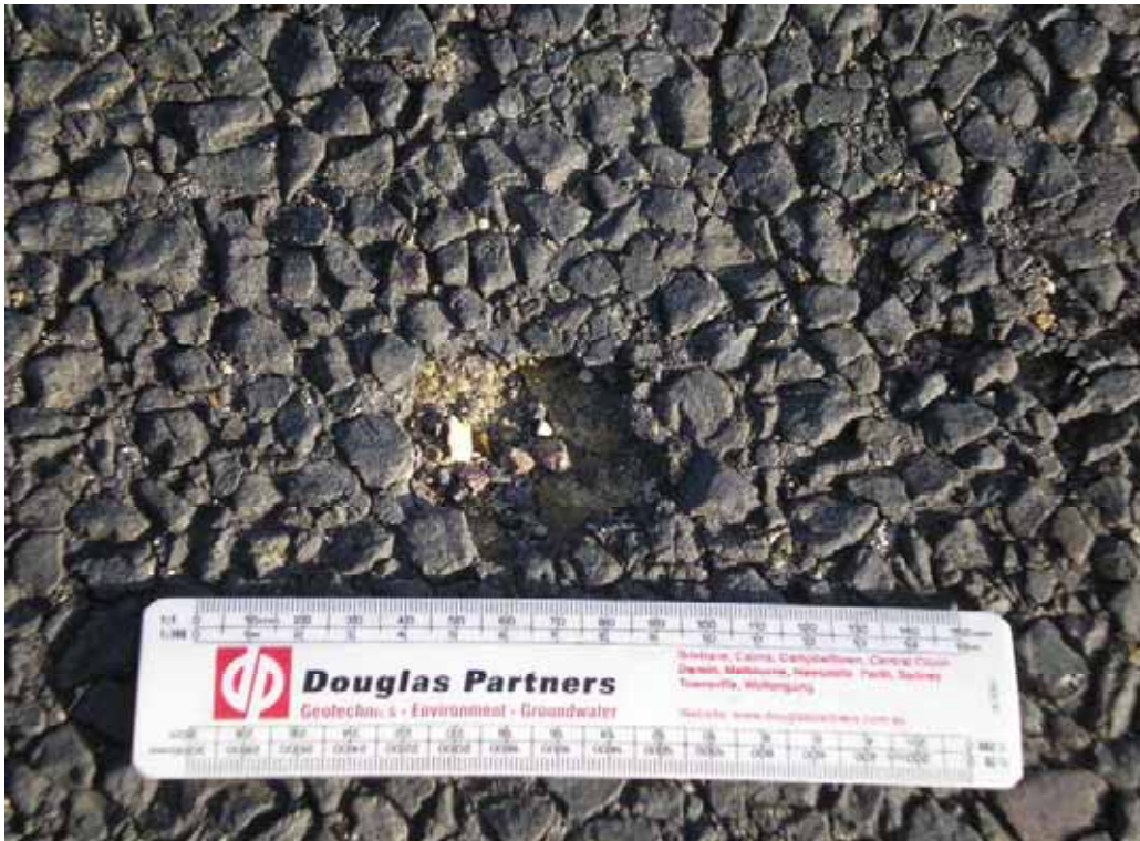
PHOTO 12: Loss of seal
