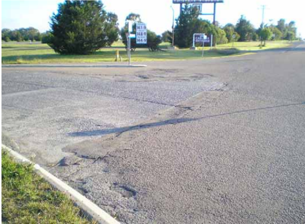
PHOTO 3: Cracking in asphalt at start of Portland Avenue
