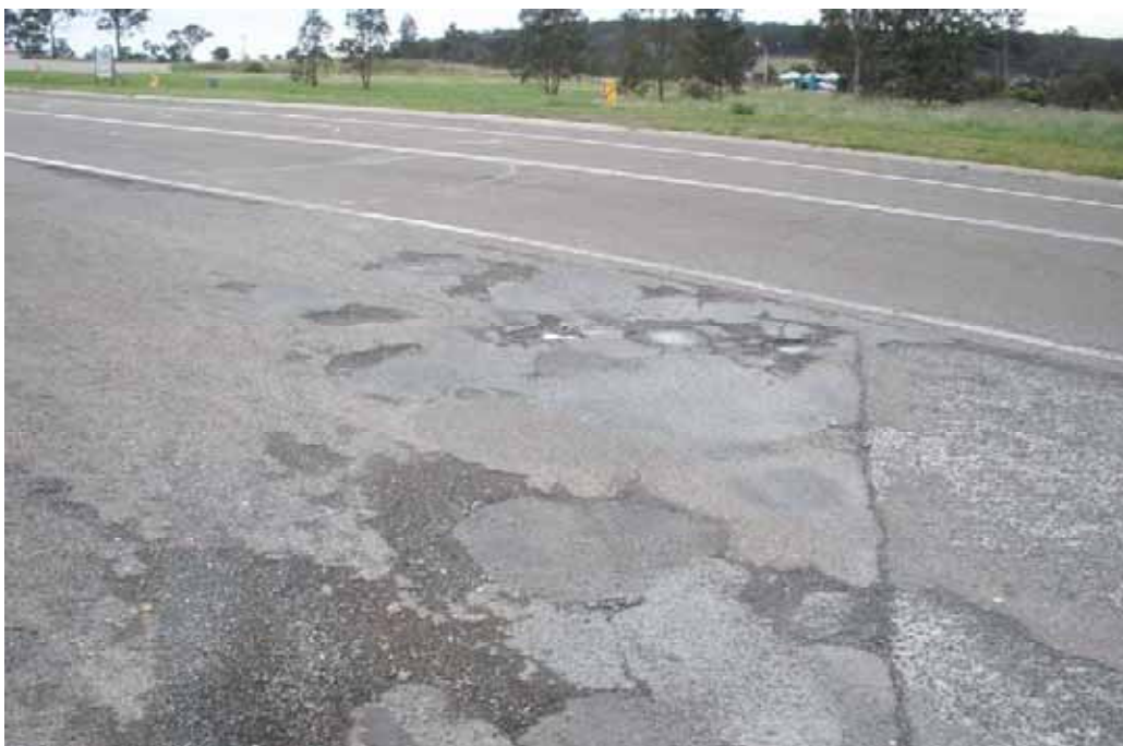
Photo 12 – Opposite exit driveway Truck Stop 31. New and repaired potholes in shoulder.
