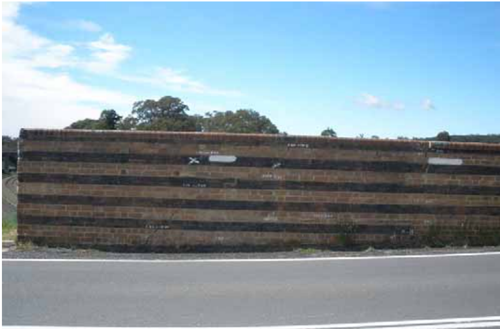
Photo 54 – Railway Bridge. Cracking in brick wall.
