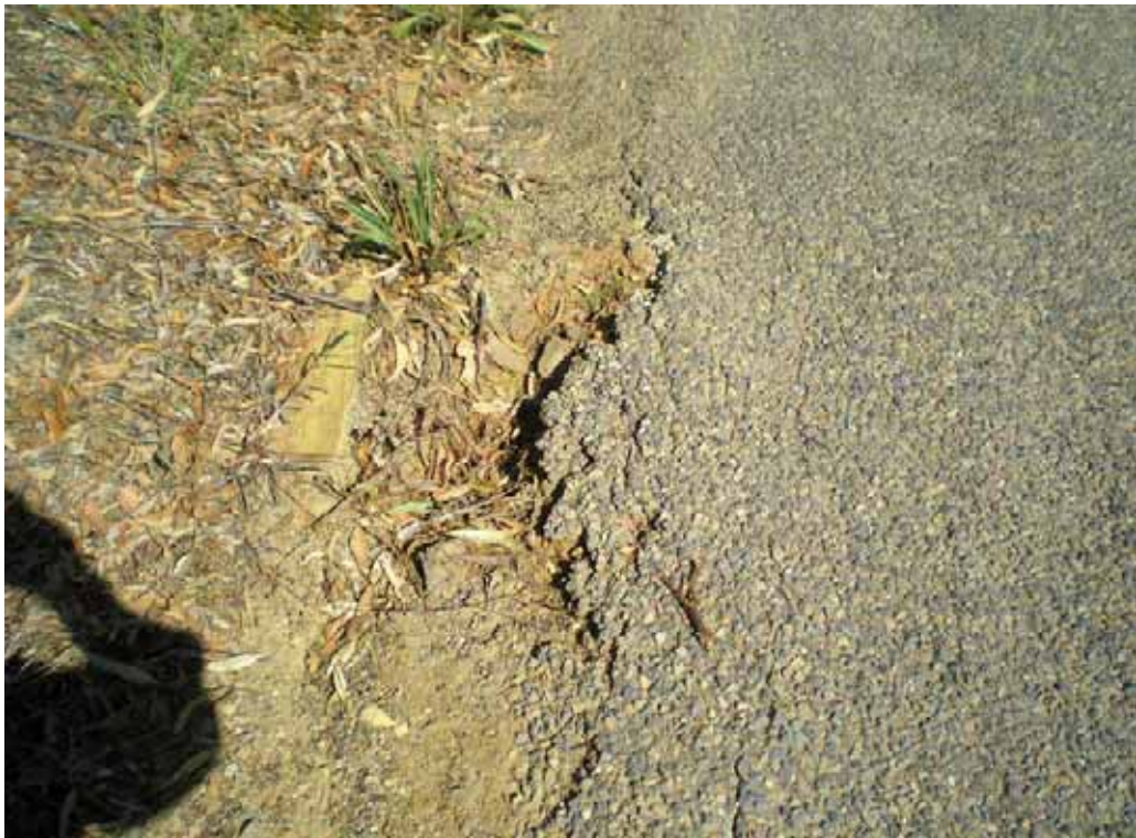
PHOTO 108: Pavement edge failure, erosion
