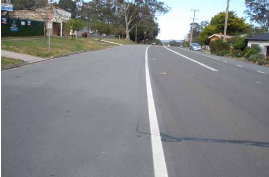
Photo 34 – Opposite school. Intermediate cracking along line marking edge.
