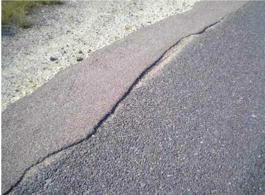
PHOTO 79: Lifting/shoving of shoulder repair/widening
