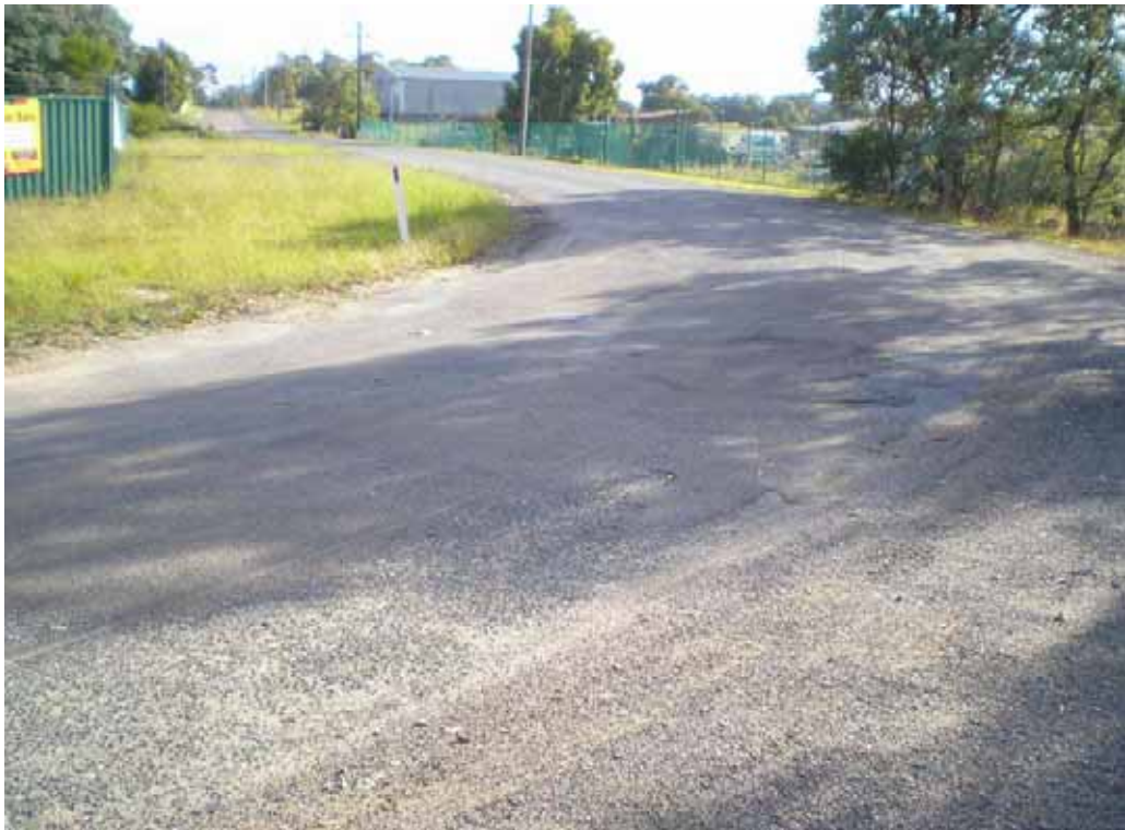
PHOTO 42: Loose gravel, repaired potholes/sections
