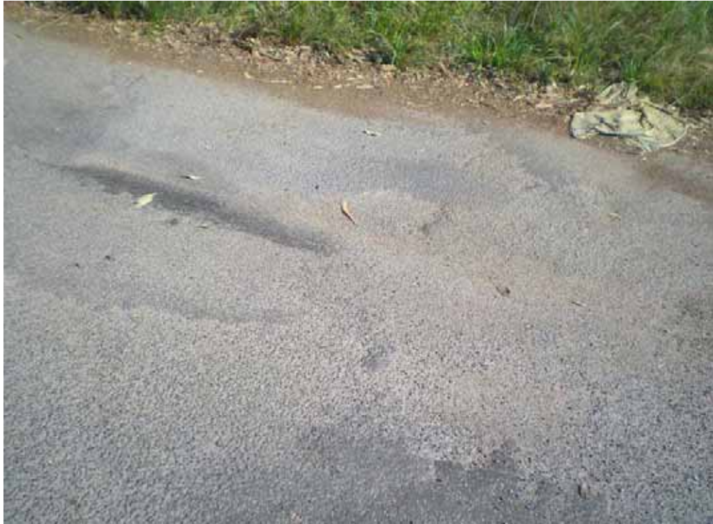
PHOTO 85: Settlement/rutting of repaired section at pavement edge
