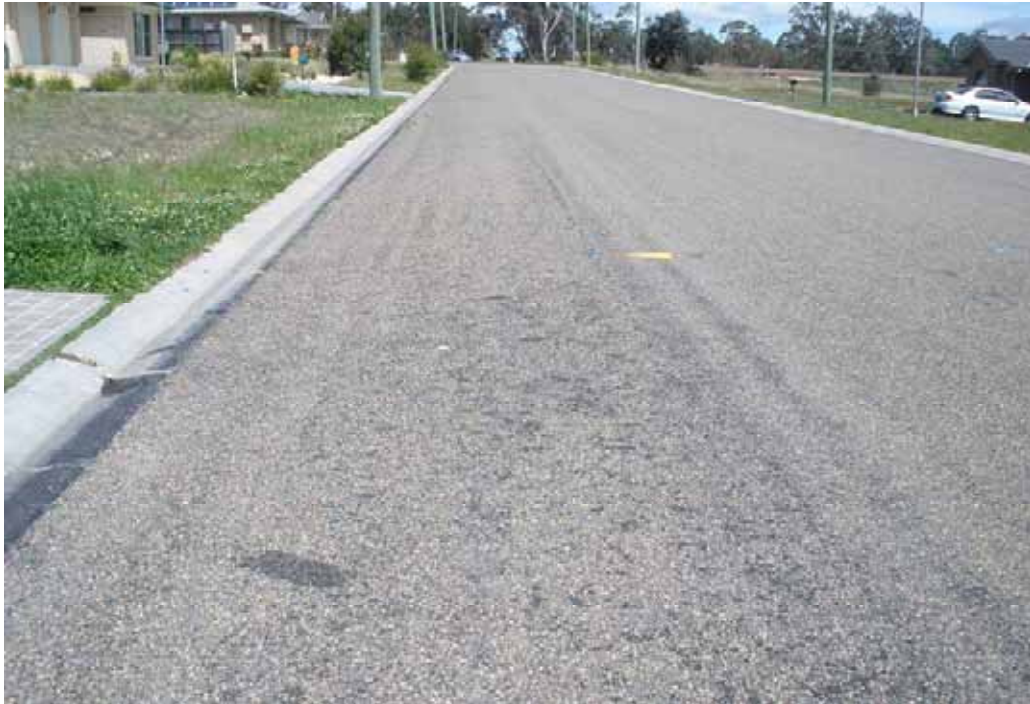
Photo 97 – Opposite No 15 Stoney Creek Rd. Bitumen bleeding and slight rutting.
