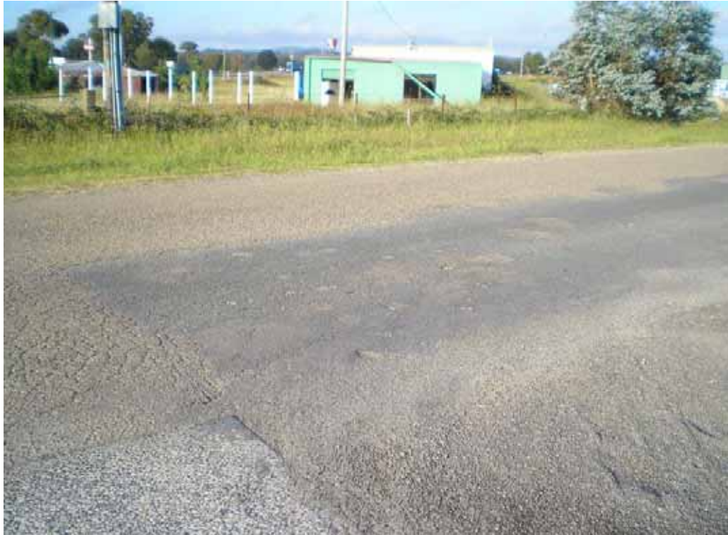
PHOTO 9: Change in seal, cracking in asphalt with some repaired sections
