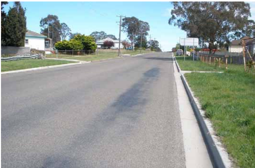
Photo 60 – Brayton Rd, edge of new/old pavement. Bitumen bleeding and slight rutting.
