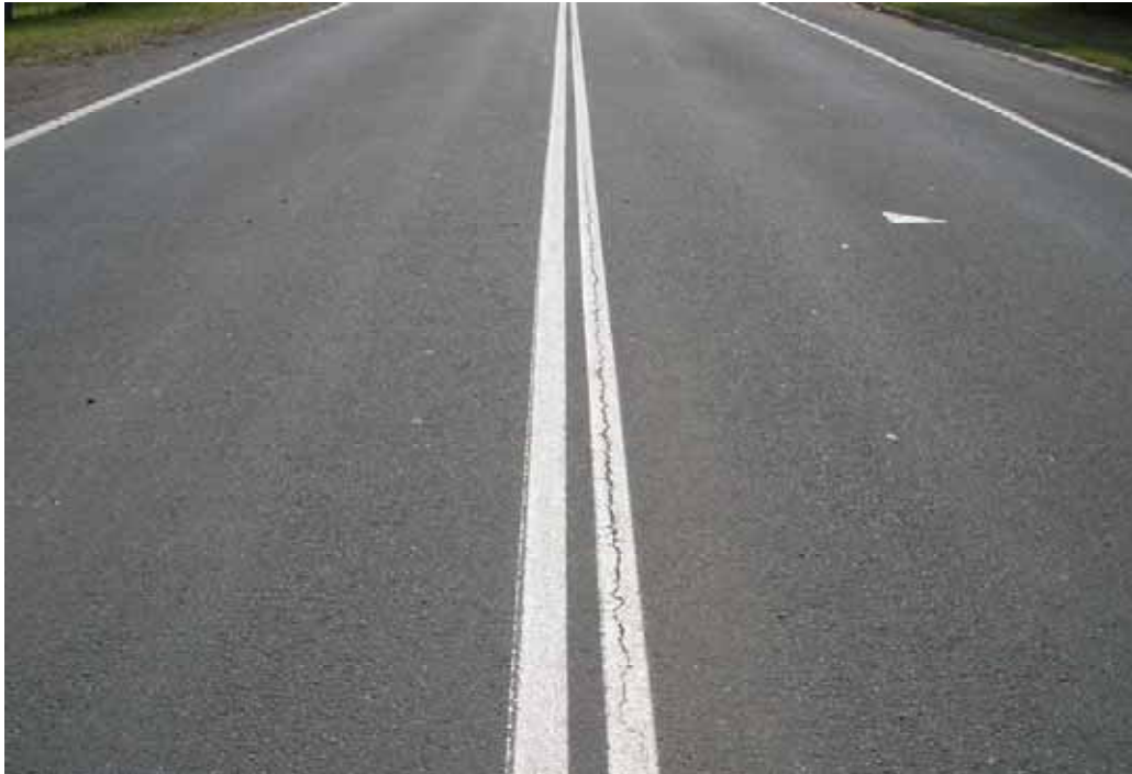
Photo 49 – Opposite police station. Longitudinal cracking in centre line marking.
