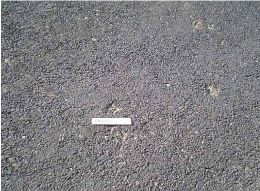
PHOTO 32: Loss of seal
