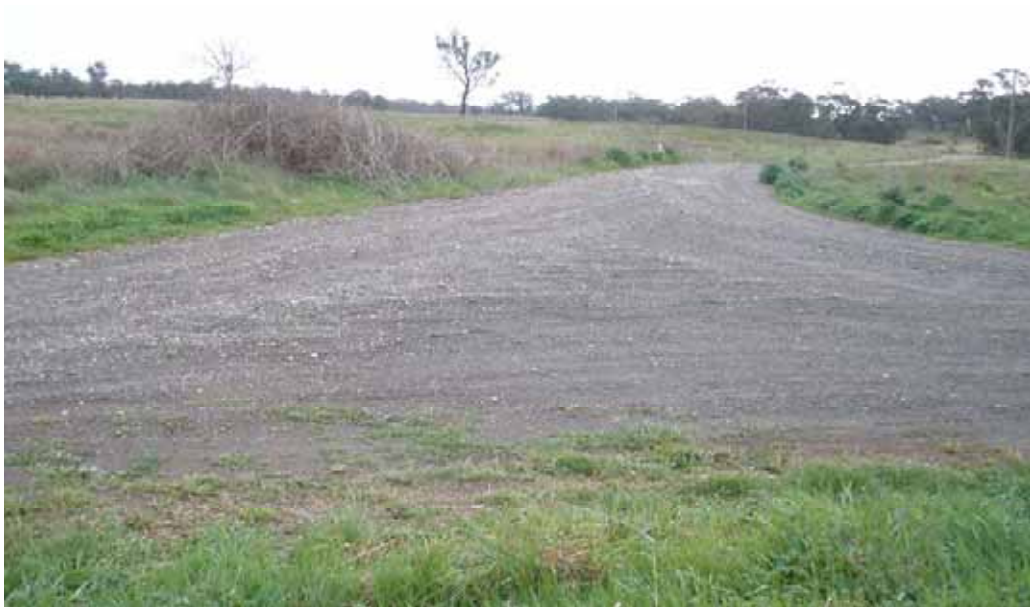
Photo 111 – Intersection of Stoney Creek Rd & Maclura Dr. Loose aggregate and uneven surface.
