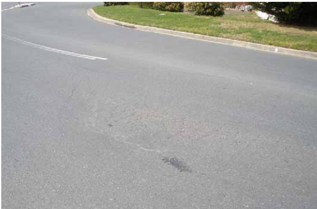
Photo 56 – Start of Brayton Rd. Crocodile cracking.
