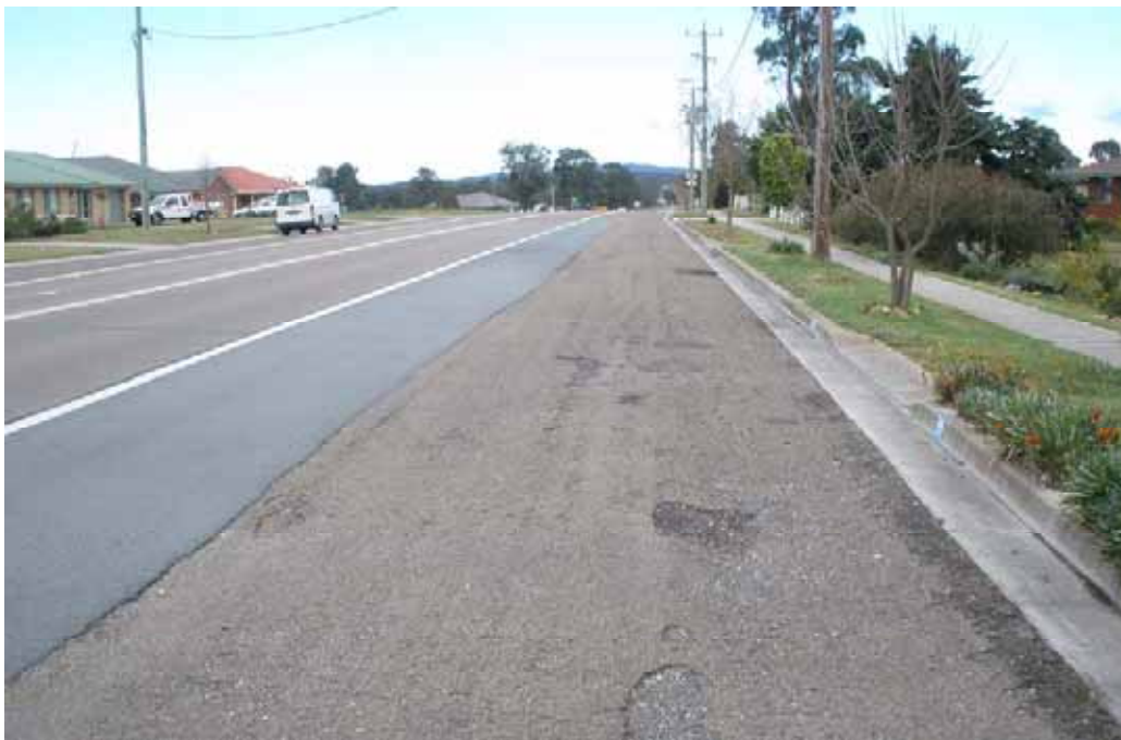
Photo 20 – Opposite No 36 George St. Resealed shoulder (west) with areas of wearing coarse loss/potholing.
