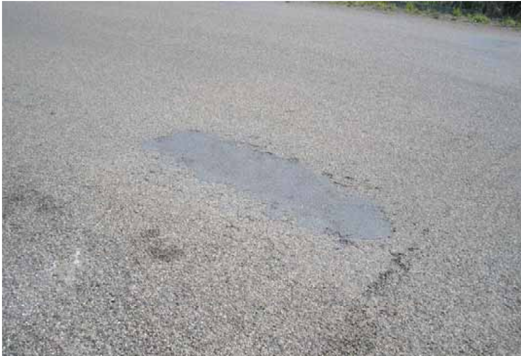
Photo 73 – Culvert structure neat tennis courts. Old repair patch with small failures surrounding.
