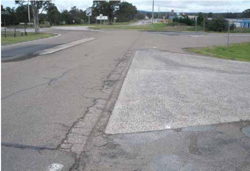
Photo 5 – Entrance to Truck Stop 31. Extensive edge failures and cracking. Some old patches.
