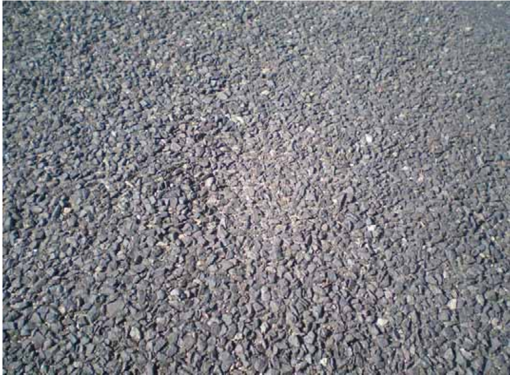
PHOTO 77: Depression in pavement
