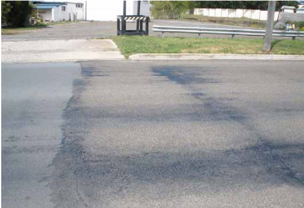
Photo 59 – Brayton Rd, edge of new/old pavement. Bitumen bleeding and slight rutting.
