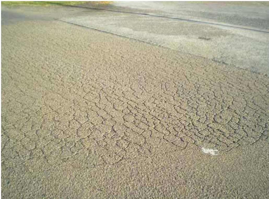
PHOTO 8: Cracking in asphalt
