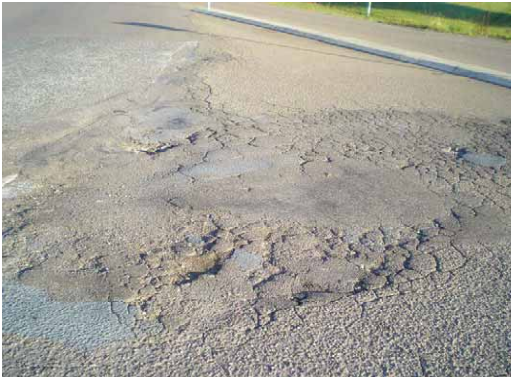
PHOTO 4: Cracking in asphalt and some repaired potholes
