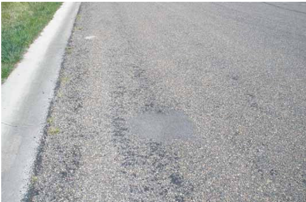
Photo 82 – Patrick Pl/Maclura Dr intersection. Repaired pothole and aggregate loss.
