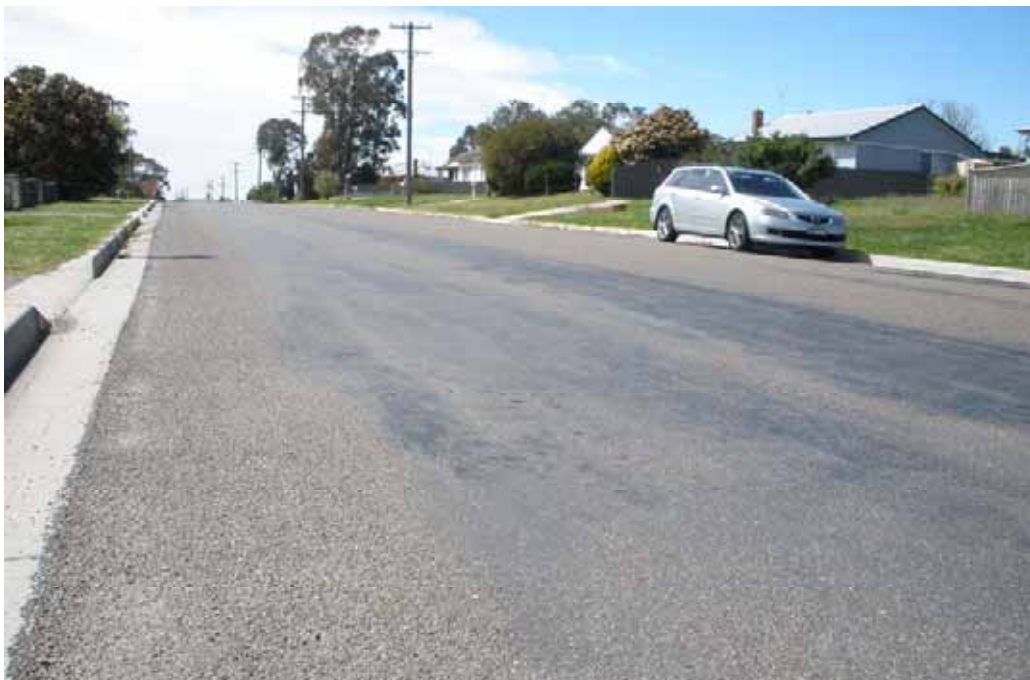
Photo 64 – Near Brayton Rd/Wollondilly St intersection. Bitumen bleeding, start of small potholes.
