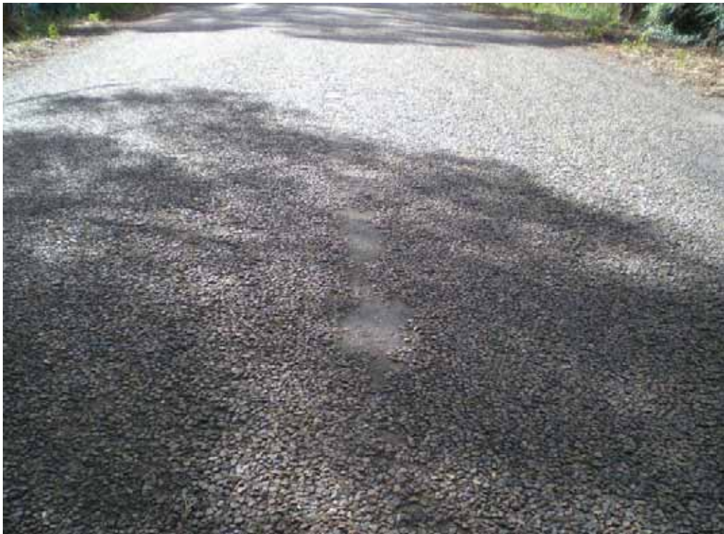
PHOTO 98: Stripped aggregate, settlement/rutting
