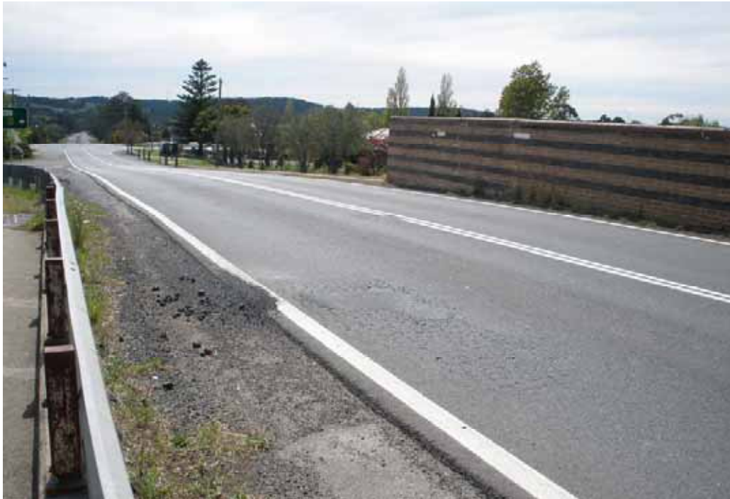
Photo 53 – Railway Bridge. Crocodile cracking with some patched areas and rutting.
