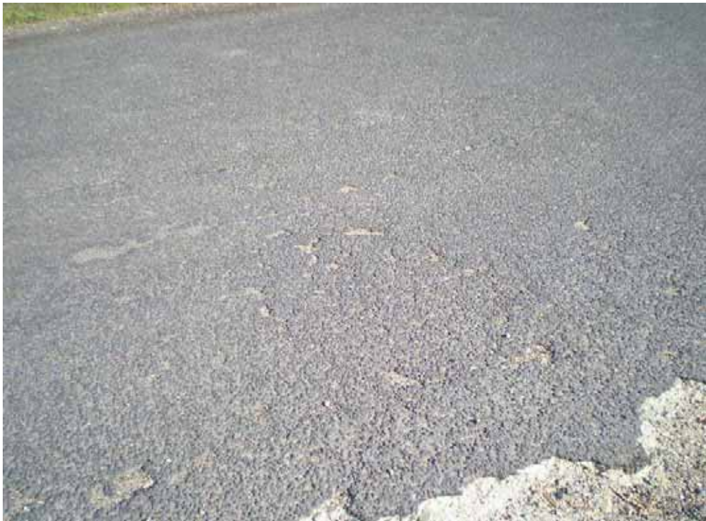
PHOTO 80: Loss of seal, cracking in asphalt
