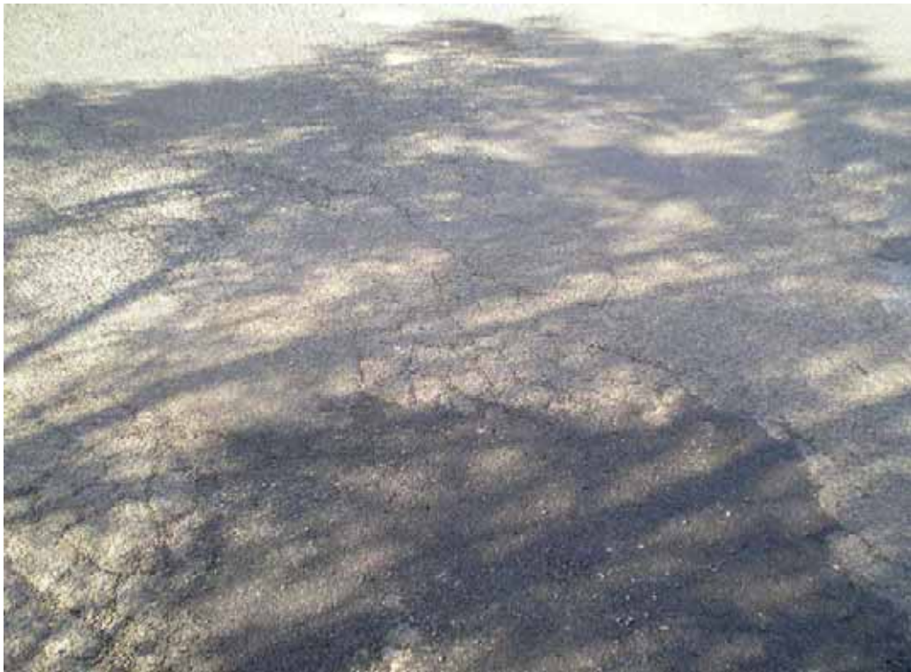
PHOTO 28: Cracking in asphalt, repaired potholes/section
