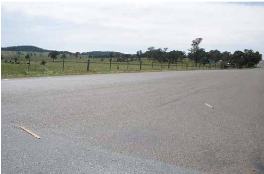
Photo 76 – Near Brayton Rd/Stony Creek Rd intersection. Rutting.
