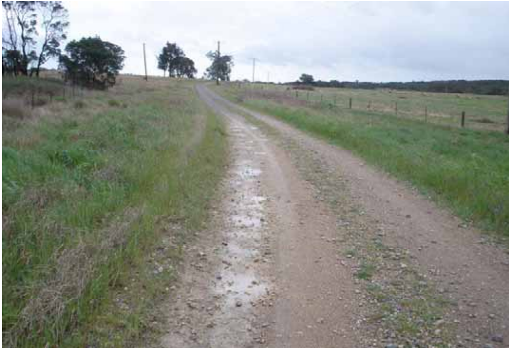
Photo 105 – Stoney Creek Rd (unsealed). Series of potholes southern side.
