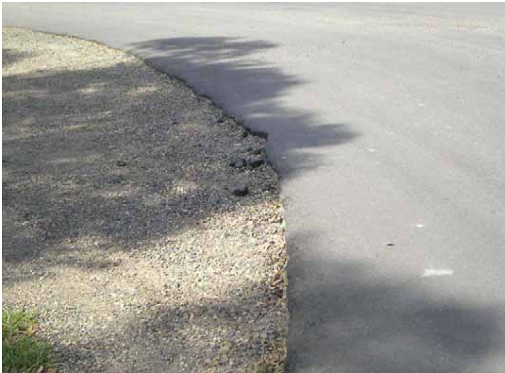
PHOTO 112: Edge failure of new seal at Orica gate
