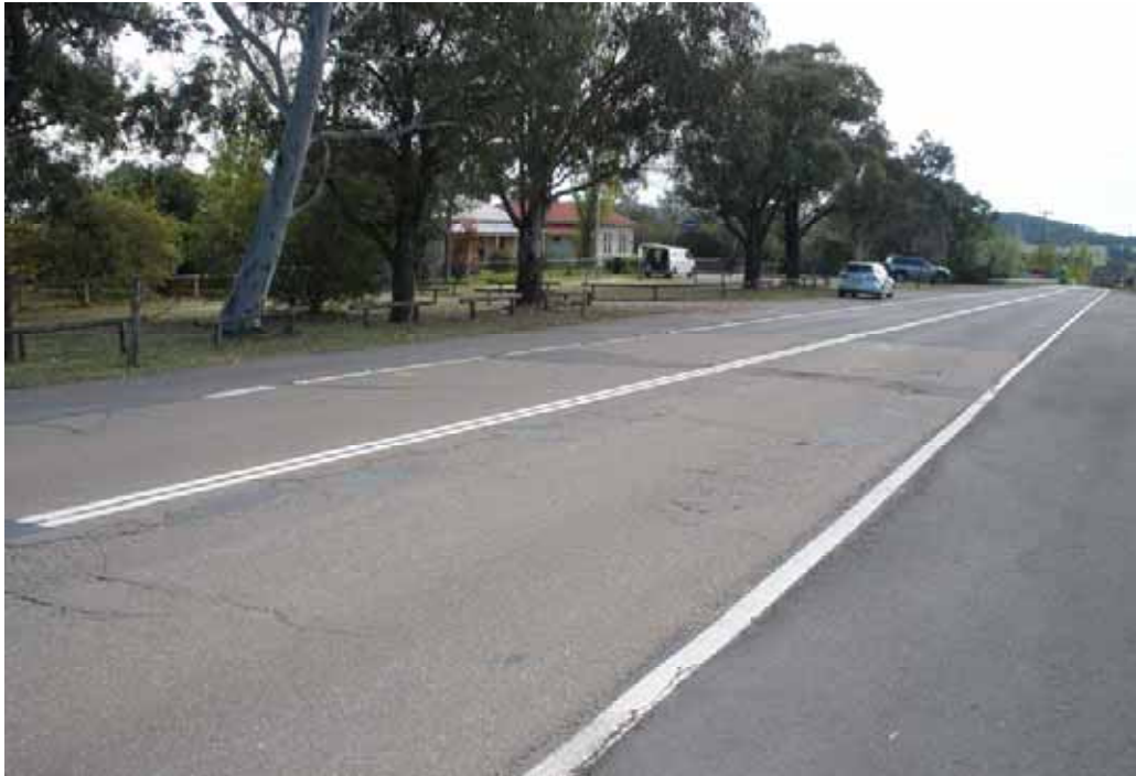
Photo 45 – Opposite park. Extensive pavement failure some old patches.
