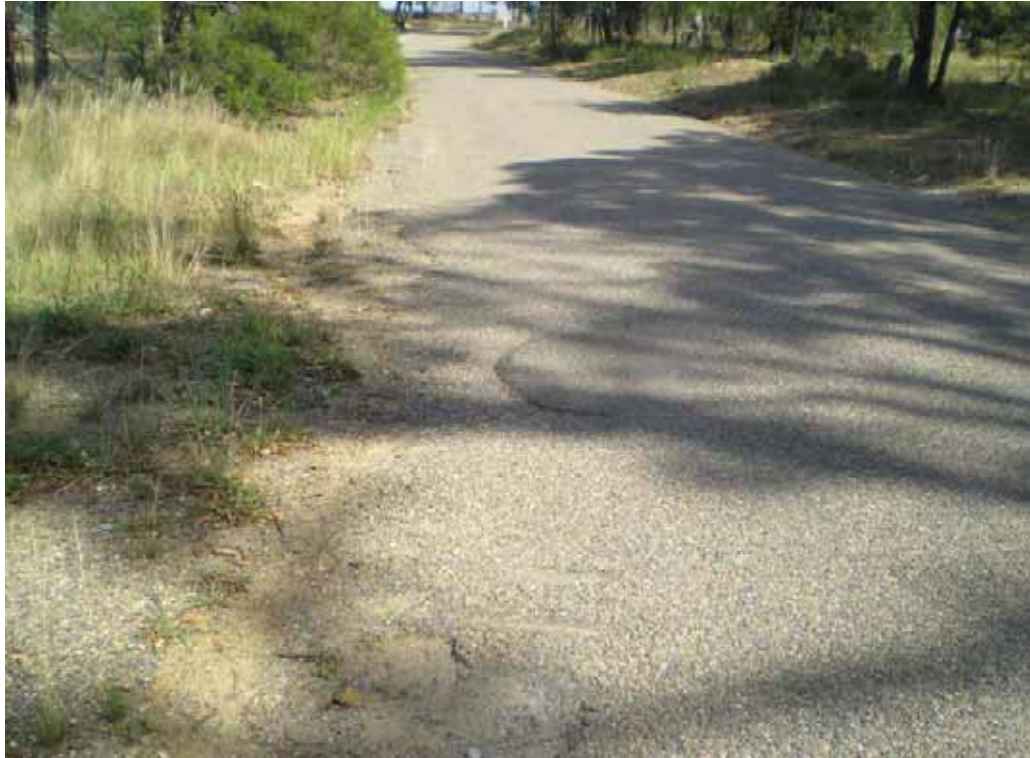
PHOTO 103: shoving of pothole repair, erosion at pavement edge
