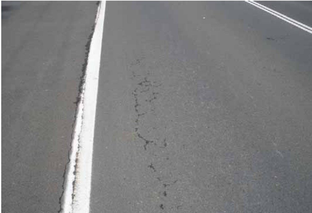
Photo 51 – Opposite police station. Start of crocodile cracking and longitudinal cracking along edge lane marking.
