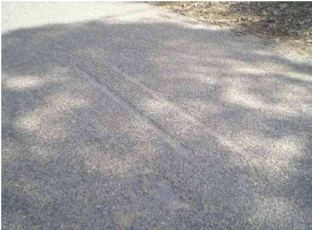
PHOTO 110: Gouging of asphalt
