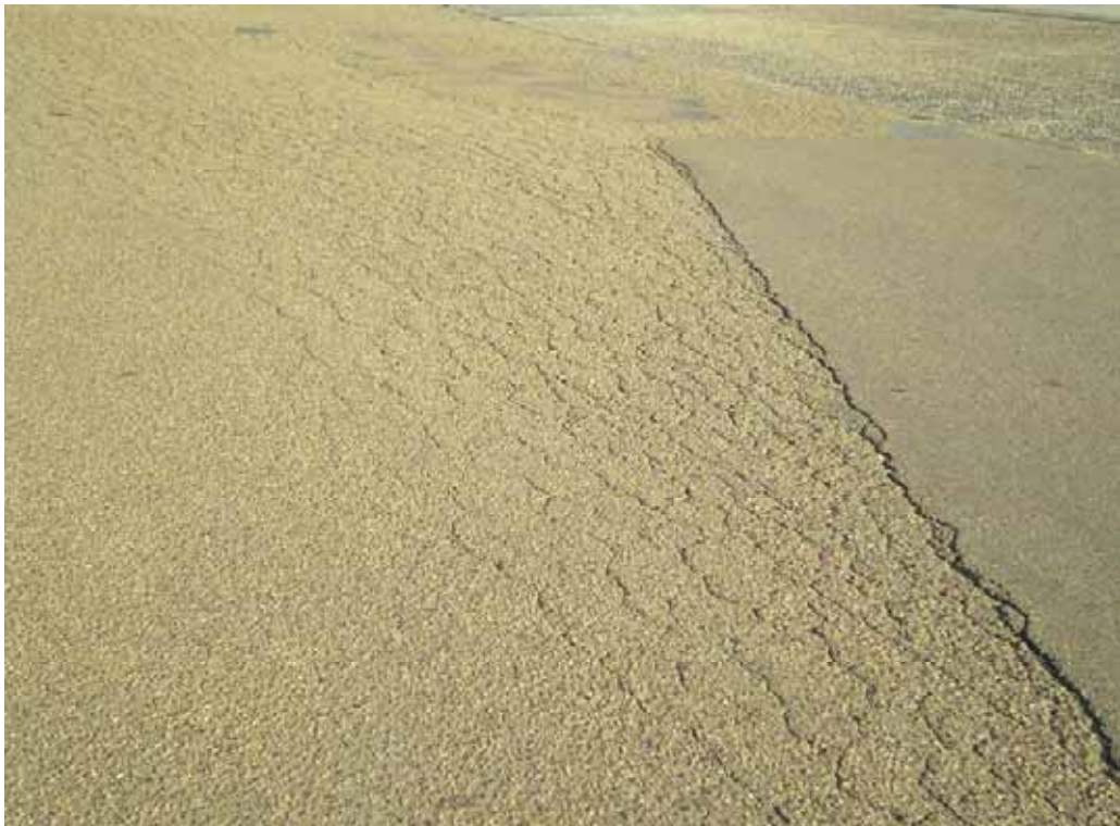
PHOTO 6: Cracking in asphalt next to repaired section
