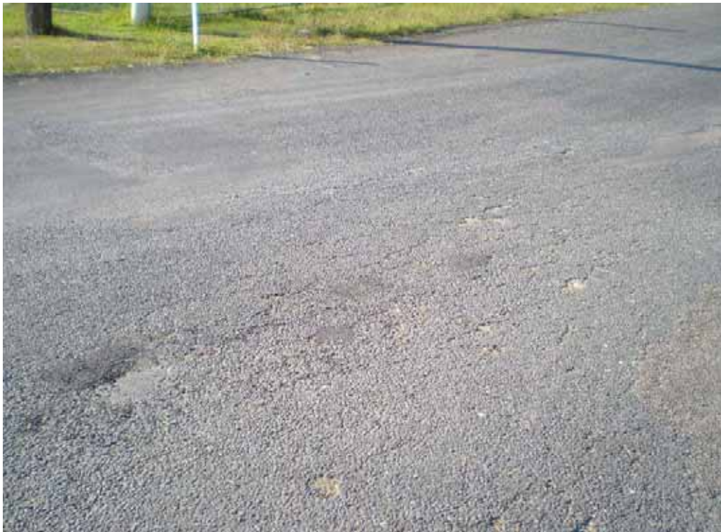
PHOTO 30: Loss of seal, cracking in asphalt, repaired sections/potholes
