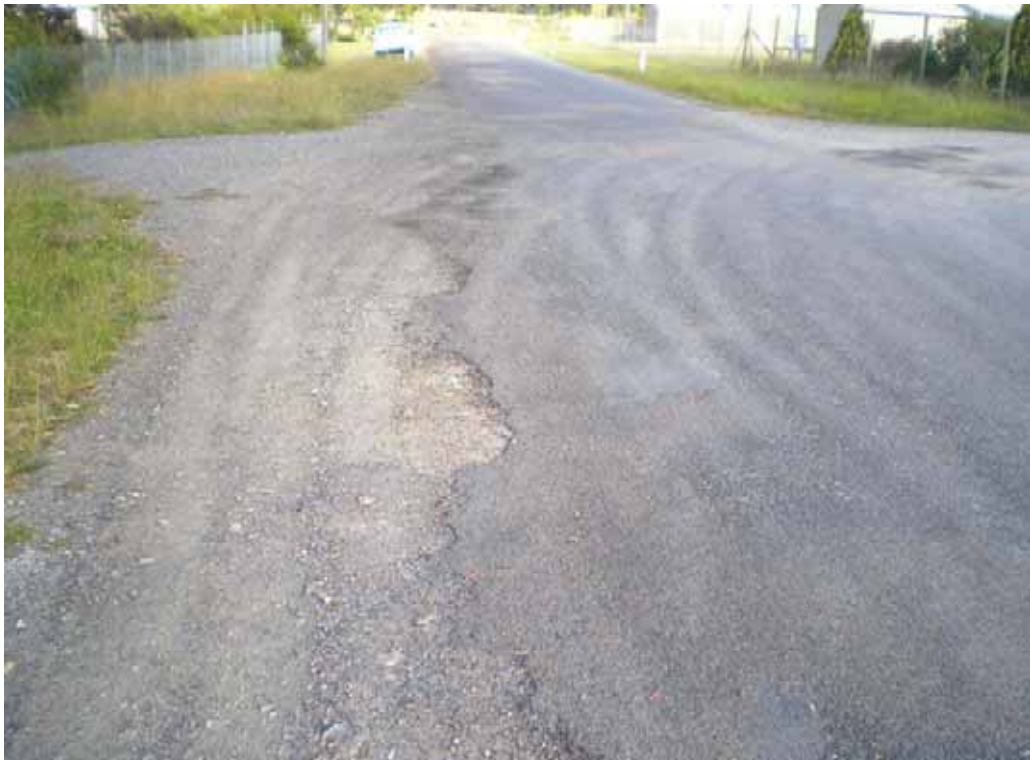
PHOTO 48: Entrance to Ploughmaster Engineering, shoulder failures and repairs
