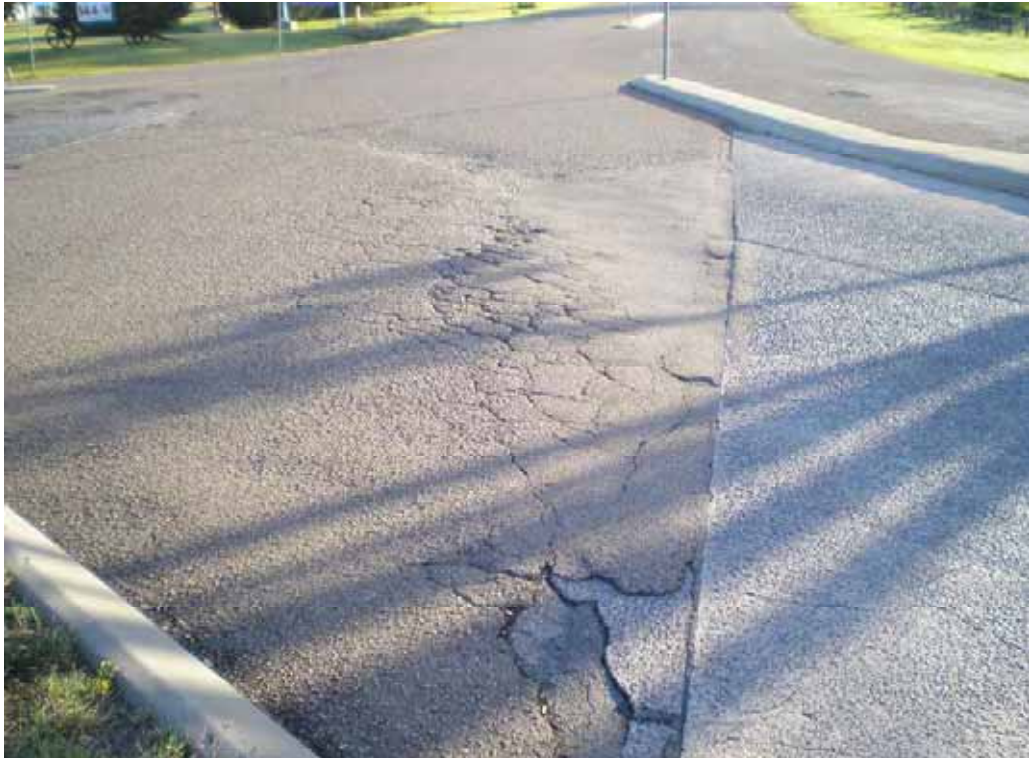
PHOTO 2: Cracking in asphalt at edge of roundabout
