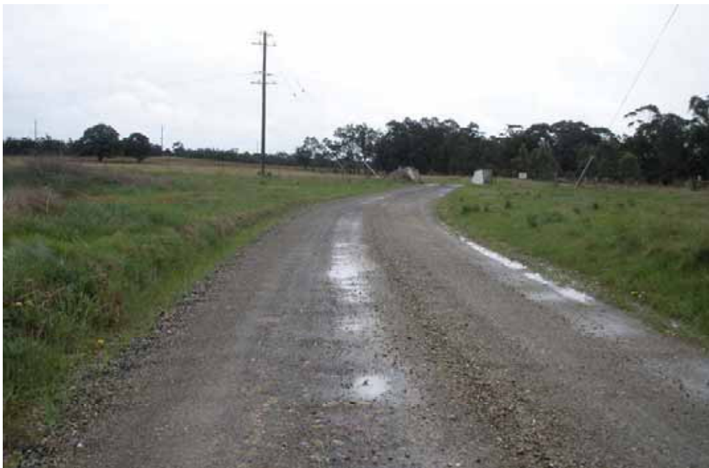
Photo 118 – Stoney Creek Rd (unsealed). Small potholes, uneven surface and corrugations.
