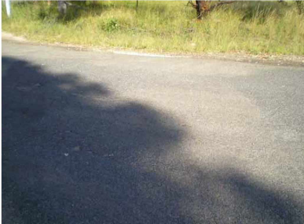
PHOTO 81: Repaired sections/potholes, loss of seal, settlement/rutting
