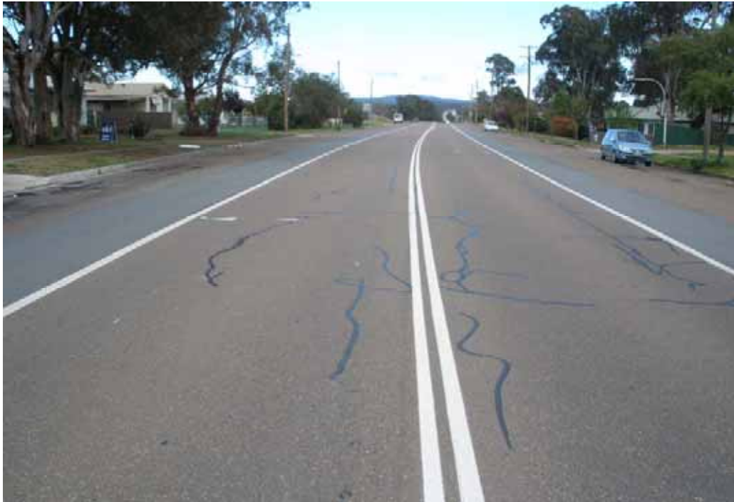
Photo 25 – Opposite Brewer Centre. Bitumen emulsion sealed cracks and some unsealed cracks.
