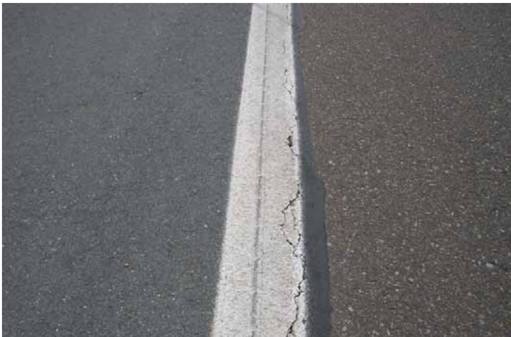
Photo 22 – Opposite No 39 George St. Longitudinal cracking at edge of line marking.
