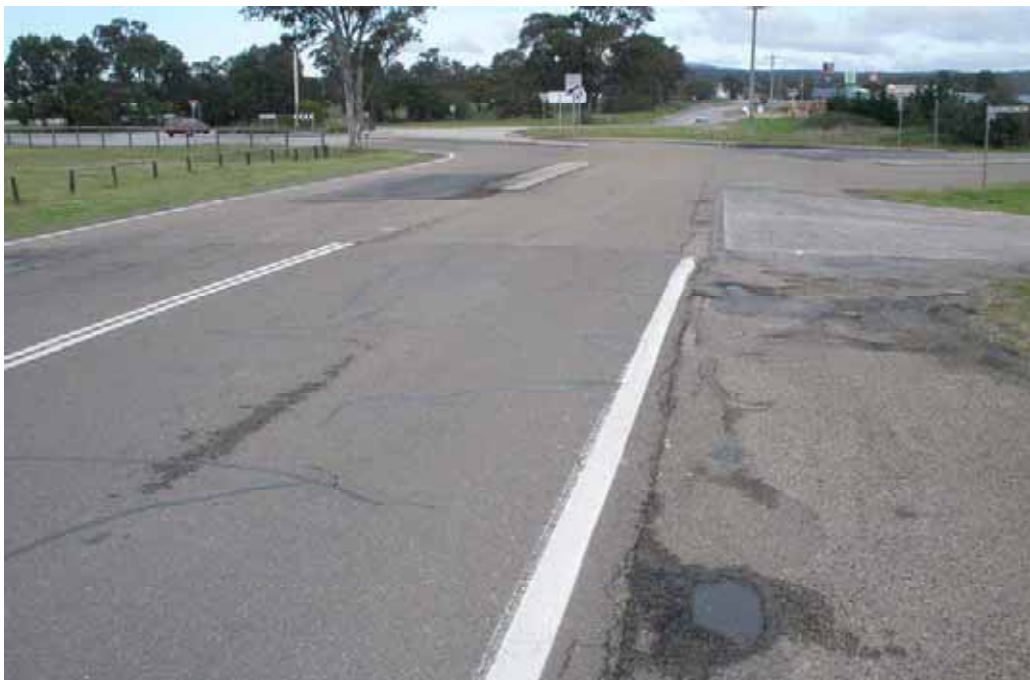
Photo 6 – Entrance to Truck Stop 31. Extensive edge failures and cracking. Some old patches and bitumen emulsion sealing of old cracks.
