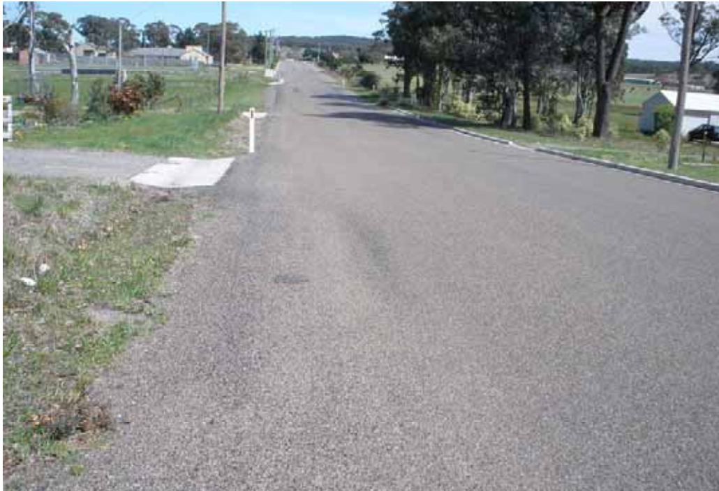
Photo 69 – Opposite No 51 Brayton Rd. Bitumen bleeding and slight rutting.
