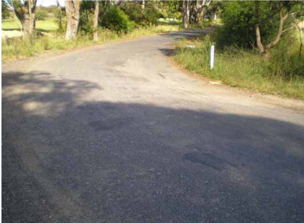
PHOTO 83: Numerous failed and repaired section/potholes
