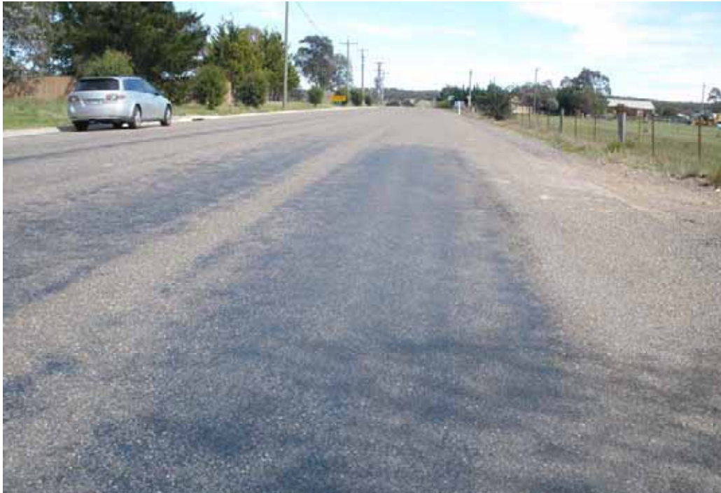
Photo 75 – Opposite No 72 Brayton Rd. Bitumen bleeding and rutting.
