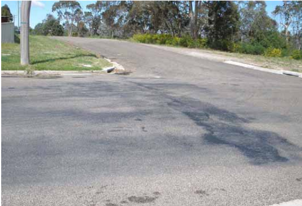
Photo 65 –Brayton Rd/Wollondilly St intersection. Bitumen bleeding, start of small potholes and slight rutting.
