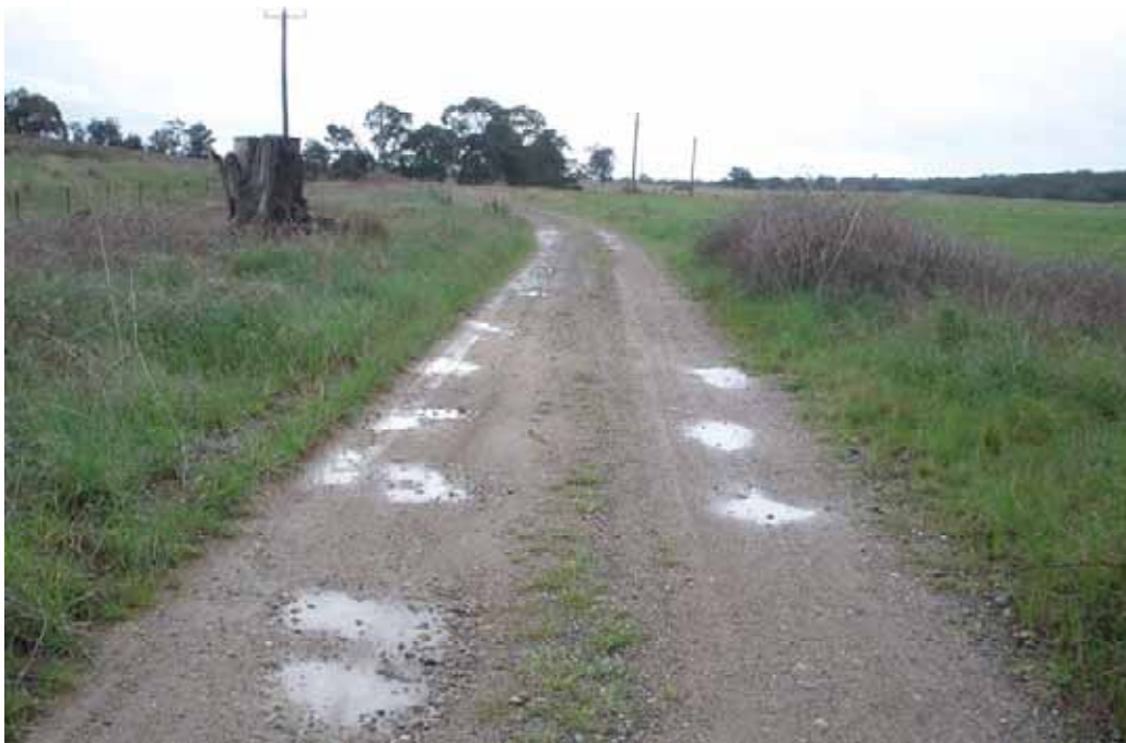
Photo 102 – Stoney Creek Rd (unsealed). Series of potholes.
