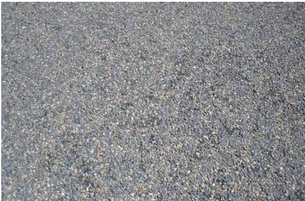
Photo 84 – Opposite No 38 Maclura Dr. Aggregate loss.
