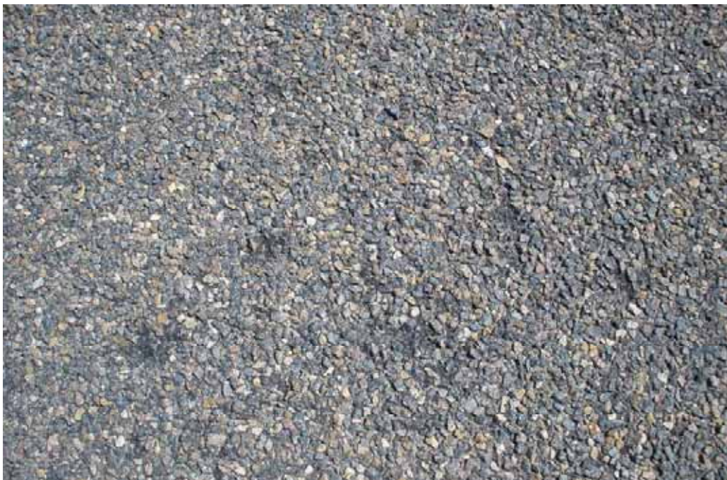
Photo 78 – Start of Maclura Dr. Aggregate loss.
