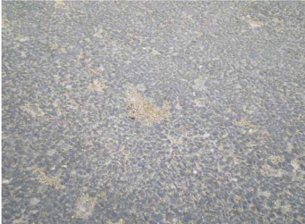
PHOTO 35: Loss of seal
