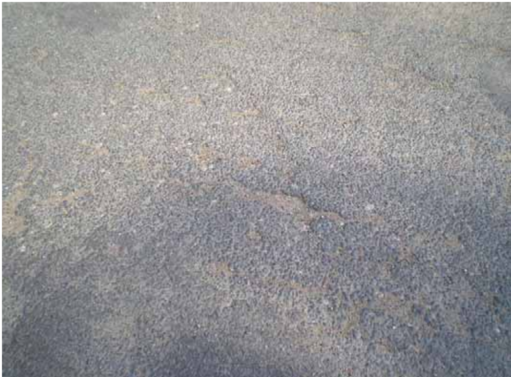
PHOTO 84: Loss of seal, cracking in asphalt
