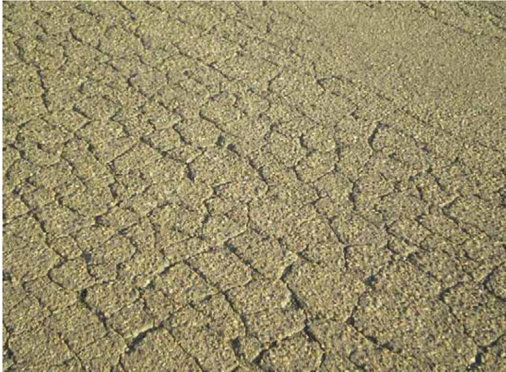
PHOTO 7: Cracking in asphalt
