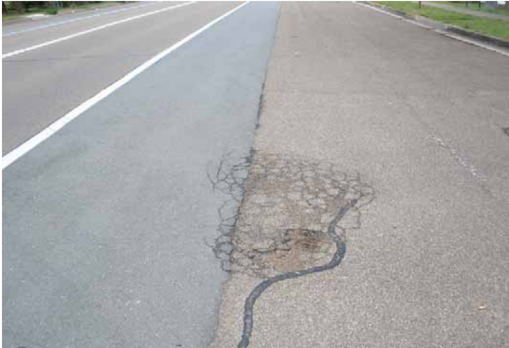
Photo 23 – Opposite Marulan Auto Port (south). Crocodile cracking.
