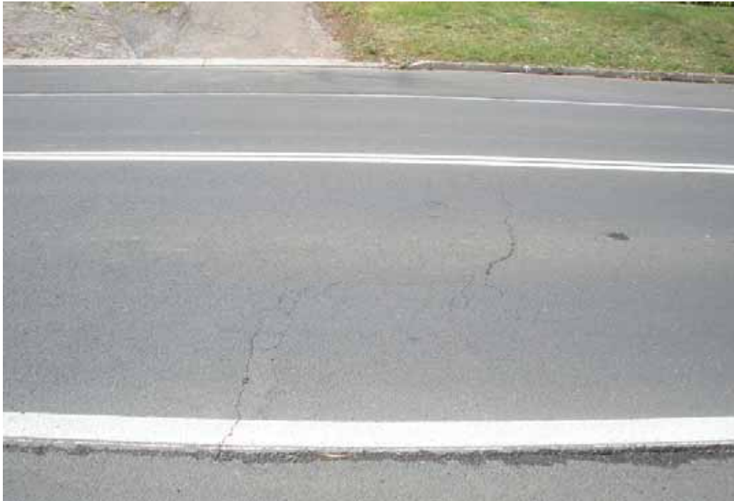
Photo 47 – Opposite Uniting Church. Cracking in section of newer pavement.
