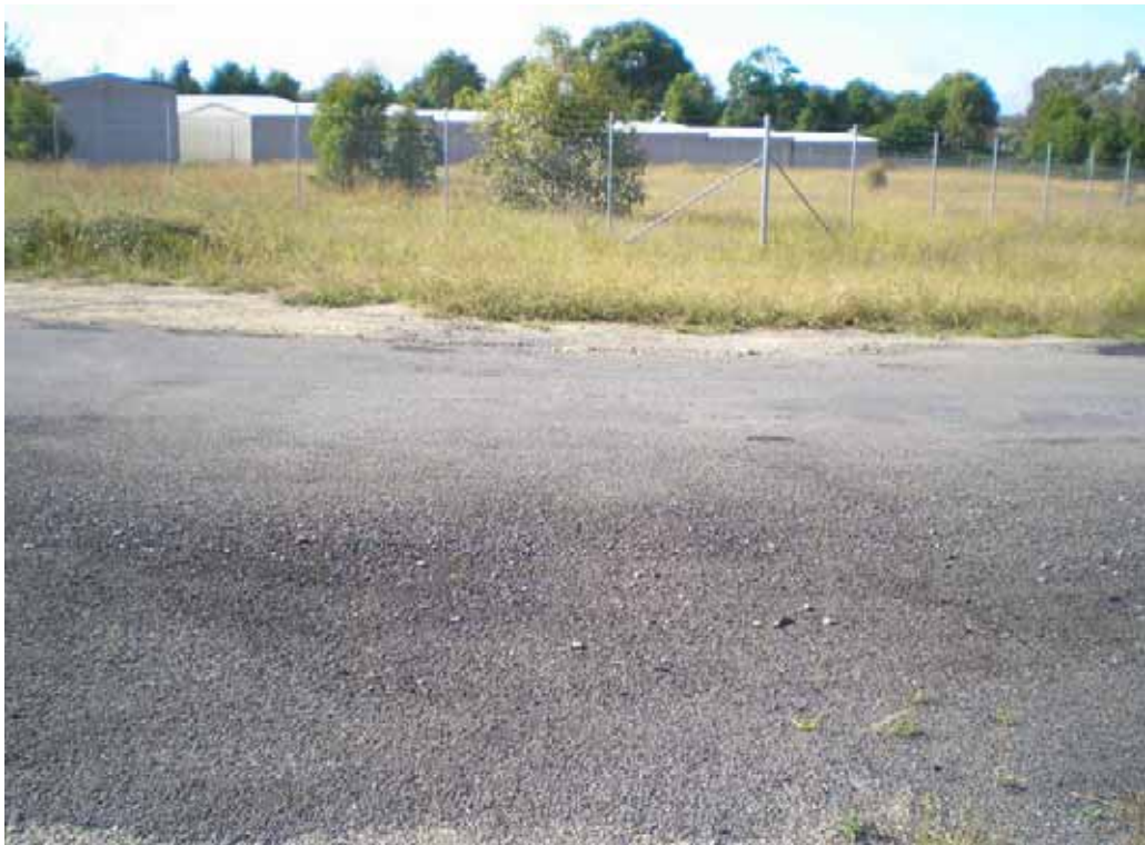
PHOTO 62: Loose gravel at pavement edge
