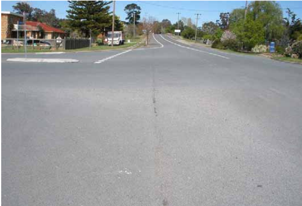
Photo 55 – Intersection of George St/Brayton Rd. Cracking along pavement joints.
