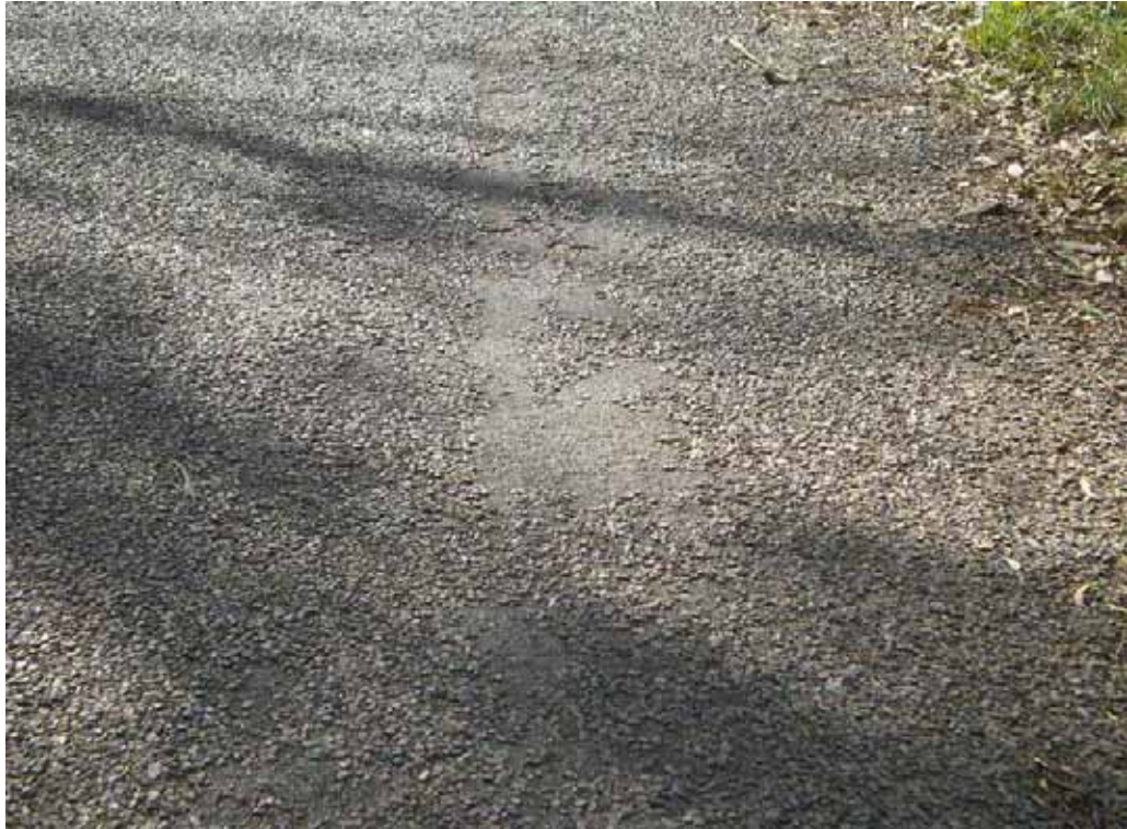
PHOTO 91: Stripped aggregate, slight rutting
