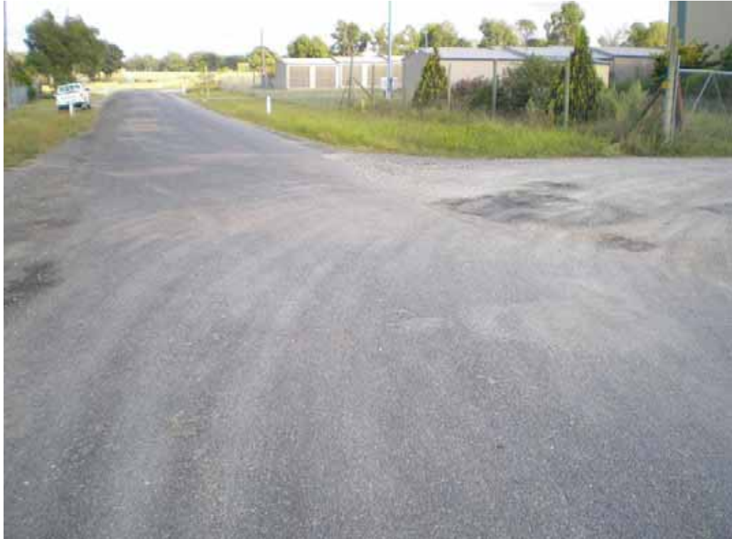
PHOTO 49: Entrance to Ploughmaster Engineering, loss of seal, repaired sections
