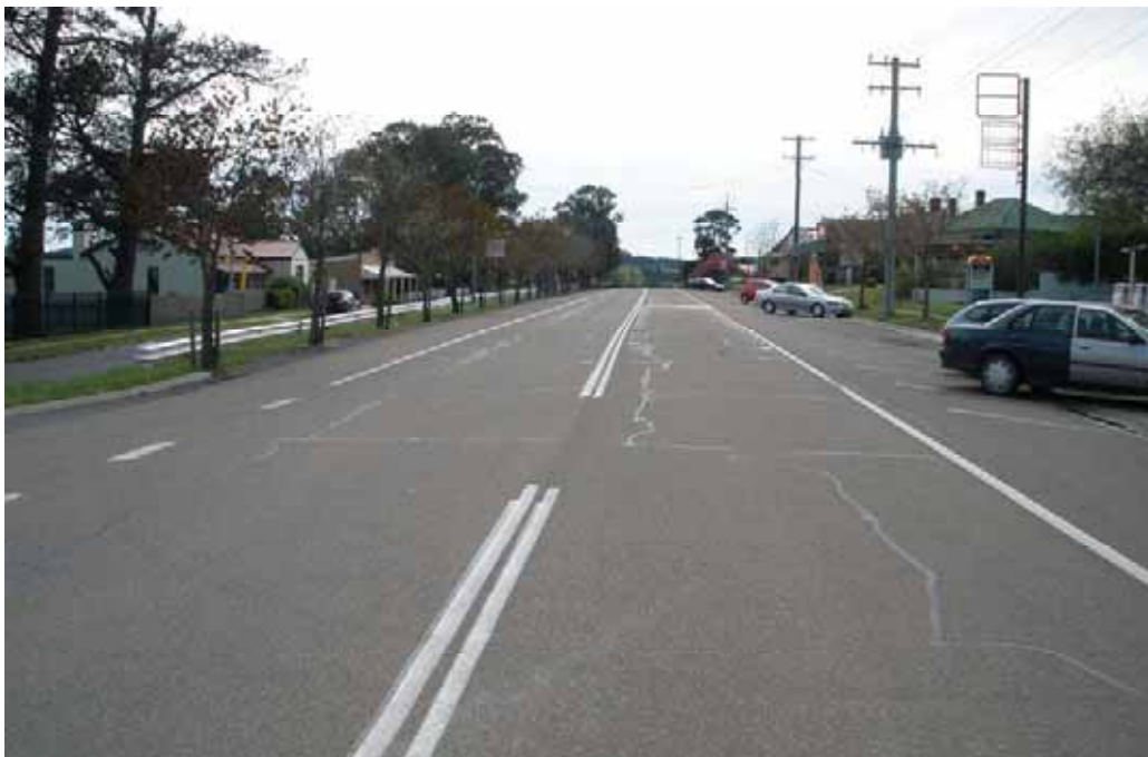
Photo 36 – Opposite butcher. Numerous cracking mainly sealed with bitumen emulsion some unsealed.
