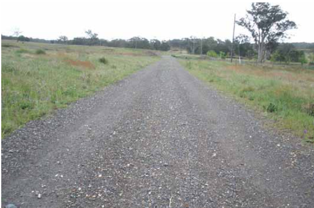
Photo 110 – Stoney Creek Rd (unsealed). Depressioning along both wheel paths.
