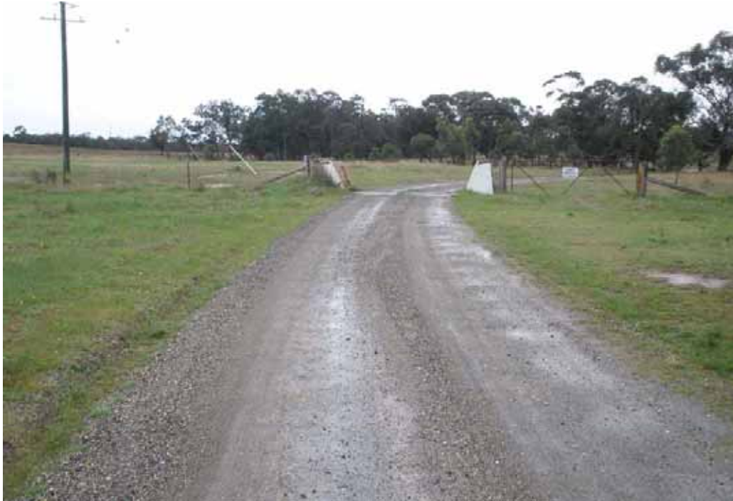
Photo 119 – Stoney Creek Rd (unsealed)/stock grid. Small potholes, uneven surface and corrugations.
