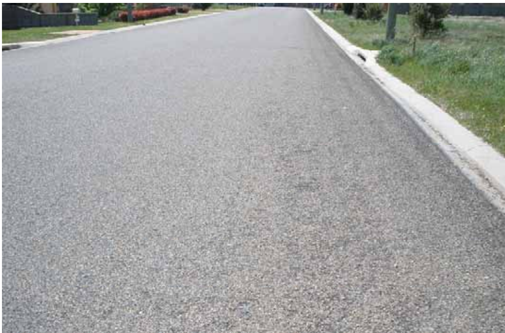
Photo 92 – Opposite No 22 Stoney Creek Rd. Aggregate loss and slight rutting.
