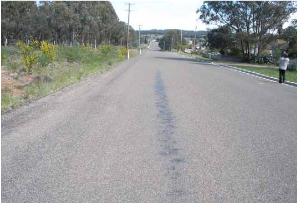
Photo 67 – Near Brayton Rd/Wollondilly St intersection. Bitumen bleeding, start of small potholes.
