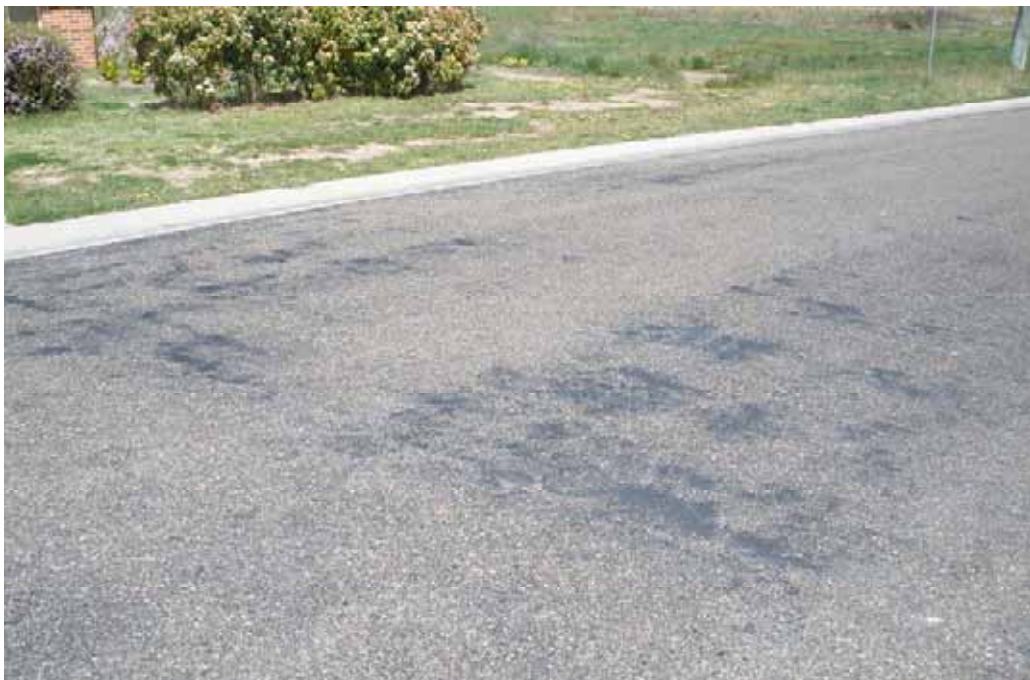
Photo 80 – Near Patrick Pl/Maclura Dr intersection. Bitumen bleeding.
