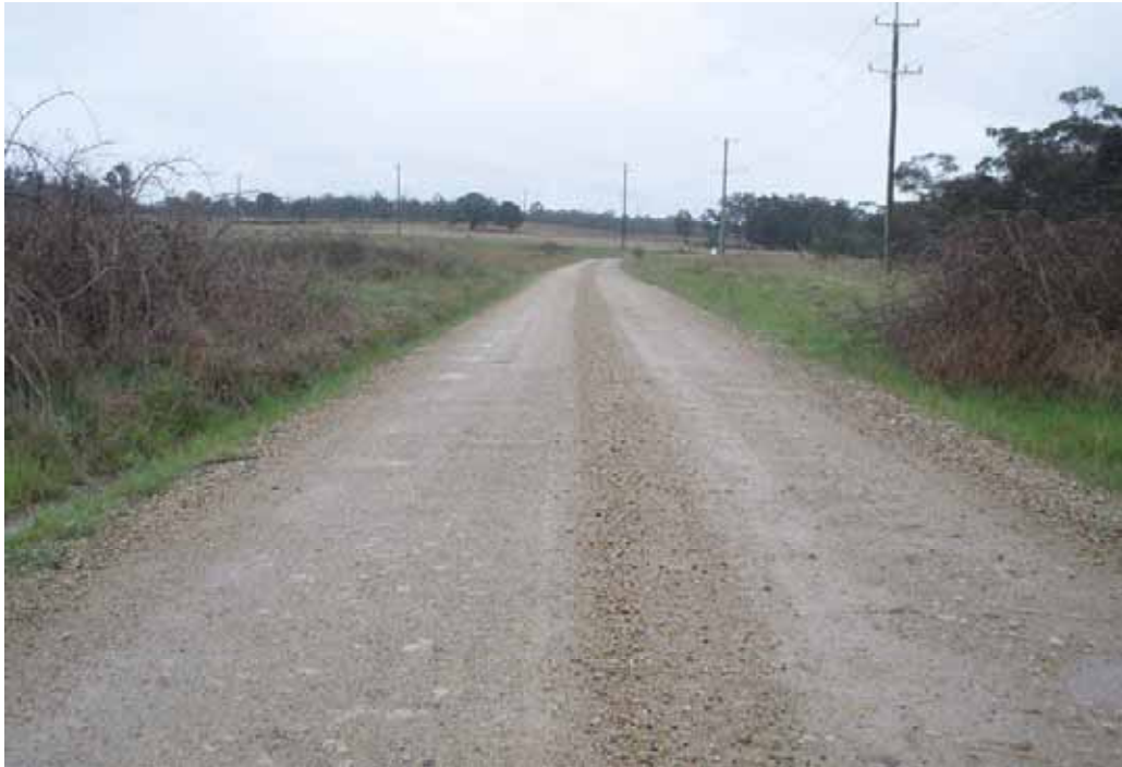
Photo 115 – Stoney Creek Rd (unsealed). Small potholes, uneven surface and corrugations.
