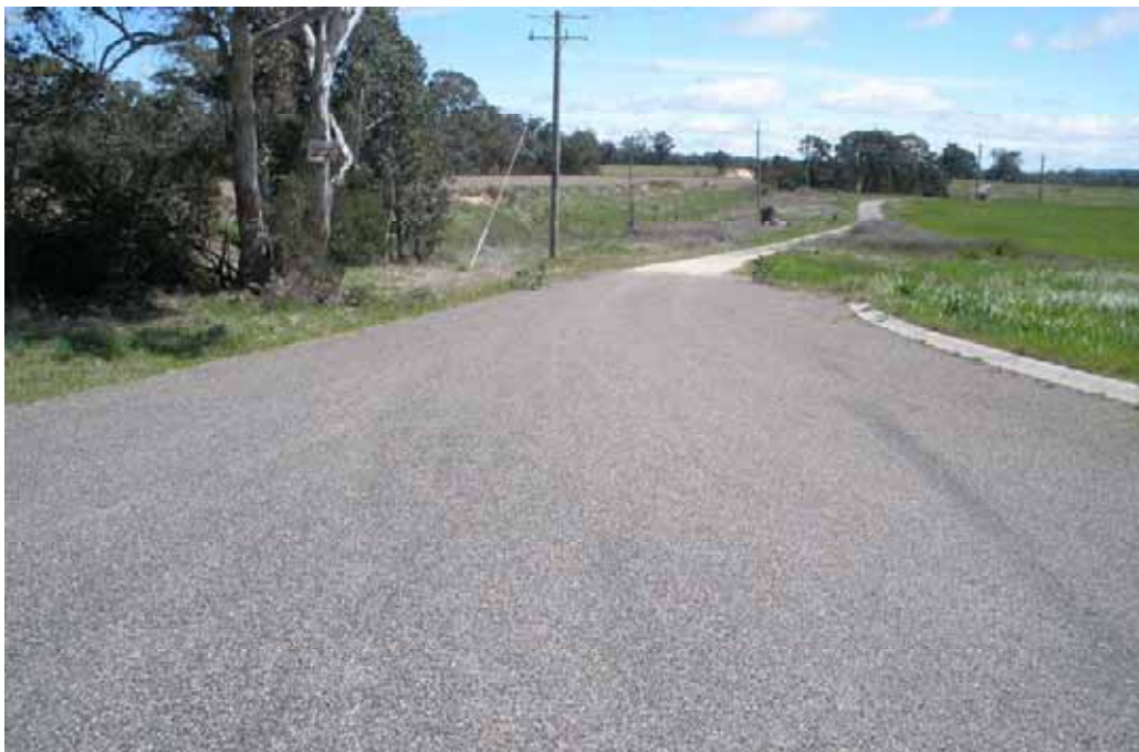
Photo 100 – End of spray seal/start of unsealed road Stoney Creek Rd. Excessive surface aggregate.
