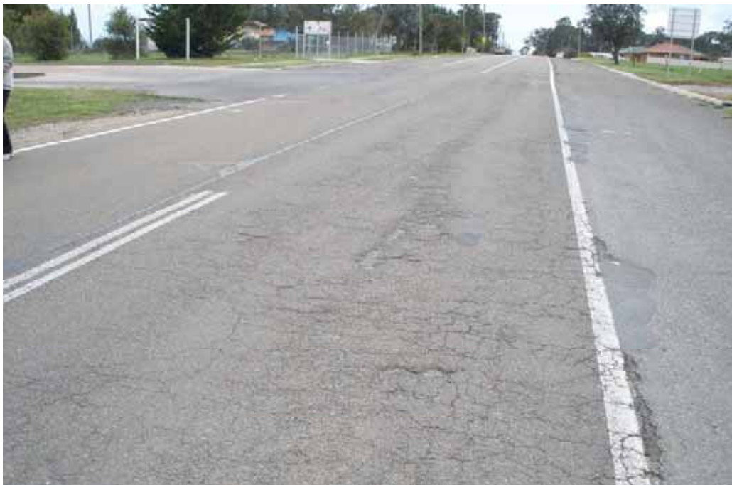
Photo 10 – Near exit driveway for Truck Stop 31. Extensive cracking and some old patching.
