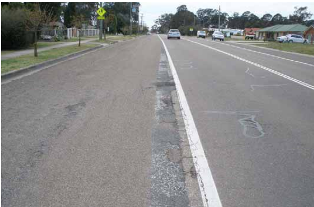
Photo 16 – George Street, opposite vacant blocks. Edge failure, numerous cracking some sealed with bitumen emulsion.
