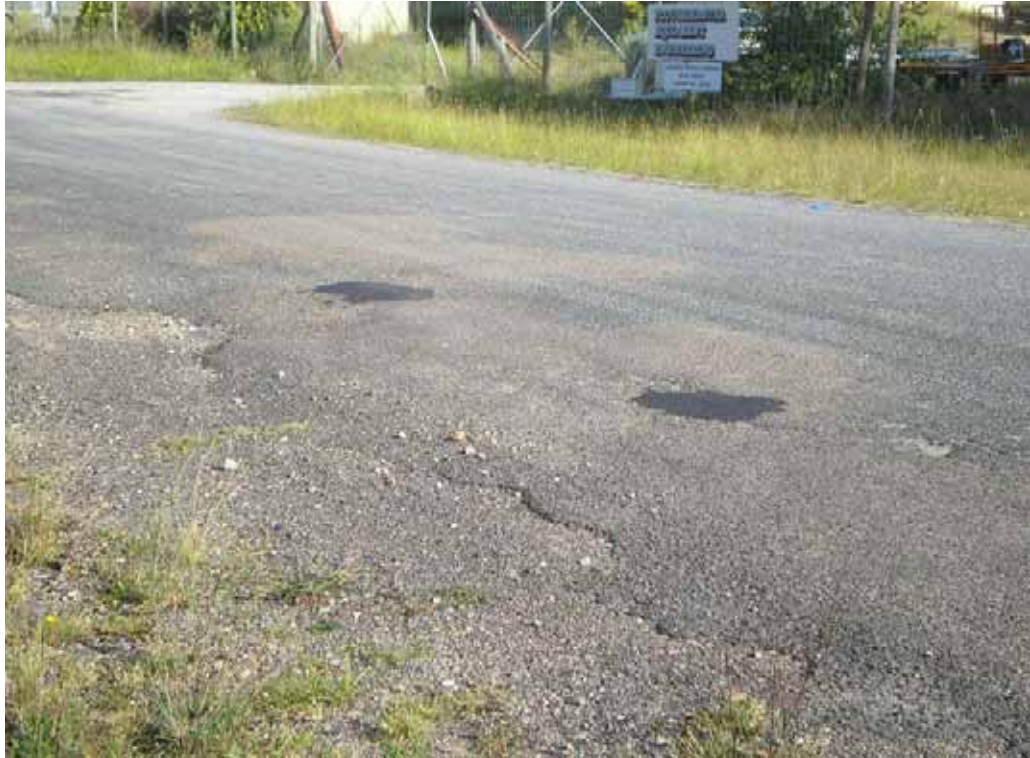
PHOTO 47: Entrance to Ploughmaster Engineering, shoulder failures and repairs
