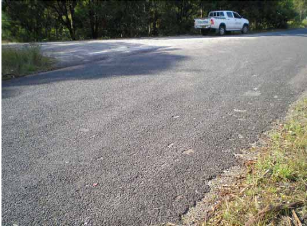
PHOTO 69: Back entrance to BP Service Centre, loss of seal, slight rutting, edge failure
