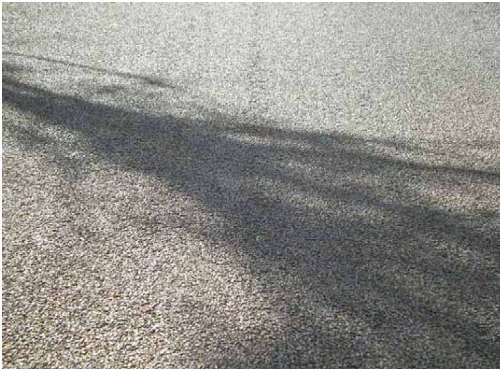
PHOTO 92: Stripped aggregate centreline
