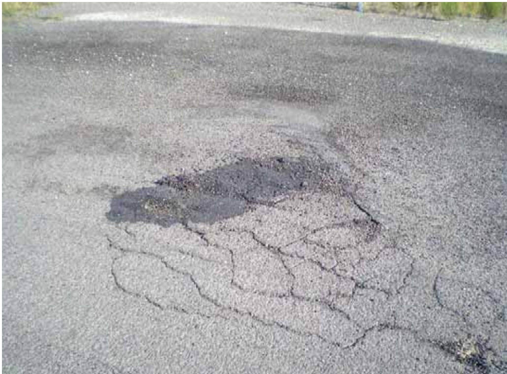
PHOTO 58: Loose gravel, cracking in asphalt, failed pothole repair
