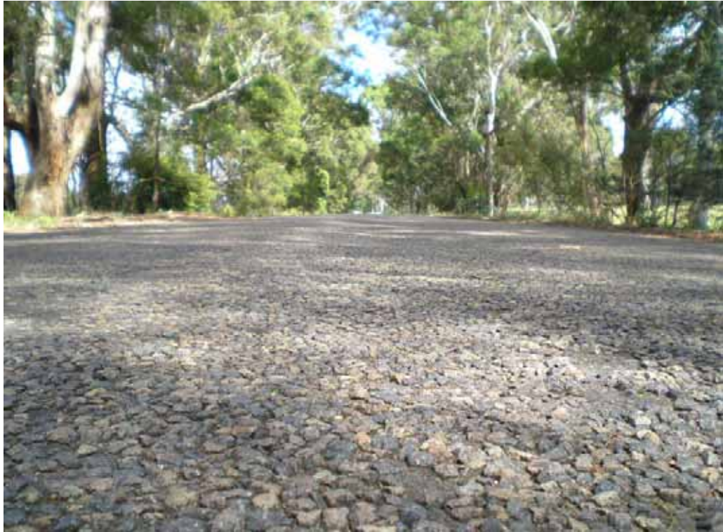
PHOTO 99: Stripped aggregate, settlement/rutting
