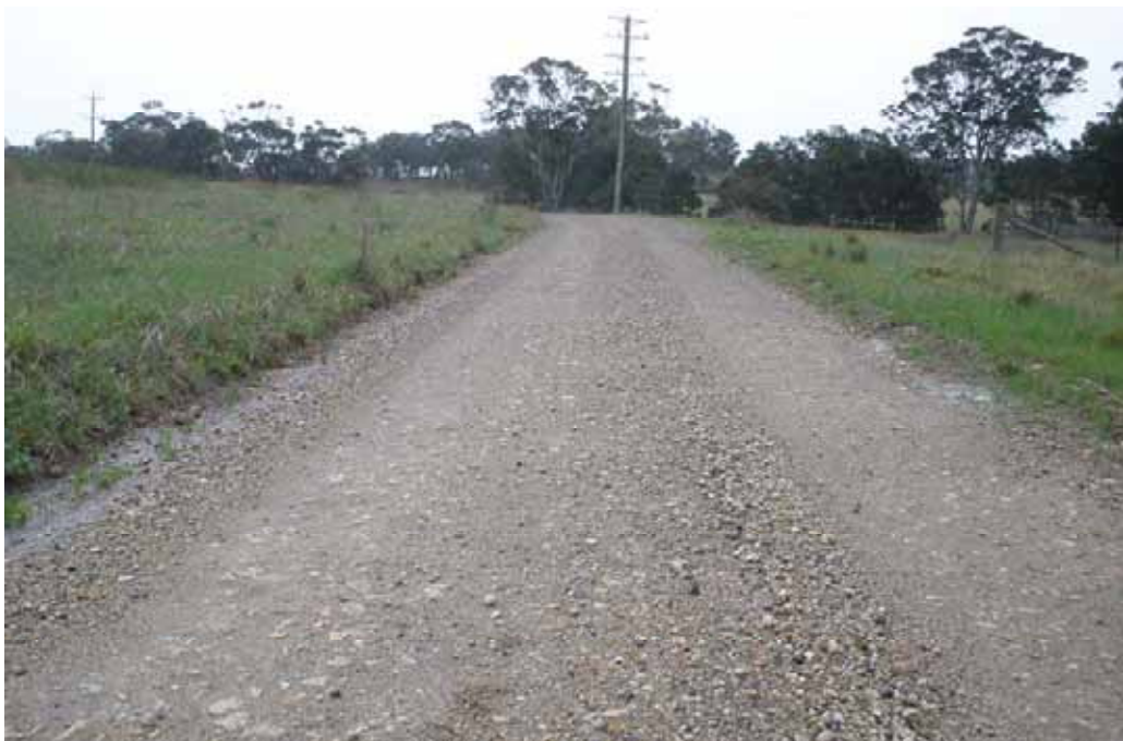
Photo 112 – Stoney Creek Rd (unsealed). Uneven surface.
