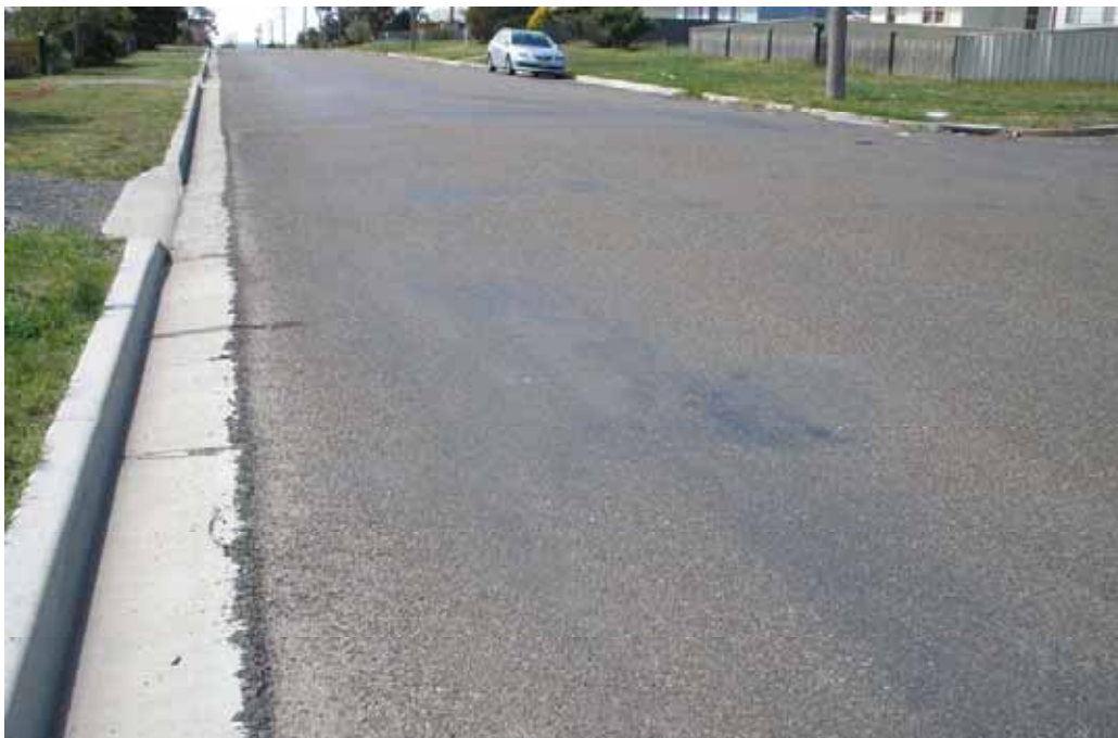
Photo 66 – Near Brayton Rd/Wollondilly St intersection. Bitumen bleeding, start of small potholes.
