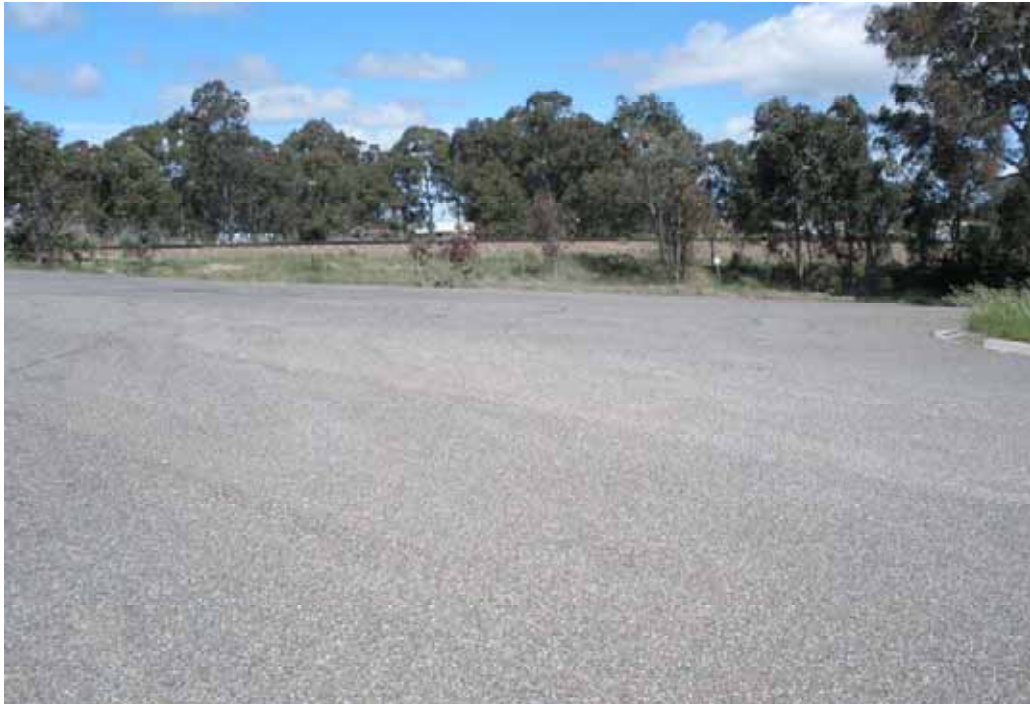
Photo 99 – 90 bend in Stoney Creek Rd. Aggregate loss and uneven surface.
