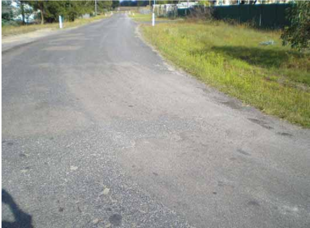
PHOTO 41: Cracking in asphalt, repaired sections, loss of seal
