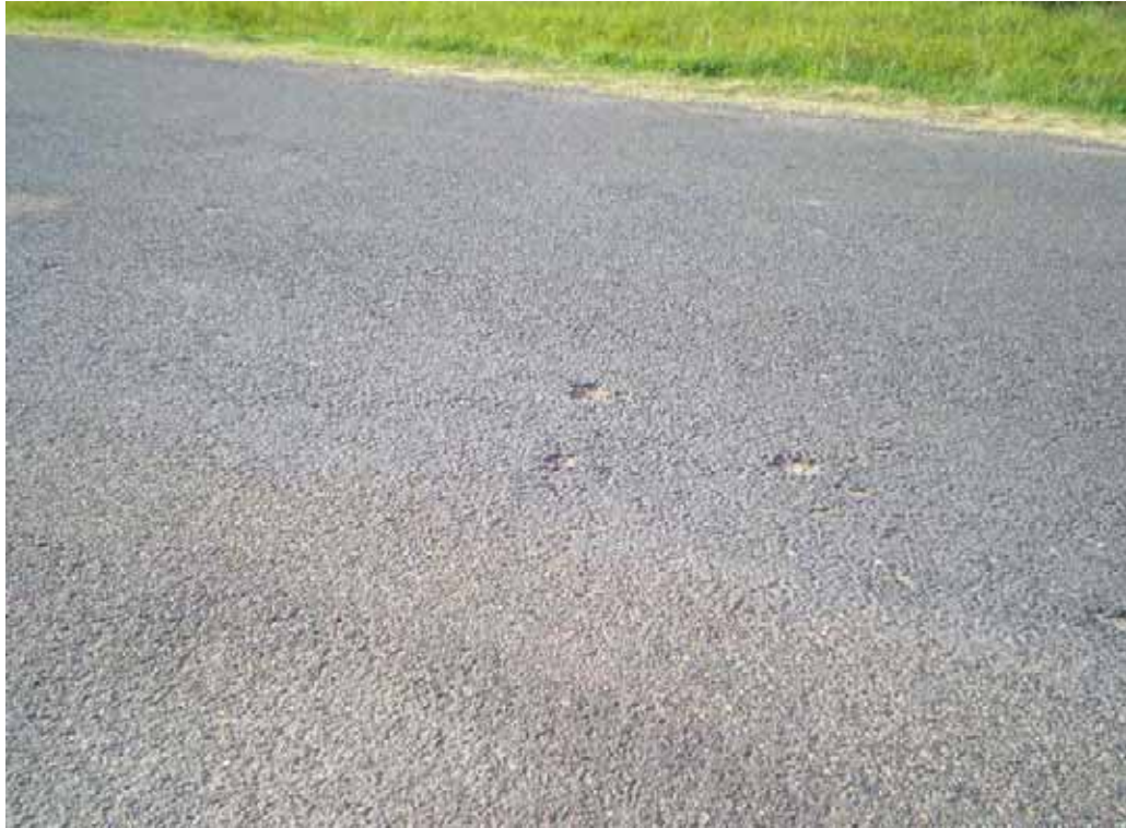
PHOTO 21: Loss of seal, slight rutting
