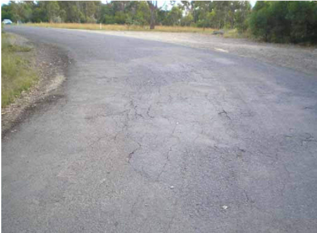
PHOTO 88: Extensive cracking in asphalt
