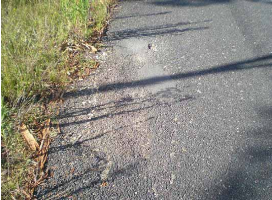
PHOTO 67: Edge failures, repaired potholes
