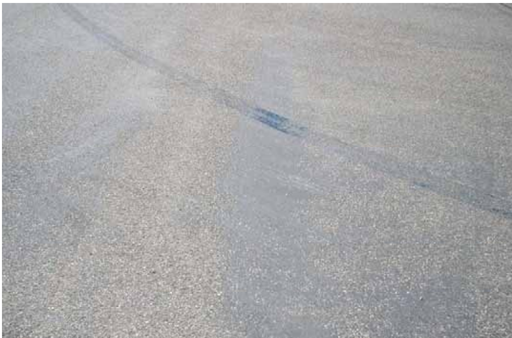
Photo 96 – Intersection of Stoney Creek Rd & Jilba Ave. Bitumen bleeding.
