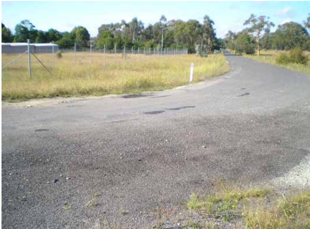
PHOTO 63: Shoulder/pothole repairs, loose gravel at pavement edge
