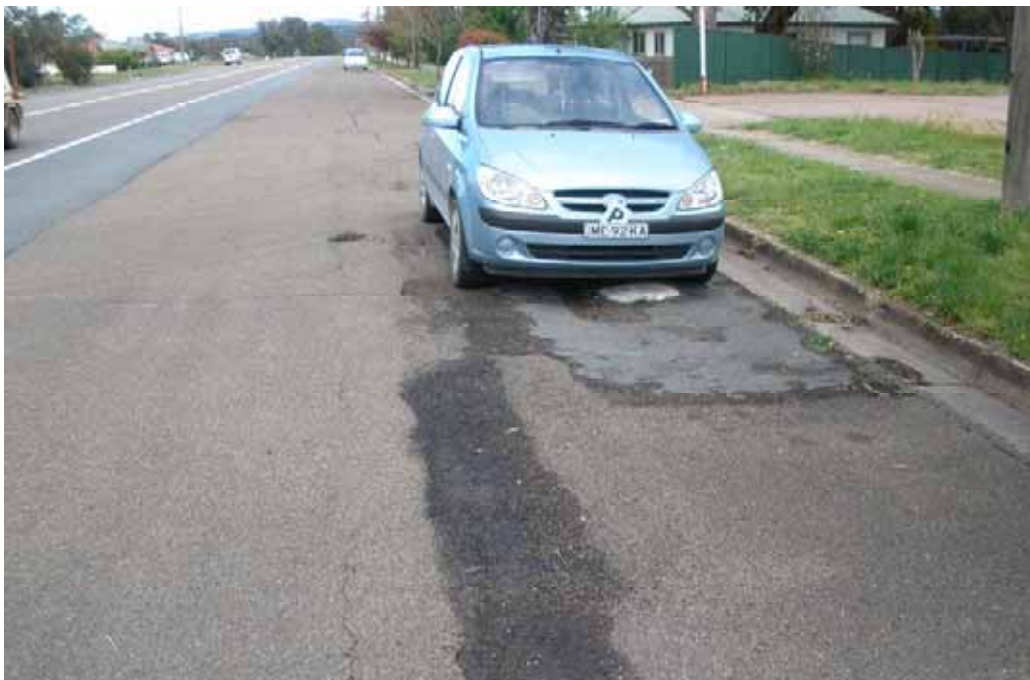
Photo 24 – Opposite Marulan Auto Port. Previously patched failed areas in shoulder.
