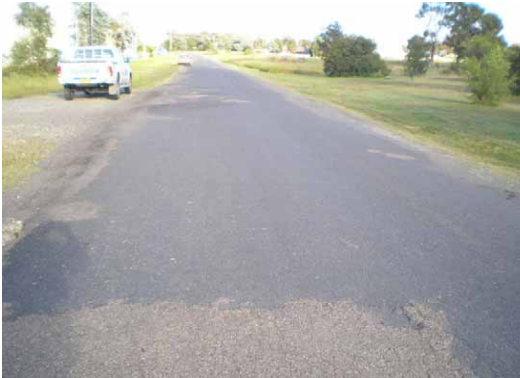
PHOTO 10: Change in seal, some repaired sections
