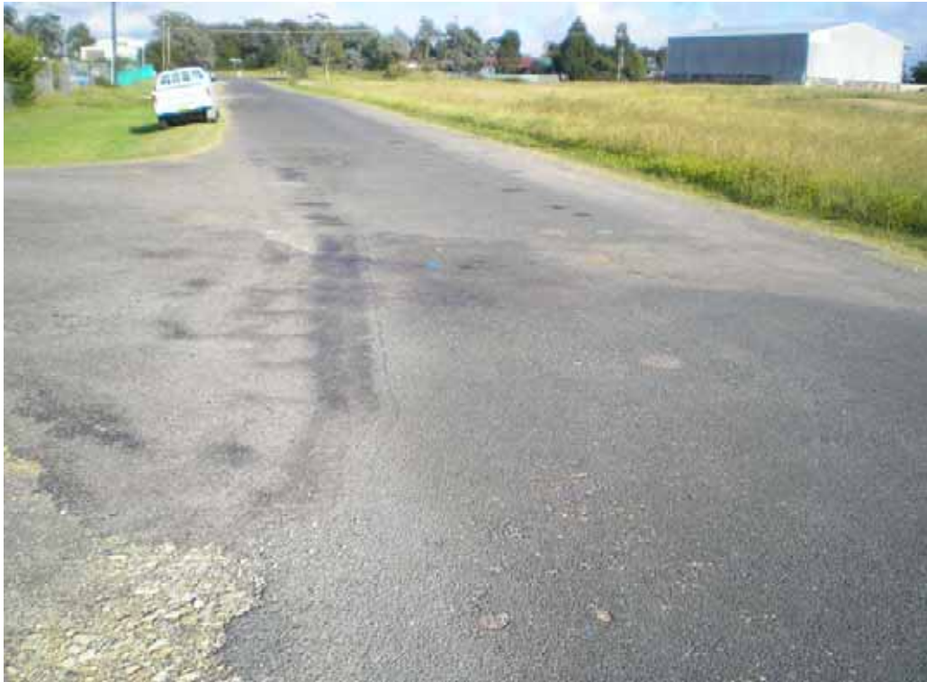
PHOTO 14: Entry to Marulan Rural Services, signs of rutting, repaired potholes and loss of seal
