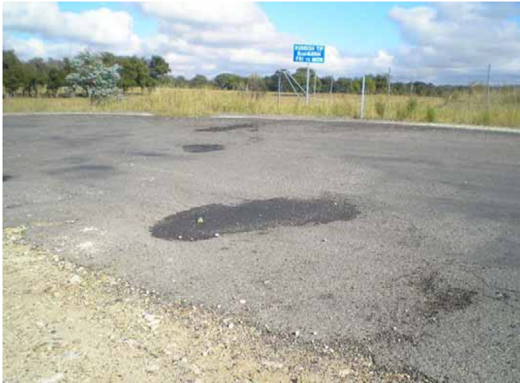
PHOTO 57: Extensive failures at corner
