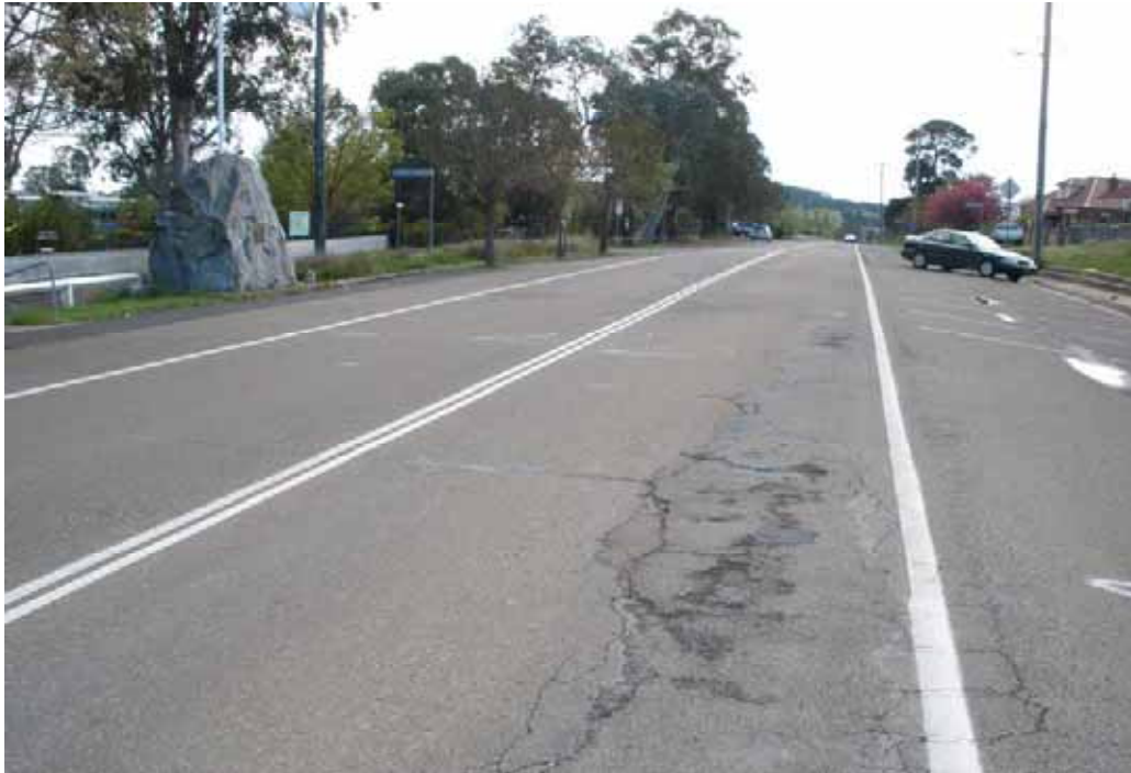
Photo 41 – Opposite No 83 George St. Extensive pavement failure some old patches.
