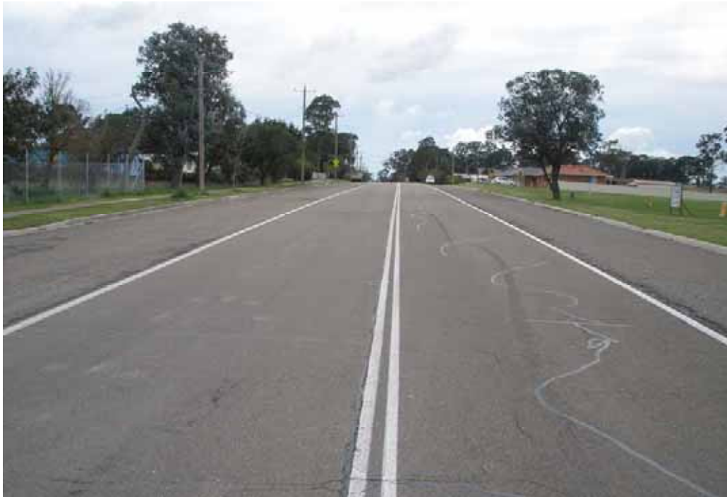
Photo 13 – George Street, opposite vacant blocks. Numerous cracking some sealed with bitumen emulsion.
