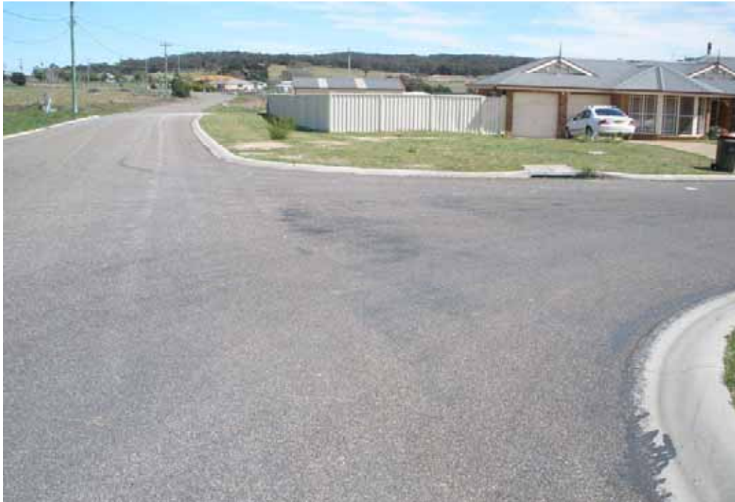
Photo 81 – Patrick Pl/Maclura Dr intersection. Bitumen bleeding.
