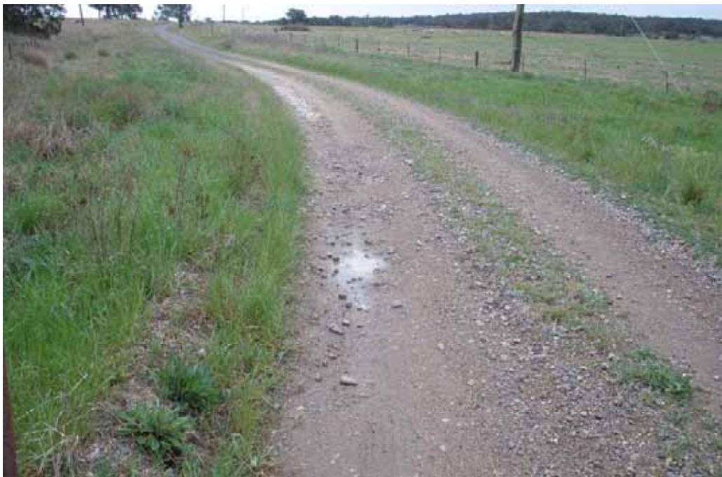
Photo 104 – Stoney Creek Rd (unsealed). Series of potholes southern side.
