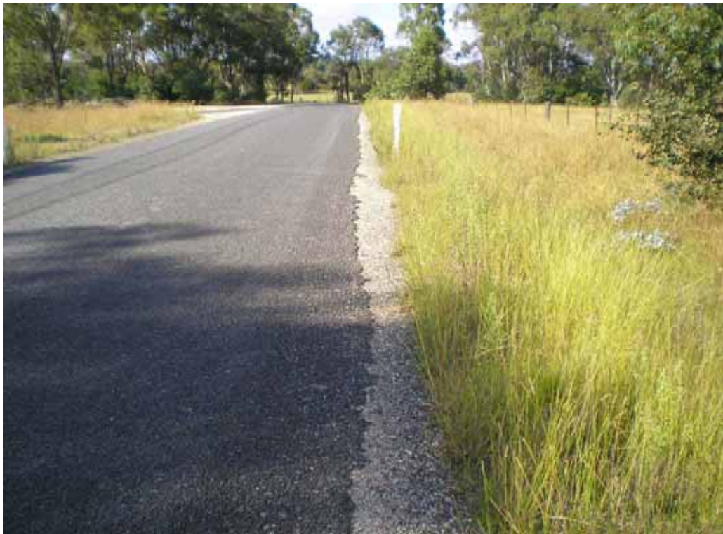
PHOTO 76: Pavement edge failure
