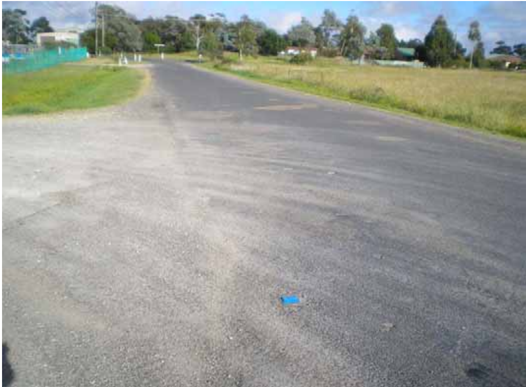
PHOTO 18: Repaired sections, loss of seal
