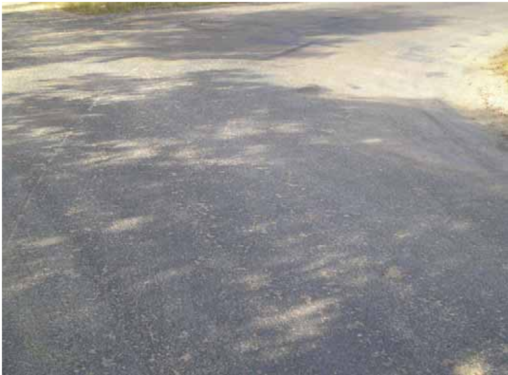
PHOTO 36: Loss of seal
