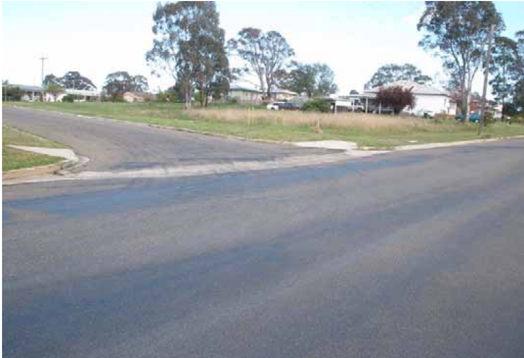
Photo 61 – Brayton Rd/Station St intersection. Bitumen bleeding and slight rutting.
