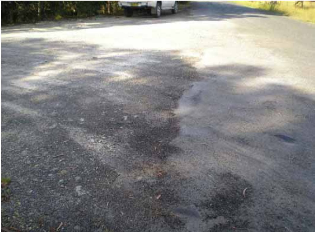
PHOTO 72: Shoving/settlement of shoulder/pavement edge, loose gravel
