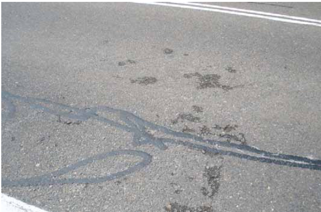
Photo 26 – Opposite Brewer Centre. Aggregate loss and bitumen emulsion sealed cracks.
