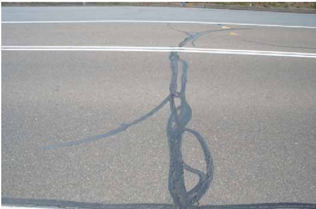
Photo 28 – Opposite church. Pavement cracking post application of bitumen emulsion.
