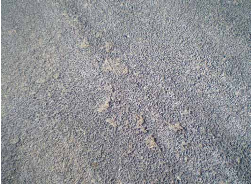
PHOTO 53: Loss of seal
