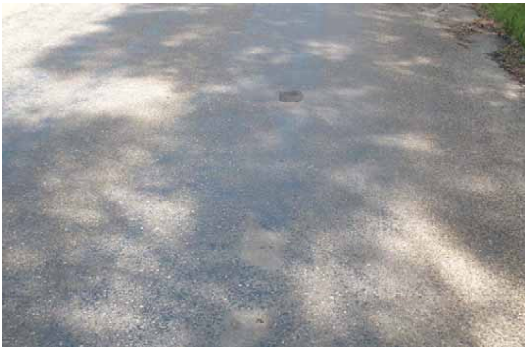
Photo 72 – Opposite tennis courts. Bitumen bleeding, small potholes and slight rutting.
