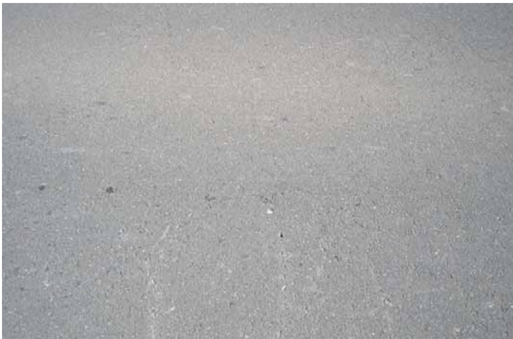
Photo 50 – Opposite police station. Start of cracking in newer pavement.
