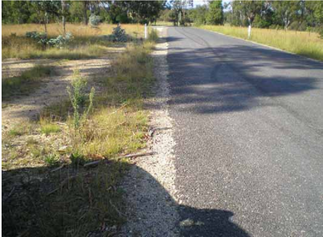
PHOTO 75: Pavement edge failure
