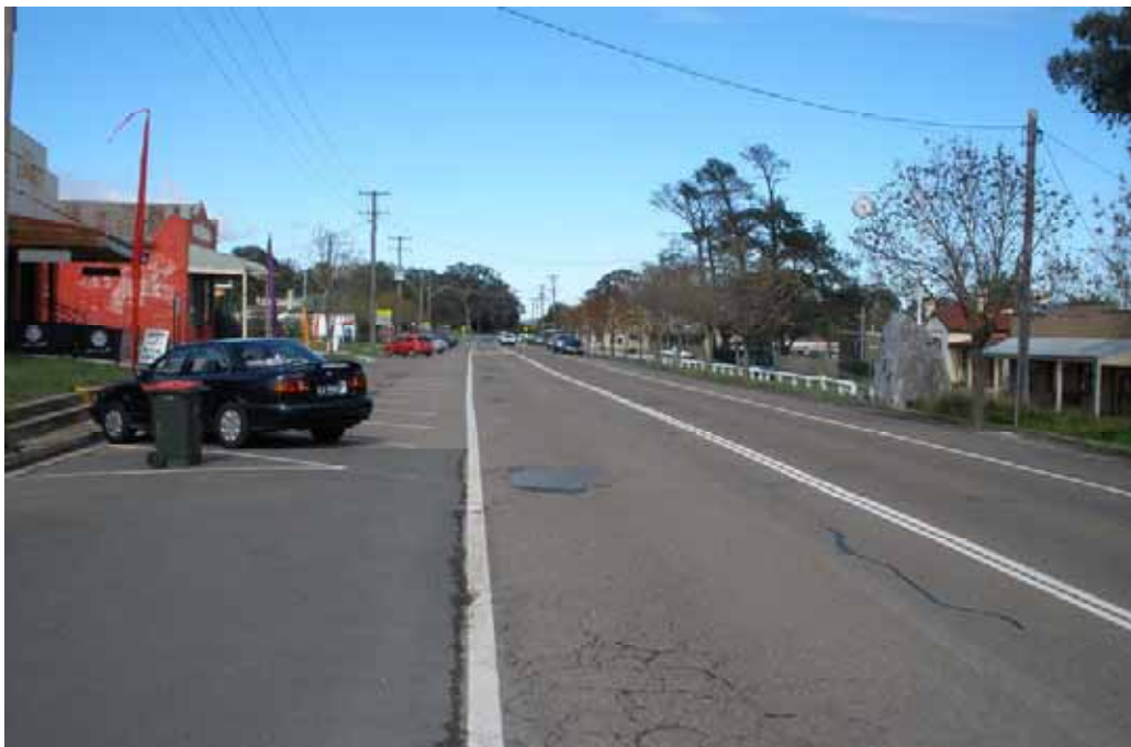
Photo 44 – Opposite park looking back on significantly failed section.
