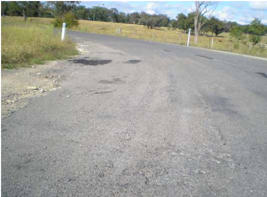
PHOTO 60: Repaired and failed sections/potholes, cracking in asphalt, shoulder failure
