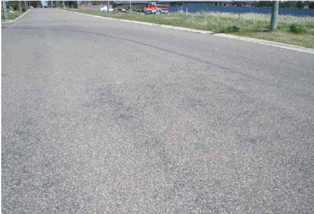
Photo 93 – Opposite No 17 Stoney Creek Rd. Bitumen bleeding.
