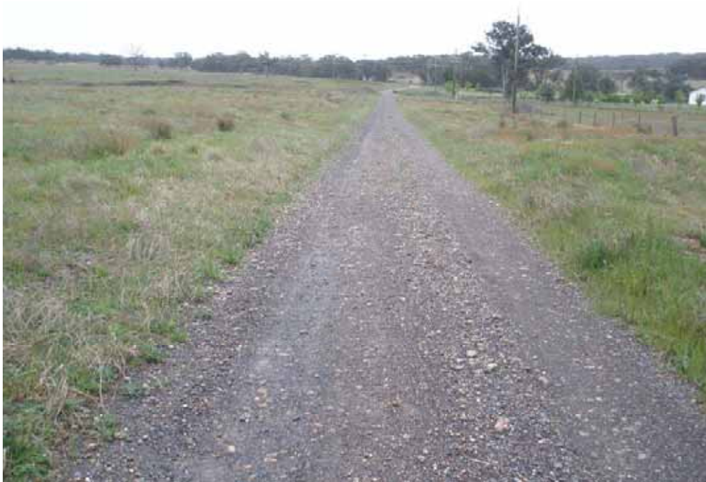
Photo 109 – Stoney Creek Rd (unsealed). Section of coarse gravel with depressioning along southern wheel path.
