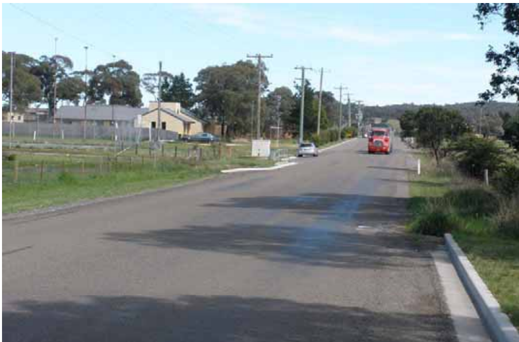
Photo 70 – Near tennis courts. Opposite No 39 Brayton Rd. Bitumen bleeding, start of small potholes and slight rutting.
