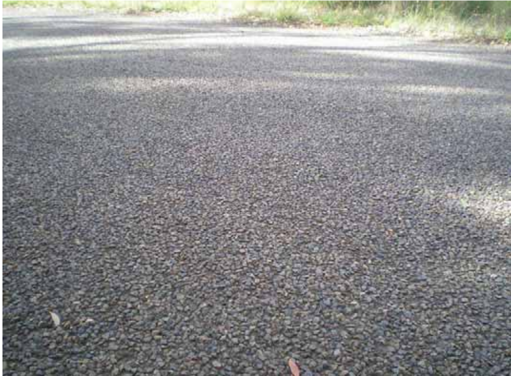
PHOTO 93: Stripped aggregate, slight rutting
