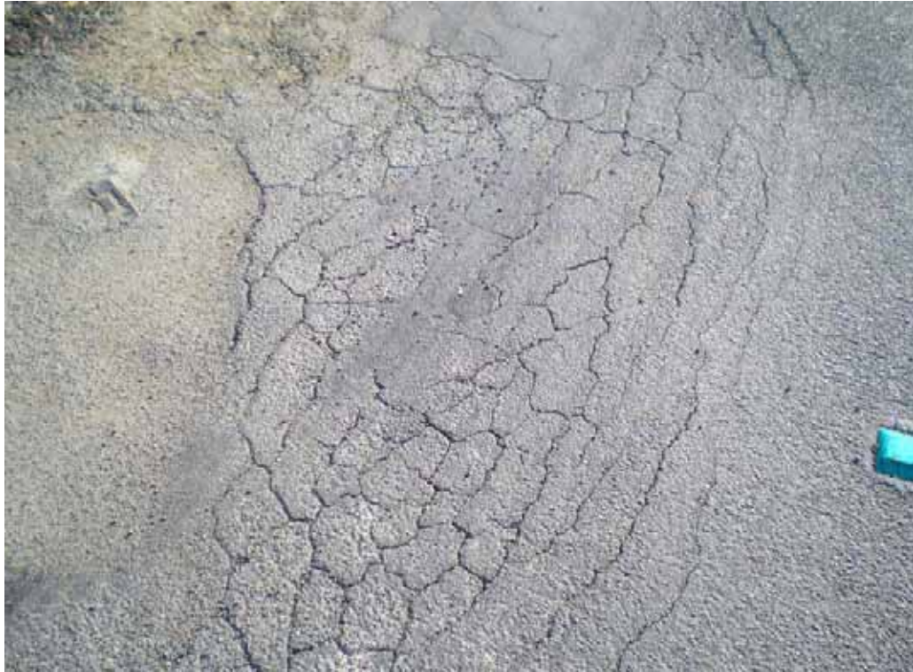
PHOTO 43: Cracking in asphalt, rutting
