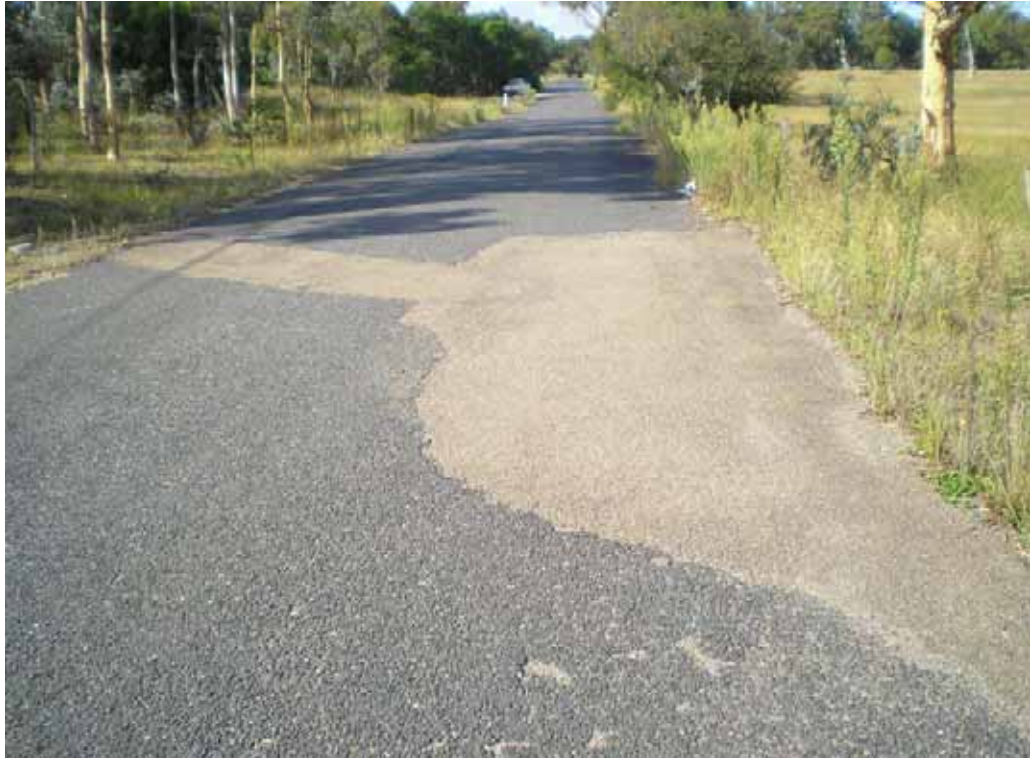
PHOTO 65: Repaired section, loss of seal/cracking
