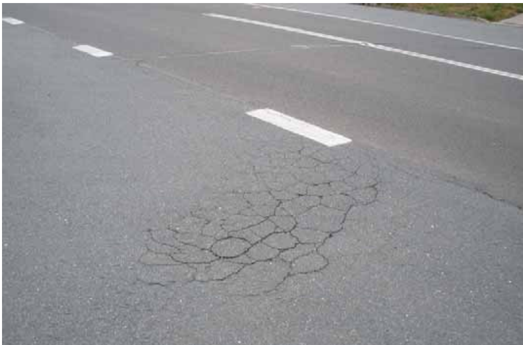
Photo 30 – Goulburn St at intersection with George St. Crocodile cracking.
