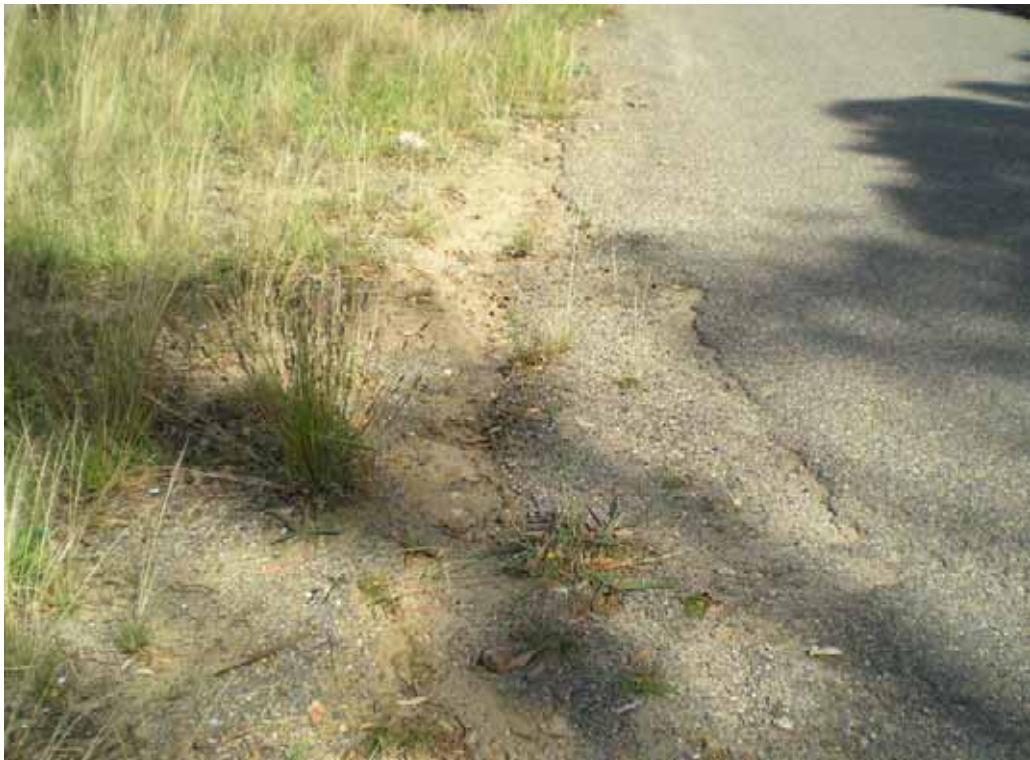
PHOTO 104: Failure at pavement edge, erosion
