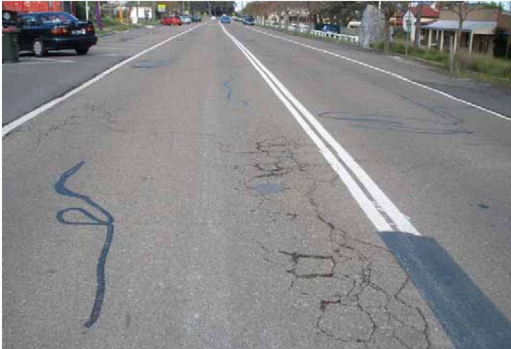
Photo 43 – Opposite park. Extensive pavement failure some old patches.
