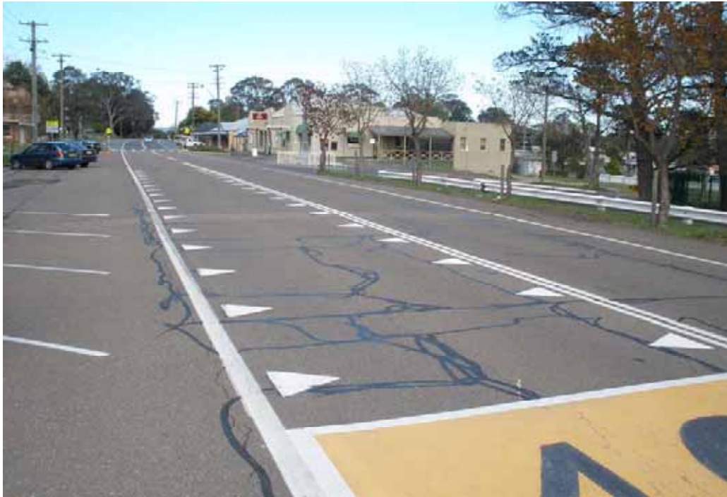
Photo 37 – Opposite butcher. Extensive cracking mainly sealed with bitumen emulsion some unsealed.
