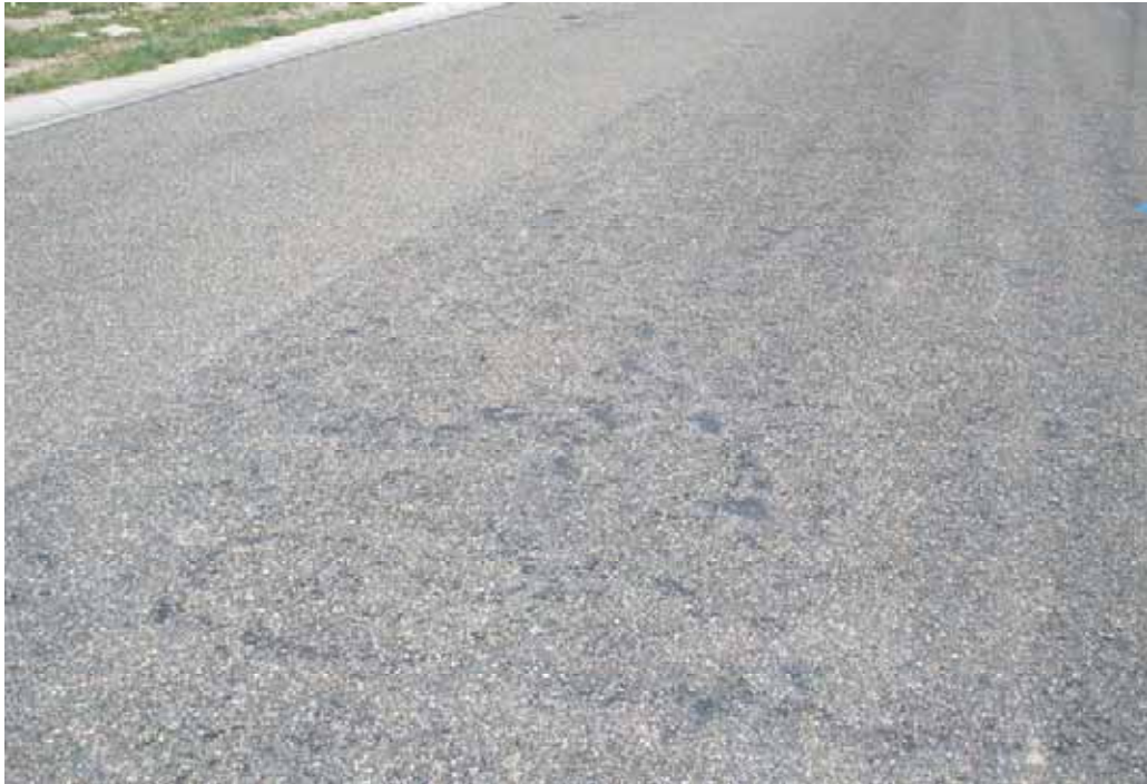
Photo 79 – Opposite No 3 Maclura Dr. Bitumen bleeding.
