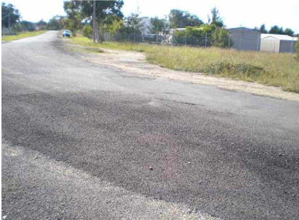
PHOTO 61: Settlement of repaired section
