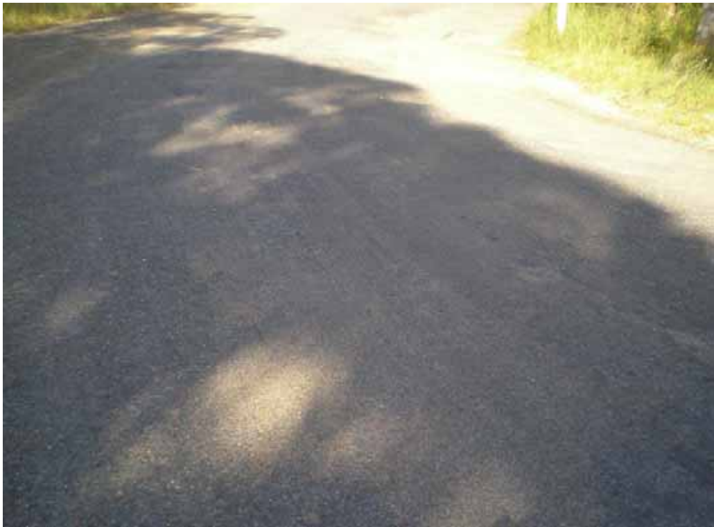
PHOTO 82: Repaired sections/potholes, loss of seal, settlement/rutting
