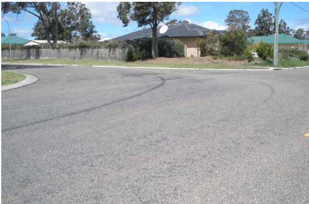
Photo 94 – Intersection of Stoney Creek Rd & Jilba Ave. Bitumen bleeding.
