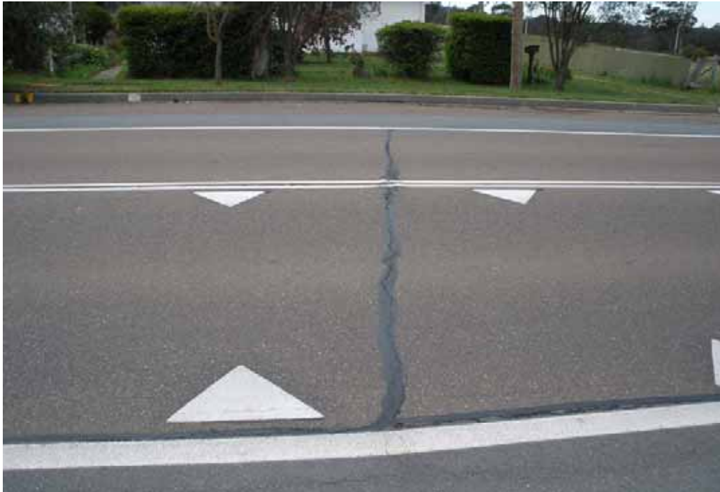
Photo 21 – Opposite No 36 George St. Bitumen emulsion sealed transverse crack.
