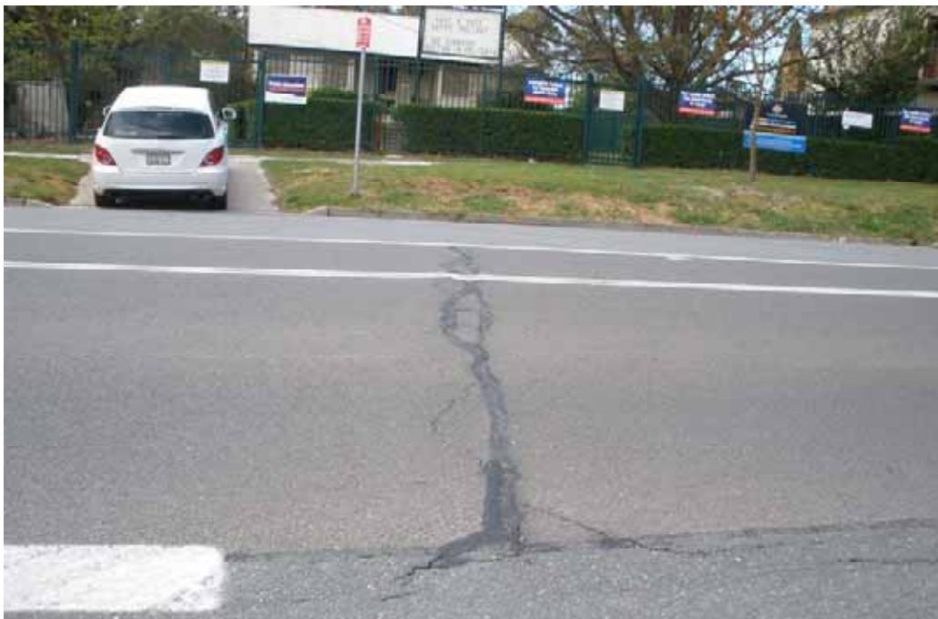
Photo 32 – Opposite school. Pavement cracking post application of bitumen emulsion. Edges of cracking rising.
