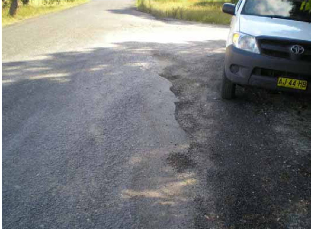
PHOTO 73: Settlement of shoulder repair, loose gravel
