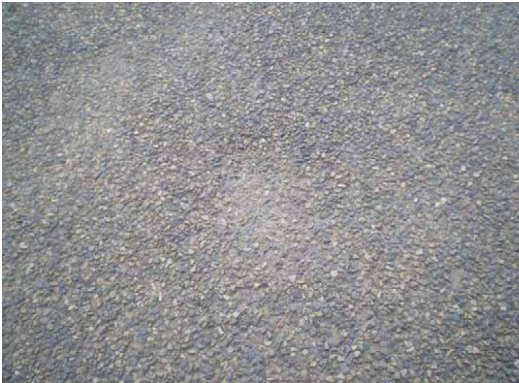
PHOTO 102: Depressions in pavement
