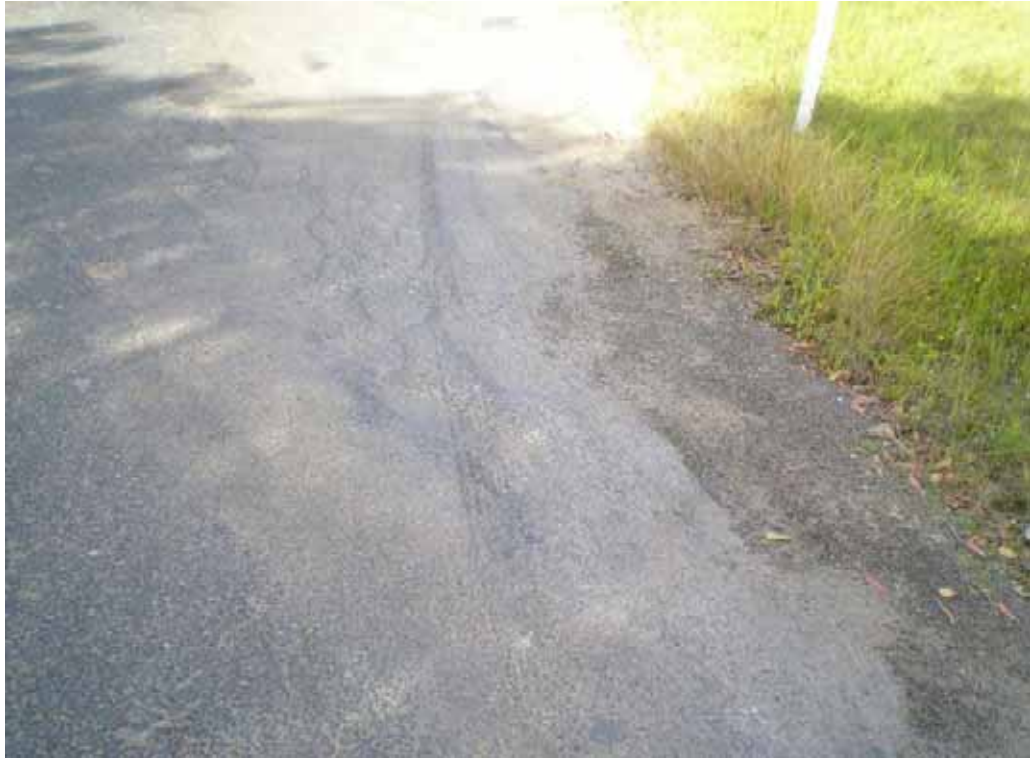
PHOTO 37: Settlement, cracking/rutting in asphalt at pavement edge
