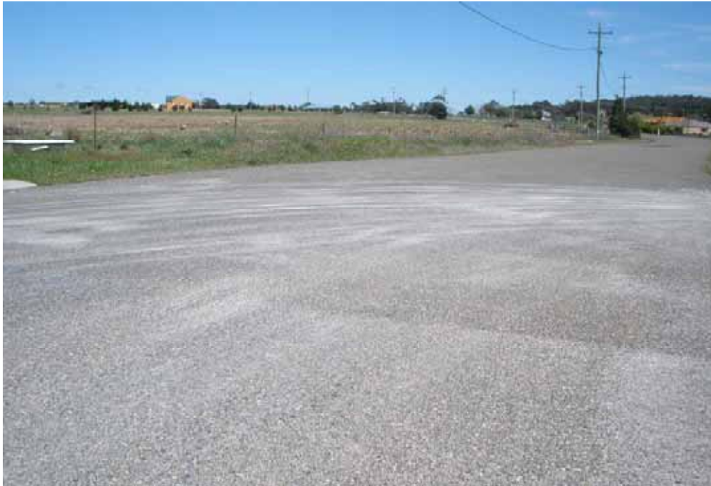
Photo 83 – Entrance to Lot 9 Maclura Dr. Uneven surface some bitumen bleeding.
