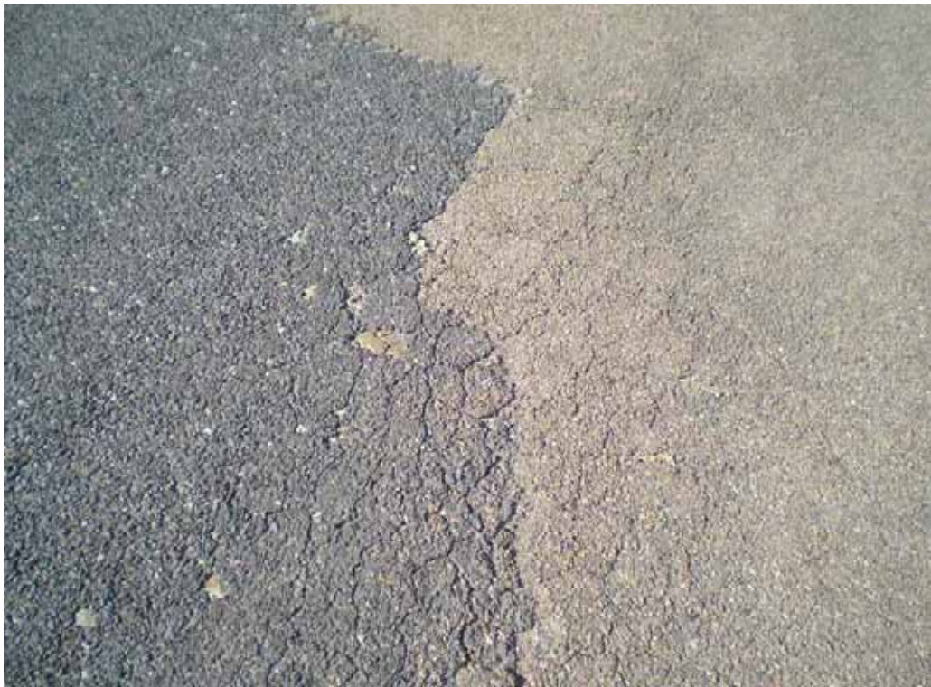
PHOTO 66: Cracking in asphalt at edge of repaired section
