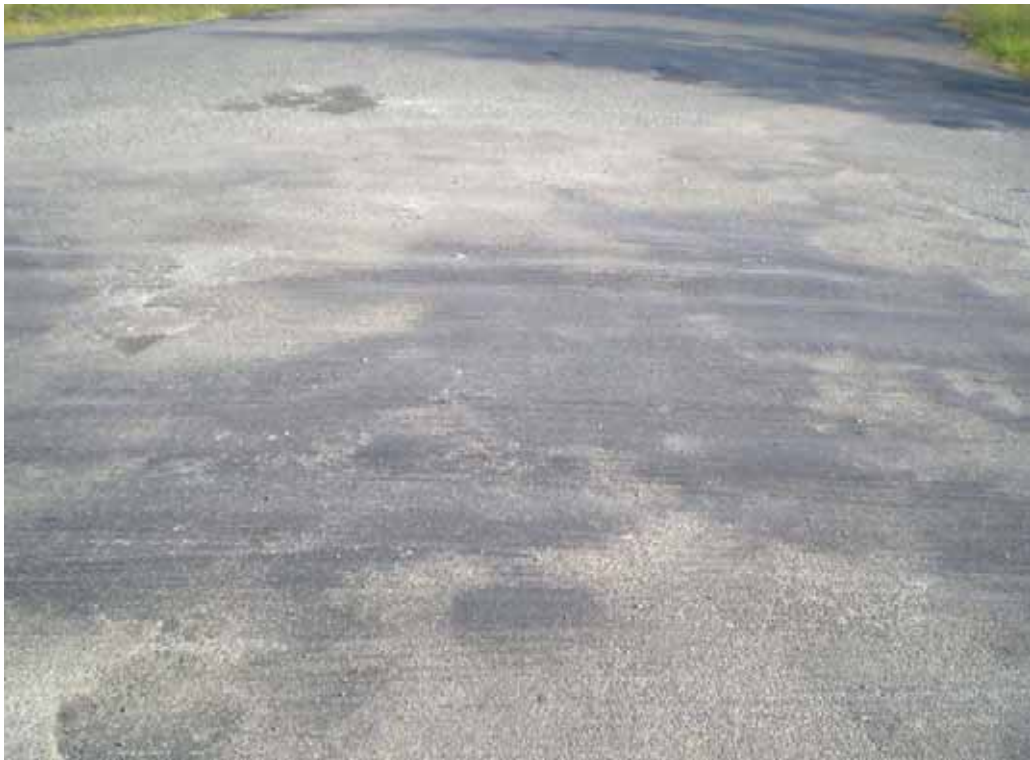
PHOTO 26: Bitumen bleeding, shoving/rutting in asphalt, repaired potholes
