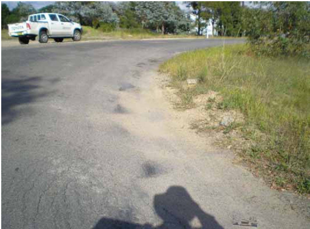
PHOTO 40: Failure at pavement edge
