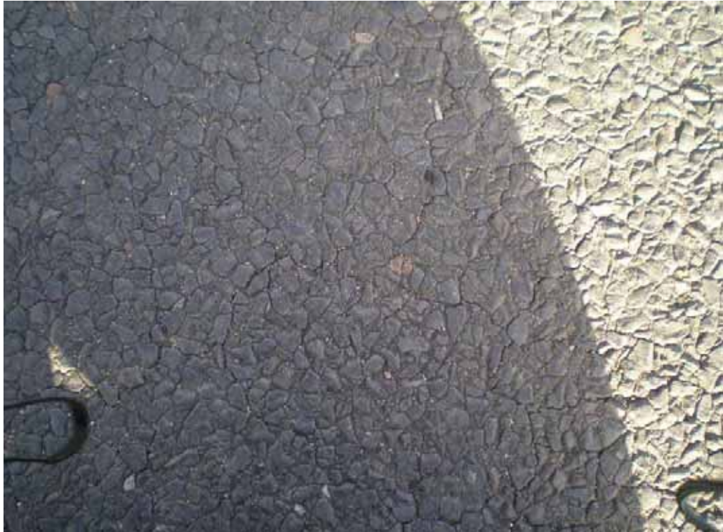
PHOTO 17: Start of cracking in asphalt
