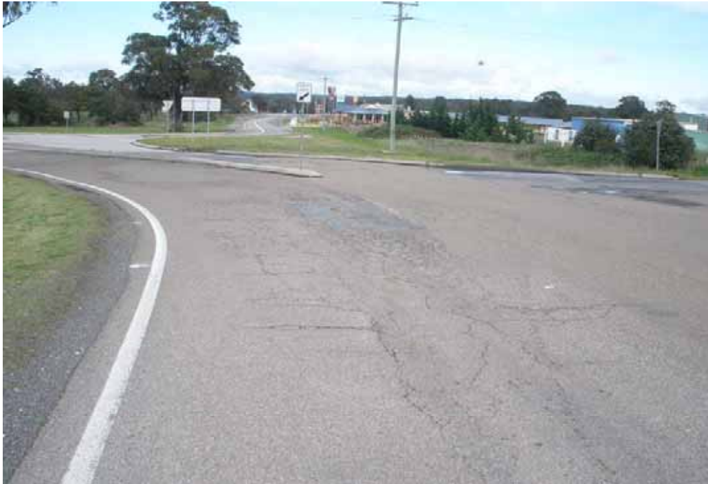
Photo 1 – Portland Ave/George St intersection. Extensive cracking, minor rutting and previous repairs.
