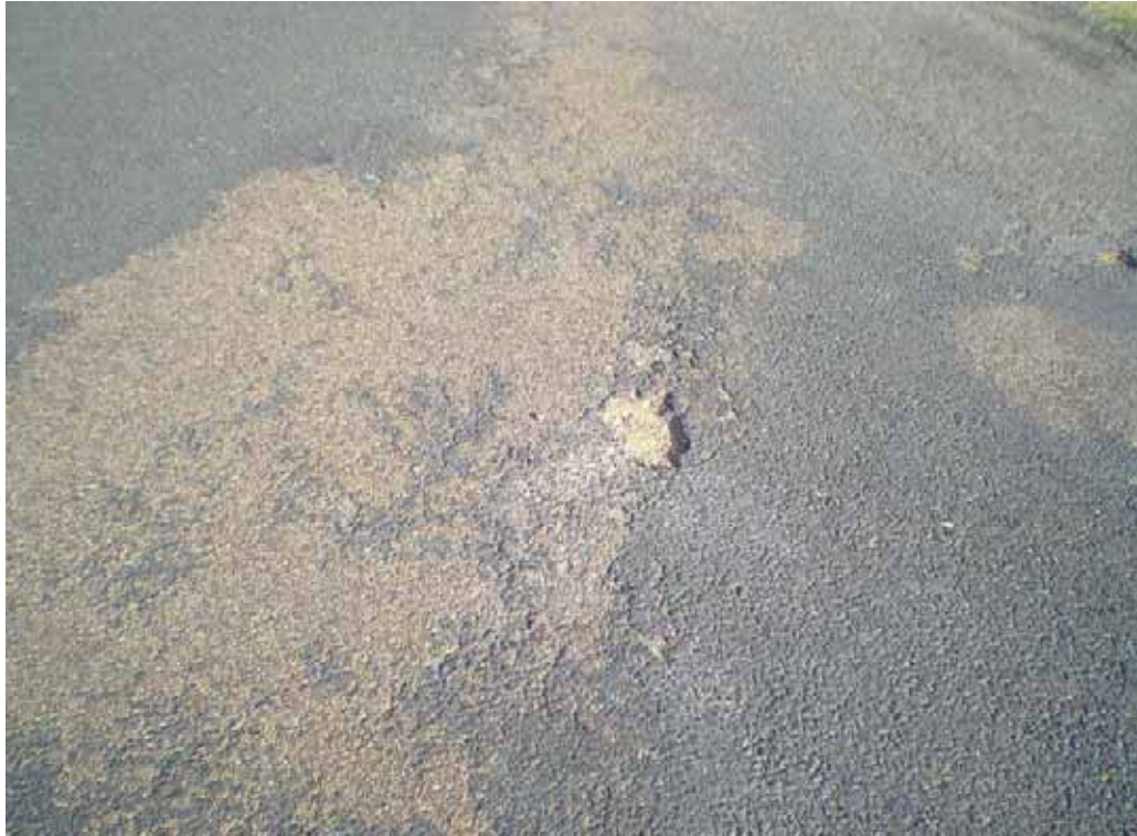
PHOTO 19: Start of pothole, some repaired sections
