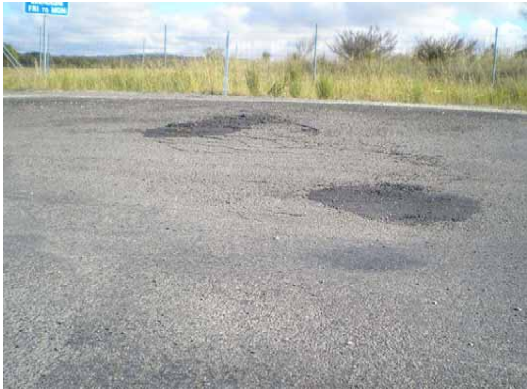
PHOTO 59: Repaired and failed sections, some rutting/shoving
