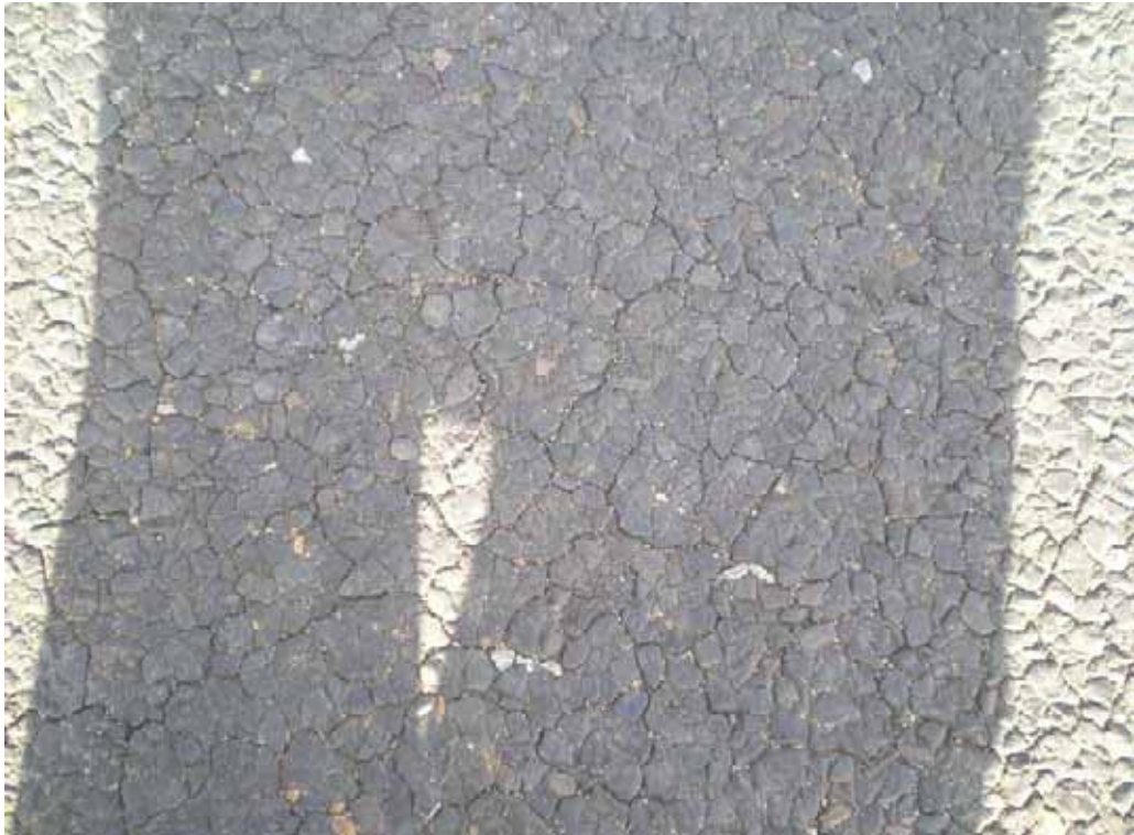
PHOTO 20: Start of cracking in asphalt
