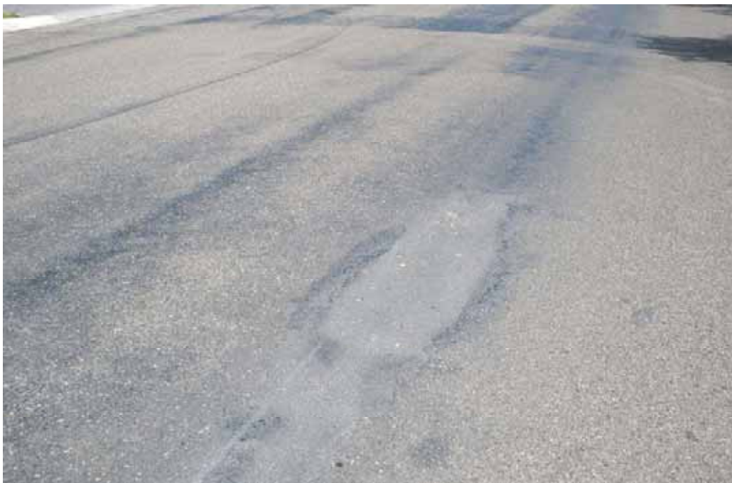
Photo 74 – Opposite tennis courts. Bitumen bleeding, small potholes and slight rutting.
