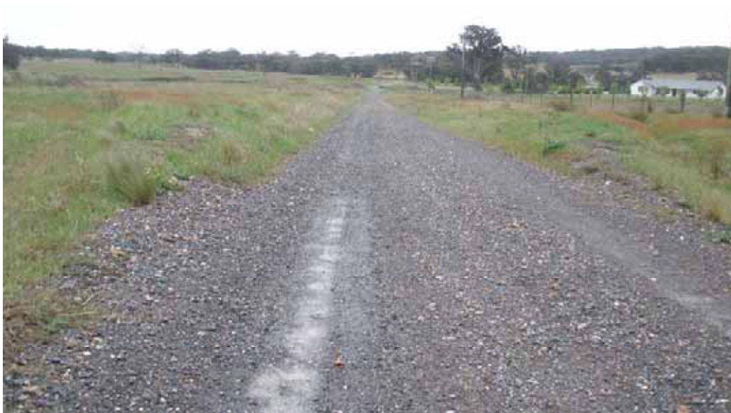
Photo 108 – Stoney Creek Rd (unsealed). Depressioning along southern wheel path.
