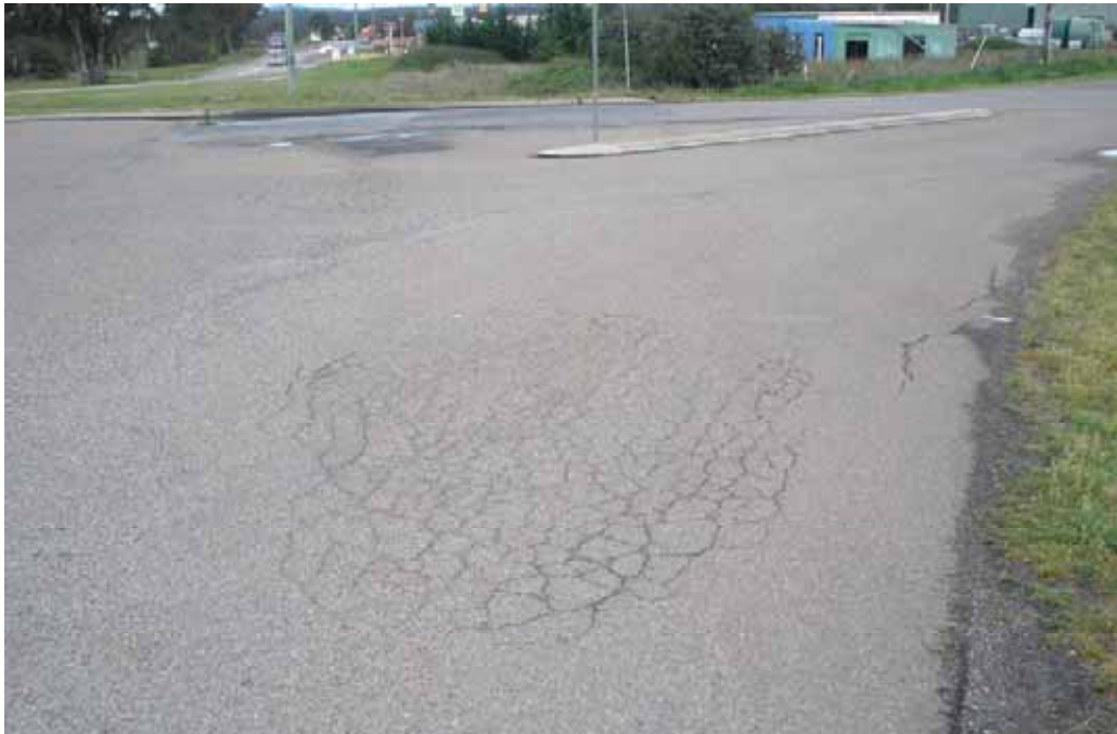
Photo 4 – Portland Ave/George St intersection. Extensive cracking, minor rutting and previous repairs.
