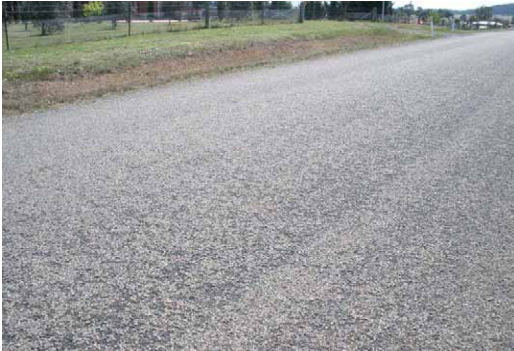
Photo 87 – Opposite Lot 18 Maclura Dr. Aggregate loss.
