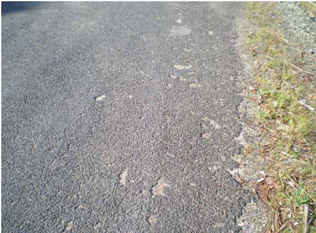
PHOTO 70: Loss of seal, edge failures, repaired pothole
