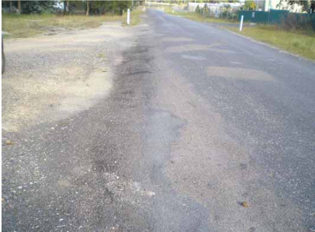
PHOTO 45: Repaired sections and shoulder, some cracking at shoulder edge
