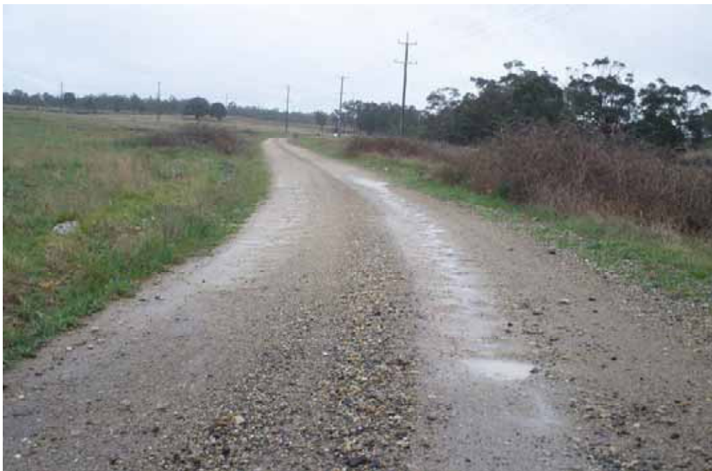
Photo 114 – Stoney Creek Rd (unsealed). Potholes and uneven surface.
