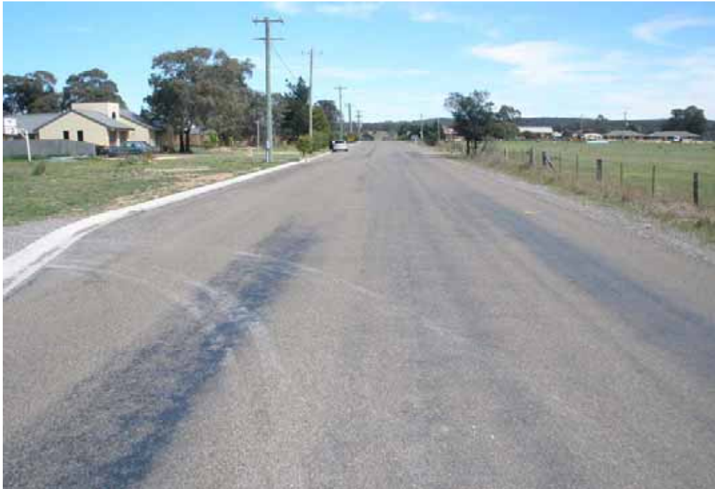
Photo 71 – Opposite tennis courts. Bitumen bleeding minor rutting.
