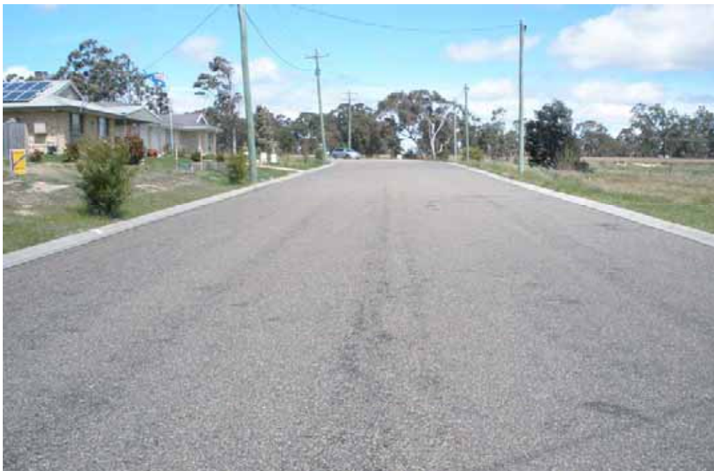
Photo 98 – Opposite No 15 Stoney Creek Rd. Bitumen bleeding, slight rutting and aggregate loss.
