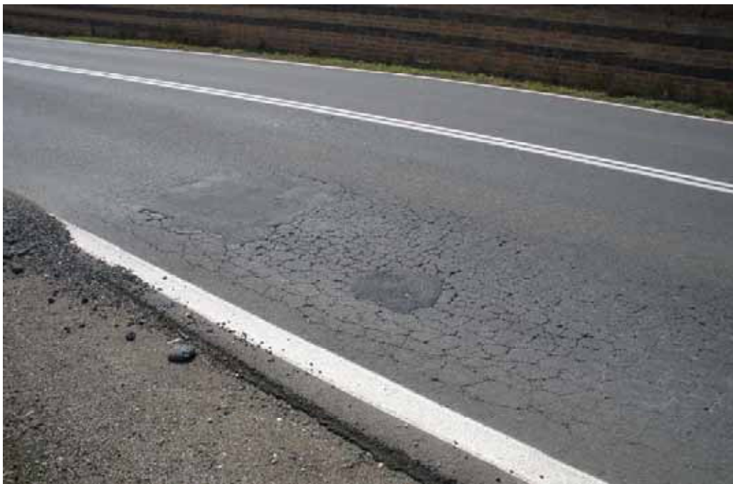
Photo 52 – Railway Bridge. Crocodile cracking with some patched areas and rutting.
