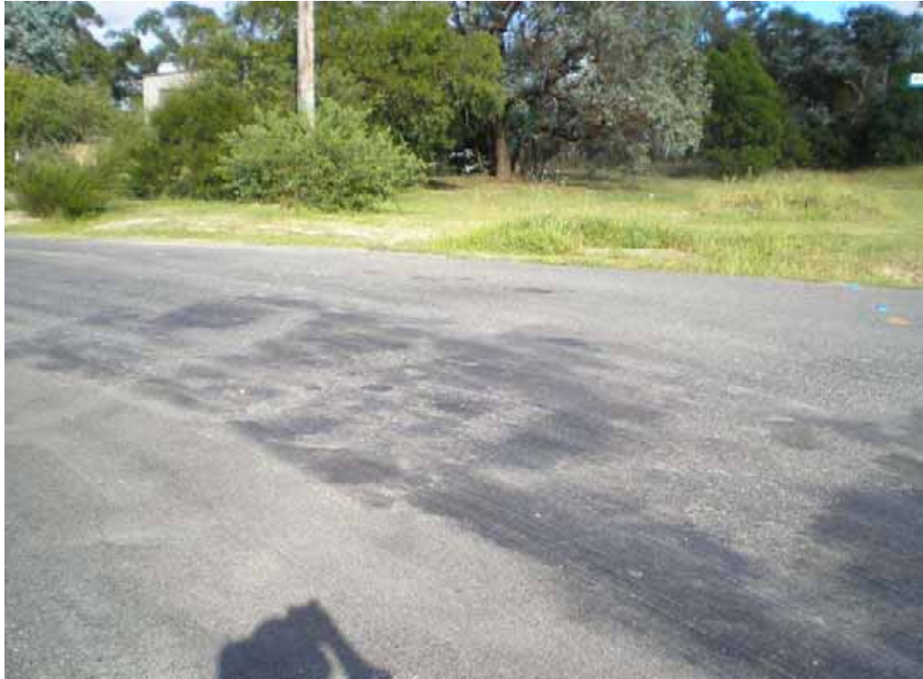
PHOTO 27: Bitumen bleeding, shoving/rutting in asphalt, repaired potholes
