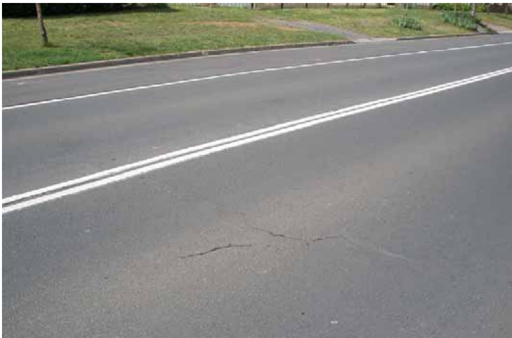
Photo 48 – Opposite Uniting Church. Cracking in section of newer pavement.
