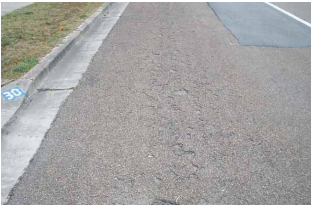
Photo 18 – Opposite No 30 George St. Wearing course loss in shoulder.
