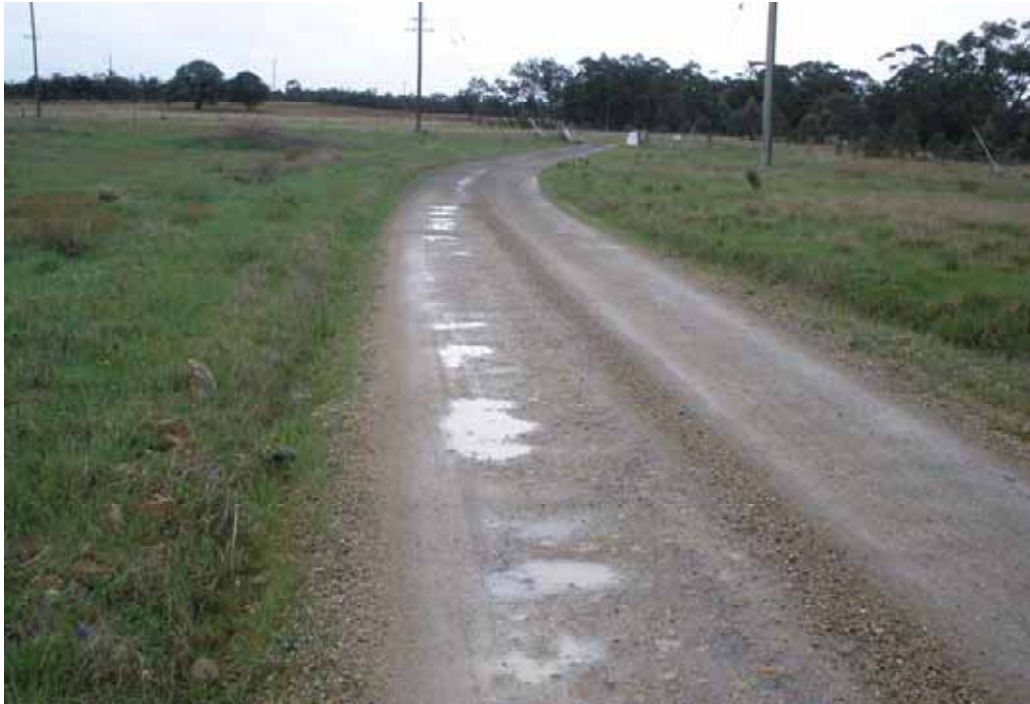
Photo 117 – Stoney Creek Rd (unsealed). Small potholes, uneven surface and corrugations.
