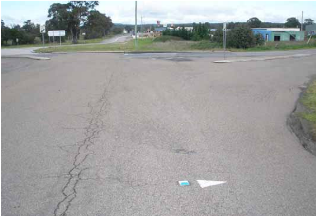
Photo 3 – Portland Ave/George St intersection. Extensive cracking, minor rutting and previous repairs.
