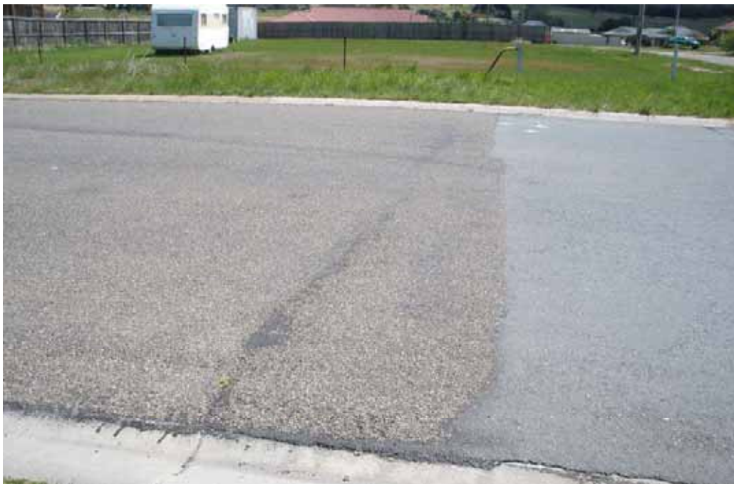
Photo 88 – Intersection of Brayton Rd & Stoney Creek Rd. Bitumen bleeding and uneven surface.
