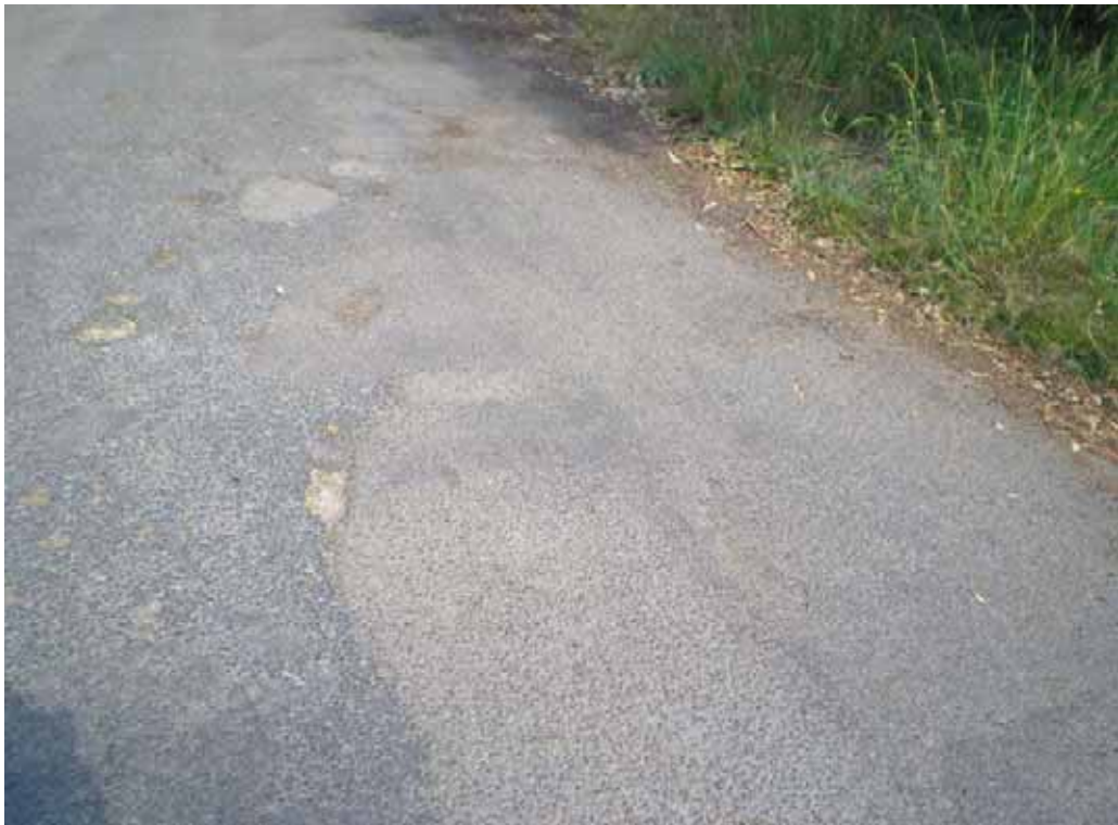
PHOTO 86: Settlement/rutting of repaired section at pavement edge, small potholes, loss of seal
