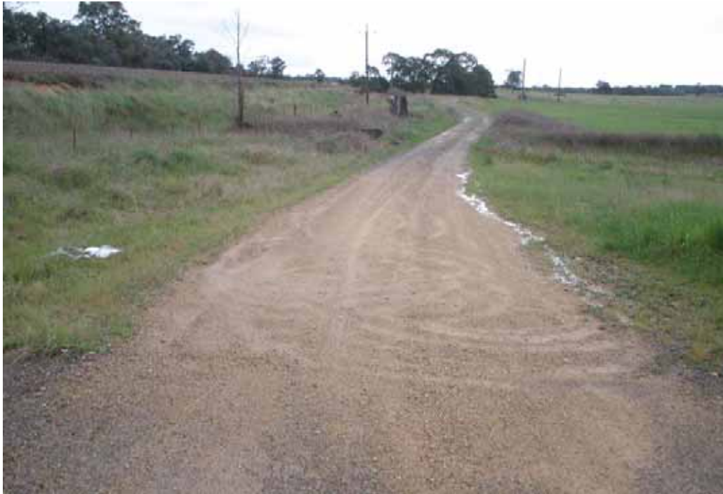
Photo 101 – Start of unsealed section Stoney Creek Rd. Uneven surface, slight erosion northern side.
