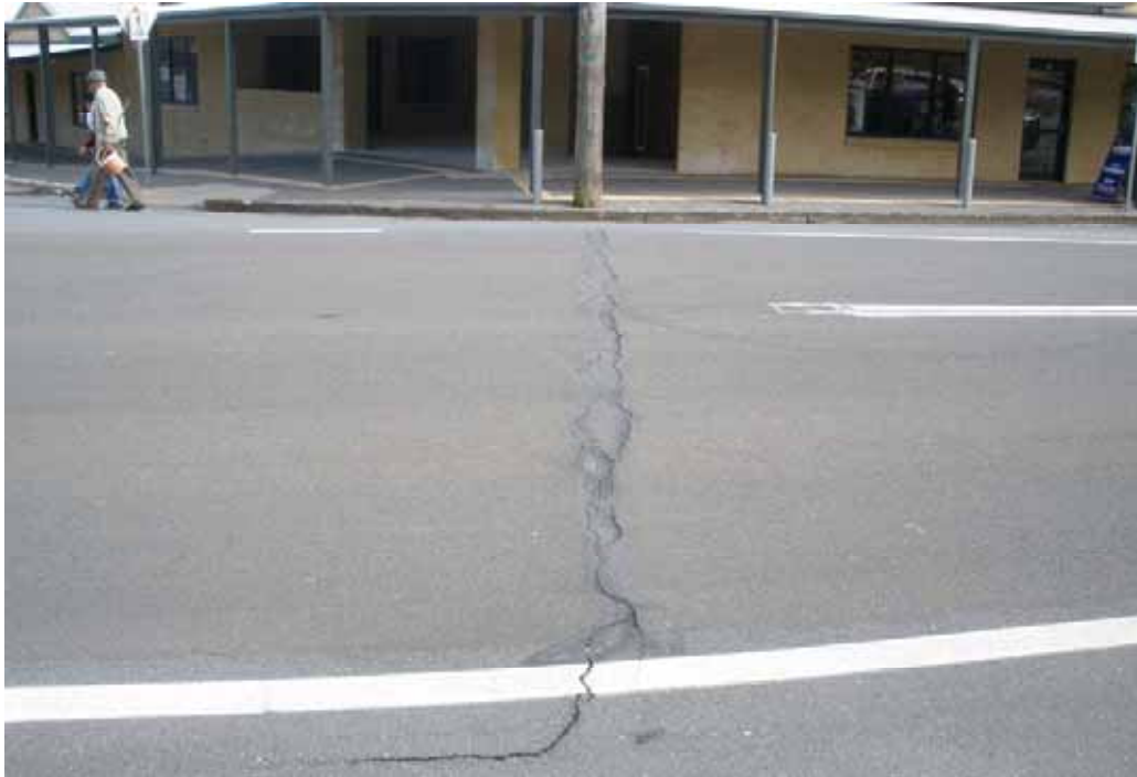
Photo 33 – George St/Goulburn St intersection. Pavement cracking post application of bitumen emulsion. Edges of cracking rising.
