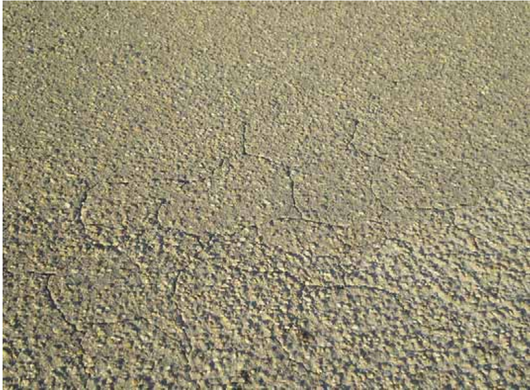
PHOTO 5: Start of cracking in asphalt
