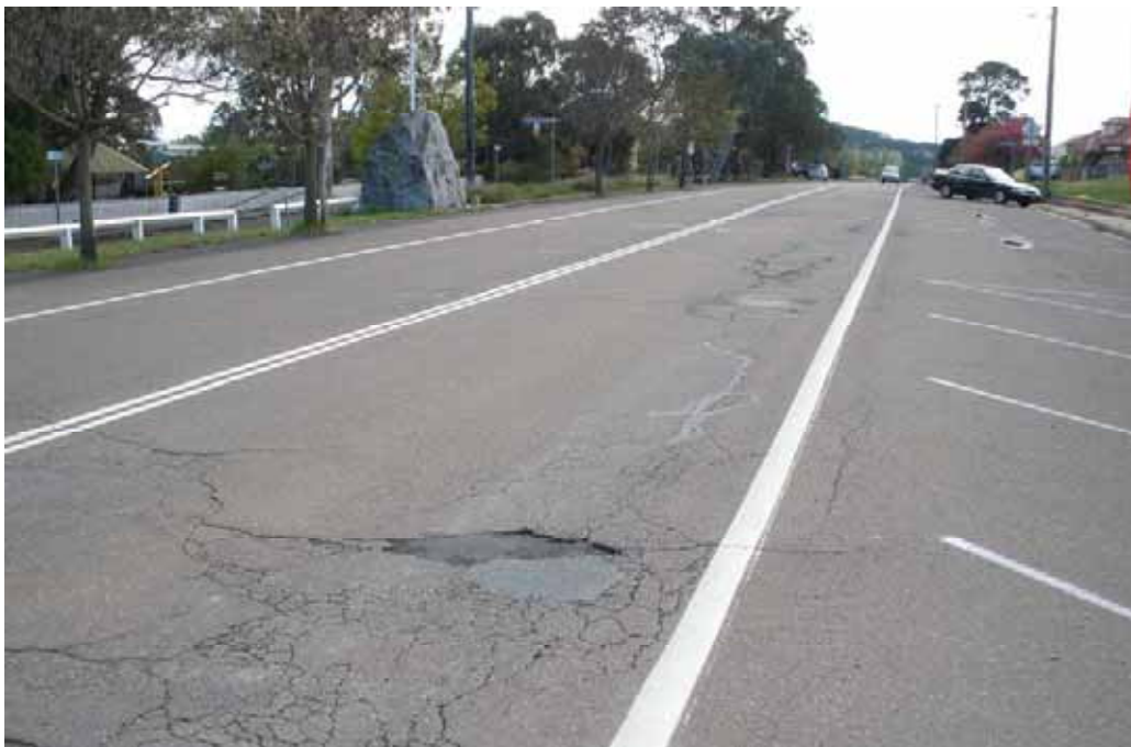
Photo 40 – Opposite post office. Extensive pavement failure some old patches.
