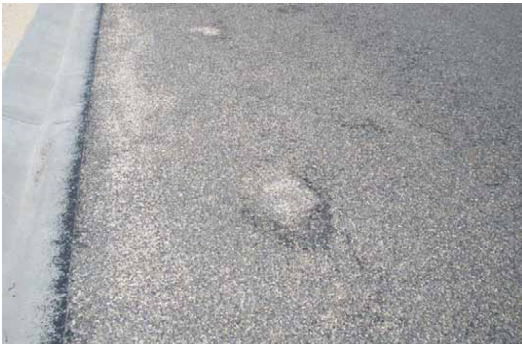
Photo 90 – Opposite No 29 Stoney Creek Rd. Small potholes.
