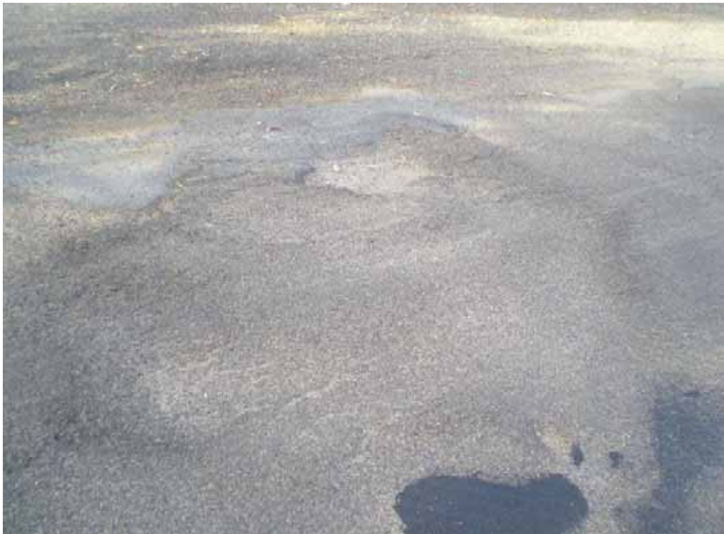
PHOTO 44: Failing repaired section
