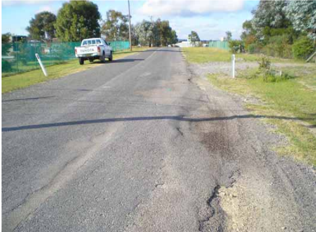
PHOTO 31: Cracking in asphalt, loss of seal, repaired shoulder, rutting at pavement edge
