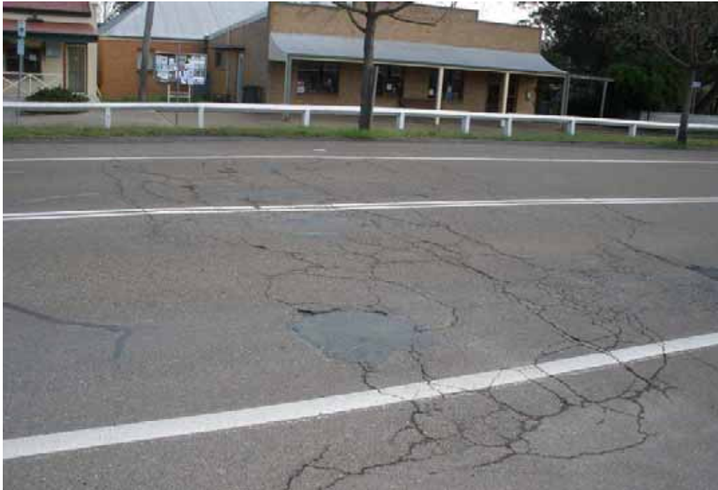
Photo 39 – Opposite post office. Extensive pavement failure some old patches.
