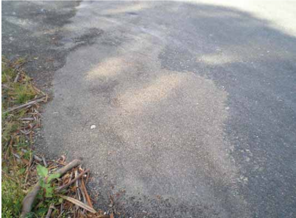
PHOTO 71: Repair to pavement edge, settlement
