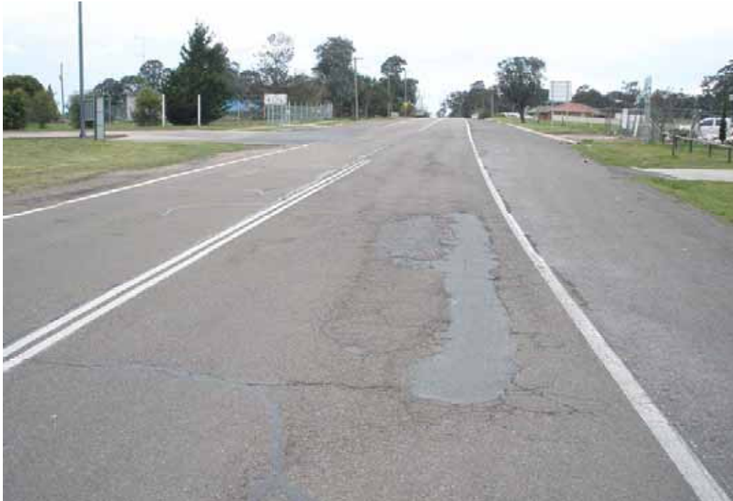
Photo 9 – In between entrance/exit driveways for Truck Stop. Extensive cracking, old patching and bitumen emulsion sealing of some old cracks.
