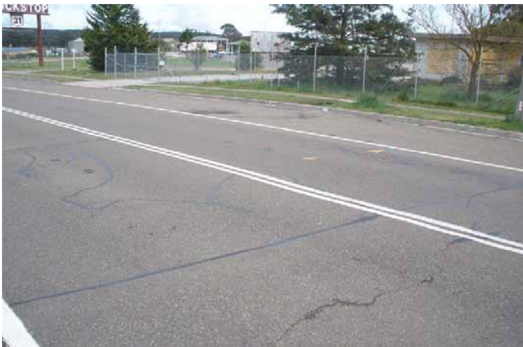
Photo 14 – George Street, opposite vacant blocks. Numerous cracking some sealed with bitumen emulsion.
