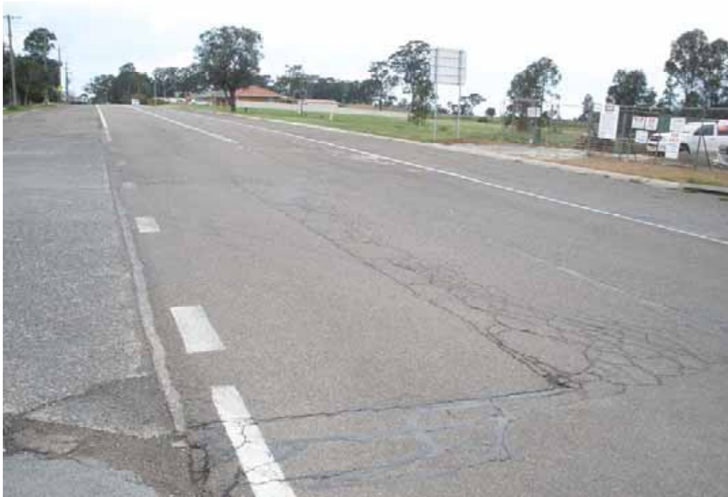
Photo 11 – Opposite exit driveway Truck Stop 31. Extensive cracking, old patching and bitumen emulsion sealing of some old cracks.
