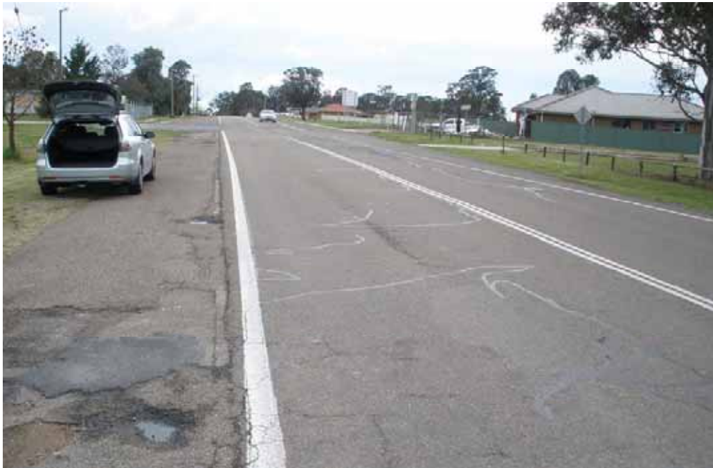
Photo 8 – In between entrance/exit driveways for Truck Stop. Shoulder failure, extensive cracking and bitumen emulsion sealing of some old cracks.
